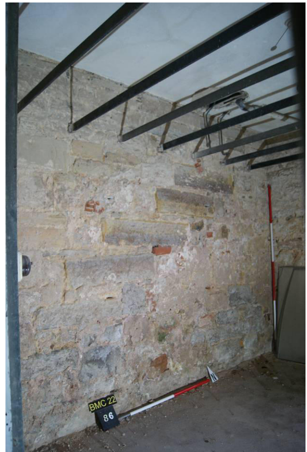
P53. R6 looking north-east with site of proposed lift against the north wall where truncated stone stair treads are visible. The iron game-larder racks are c.1892 or later
