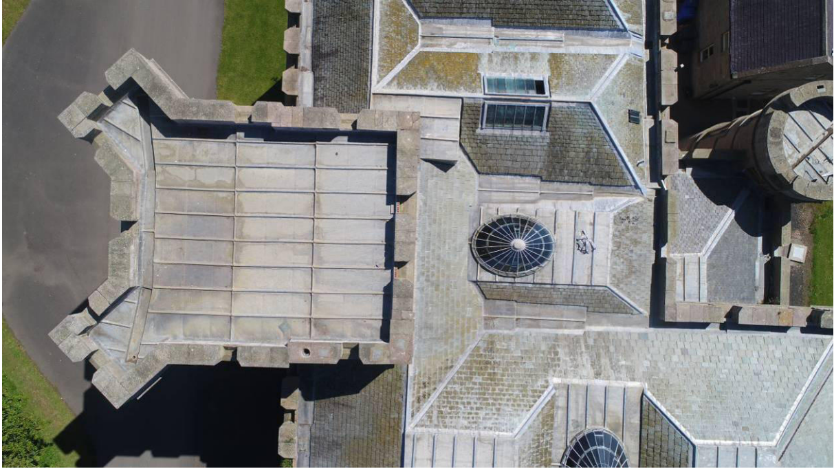
P35. Drone view of the Gatehouse and south wing roof showing 1980s lead and slate pitches. The cupola over the Great Stair is at the centre, and that above the Oval Saloon is just visible at the bottom of the picture.
