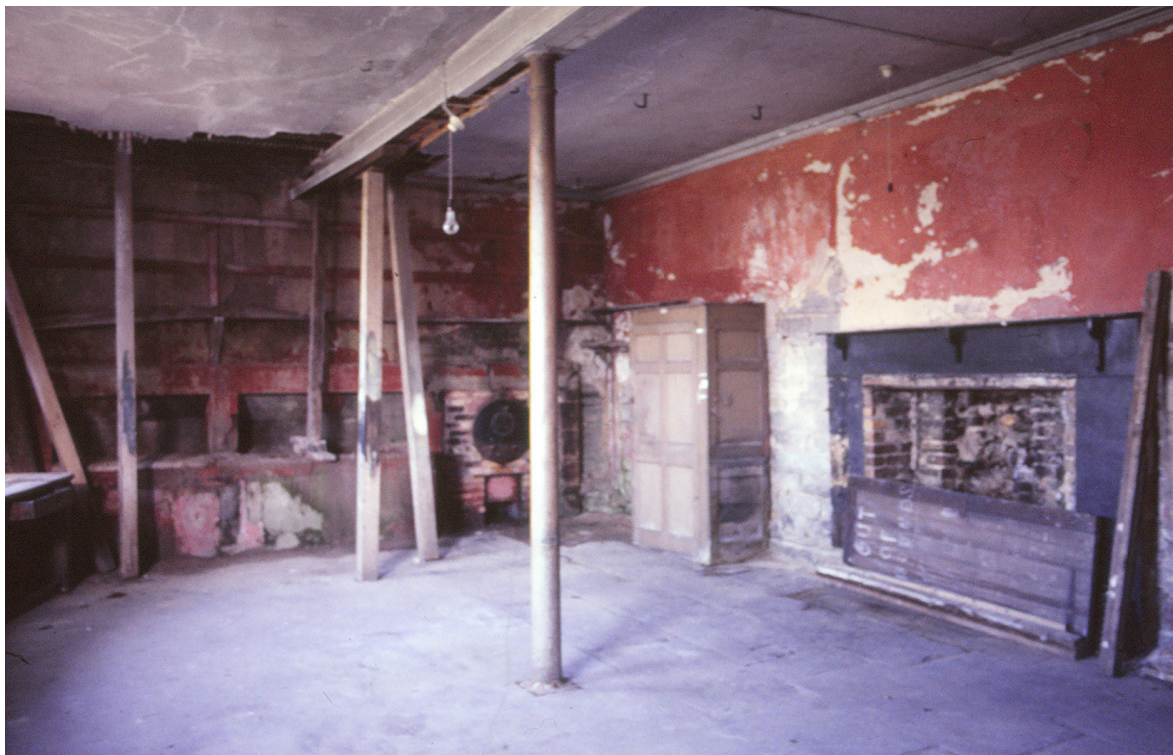
Fig. 48. R14 (kitchen) c.1984 looking north to the stewing range and oven [48-9], fire [50] right, and cast-iron column [70] centre.(J.Penn)
