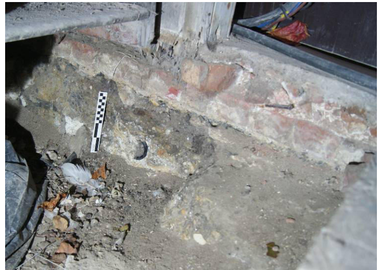
P45. R2 west end, showing deposits including a ?brick floor and a bottle-base, exposed in a partly backfilled 1980s service trench running from below the dumb waiter [78] to the west wall.
