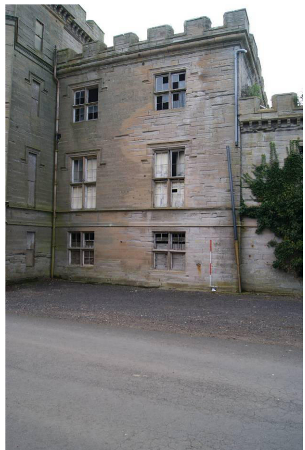
P5. East facade from the north, showing the late 16th-early 17 th century range refaced in 1801-4 and butted by Paterson's North Range (right).
