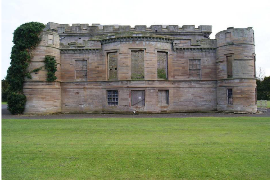
P19. North Range, north facade, showing barred ground floor windows [18-20] large former sashes at first floor level in the bay front [136-140], with 'blind' windows [133] and [141] either side. It is proposed to form a new 'house' within the North Range, and to convert central ground floor window [19] into a doorway.
