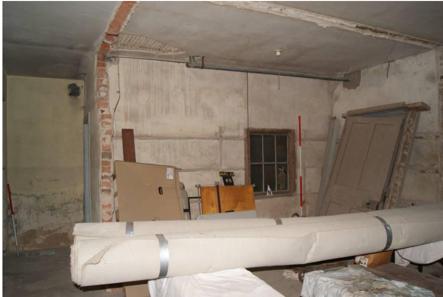
P51. R5 looking north to a brick partition wall with glazed panel [85] enclosing R6, this is proposed to be removed, and the space
