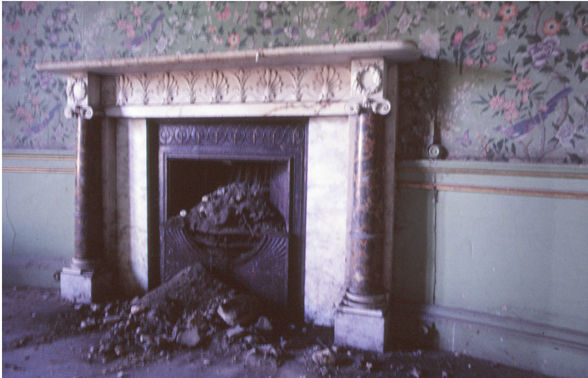
Fig. 53. R36 fire [175] c.1986 before stripping-out for dry rot remediation, showing dado rail and wallpaper. (J.Penn).
