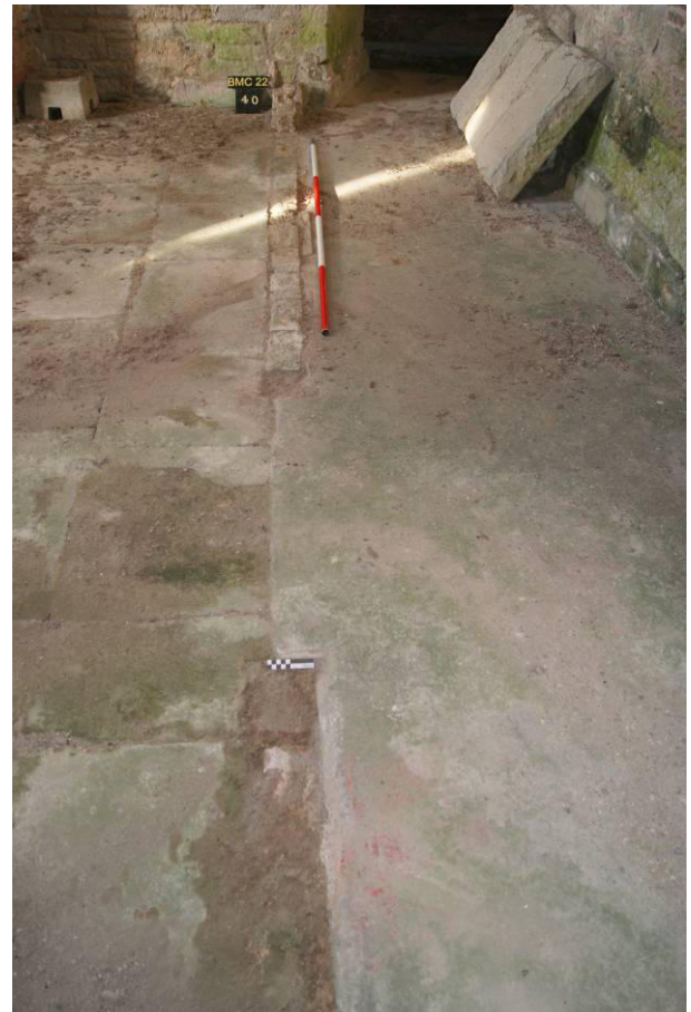
P58. R8 looking north. Showing the line of the lost partition wall between the scullery (left) and cement-floored
