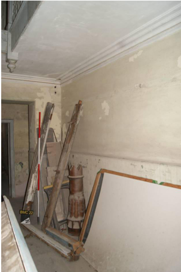
P47. R2. Looking east to the site of a proposed new door in the south wall, showing the matchboard lining to dado level.
