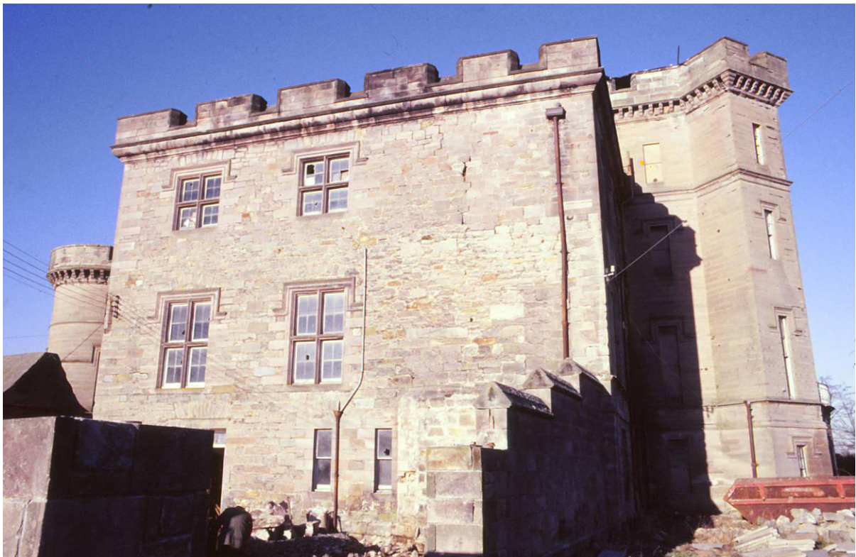
Fig. 38. The south-east angle of the Castle c.1986 with work underway, showing the stepped coped wall, part of the courtyard wall, and windows [37-8] (ground), [162-3] (first) and [225-6] (second). (J.Penn).
