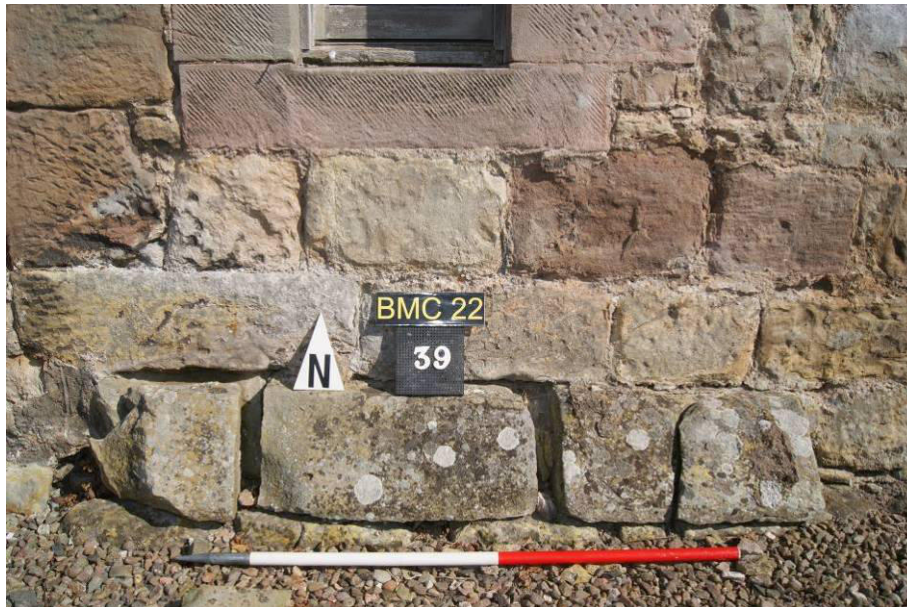
P32. South Wing south facade. Detail of the medieval chamfered plinth [39] and surviving facing stones below later window [38].
