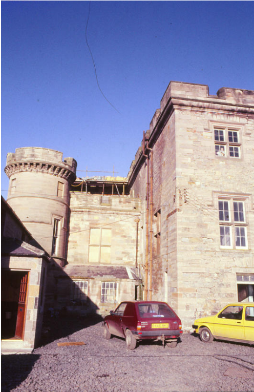
Fig. 43. The south-west facade c.1986 during roof works, showing the pump house between the South Wing and the south-west turret. (J. Penn)
