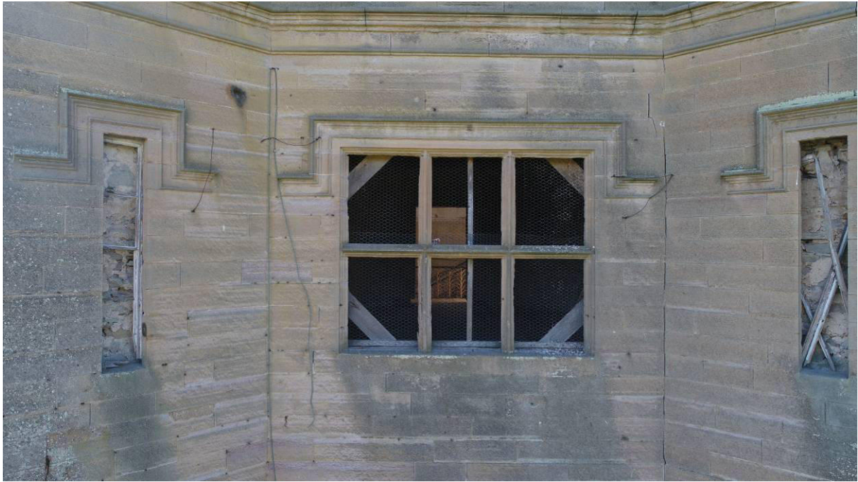
P15. East facade. The Gatehouse at second floor level, showing window [205] to R57, with 'blind' windows [204] and [206] to the corner turrets. Though blocked internally both of these have the remains of 'cosmetic' sashes. There is cracking in the masonry in the angle to the right of [205].
