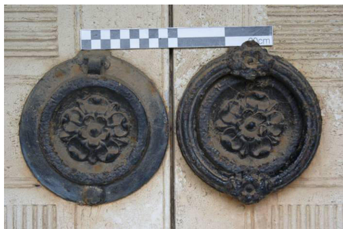
P11. Iron knockers, probably secondary, on the double doors to [7]. The left hand knocker has lost its ring.
