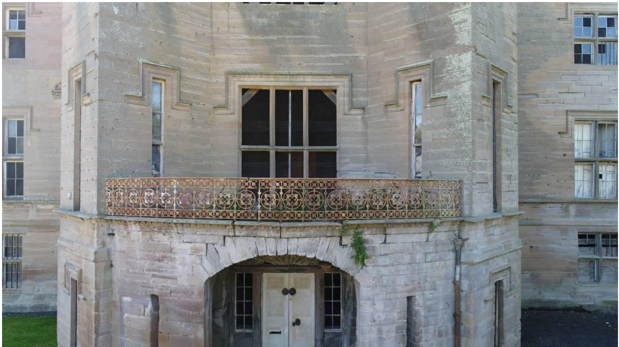
P6. The balcony at first floor level, with its cast-iron railing and window [169] to R36 behind. There are signs of structural movement in the arch of the porch below.
