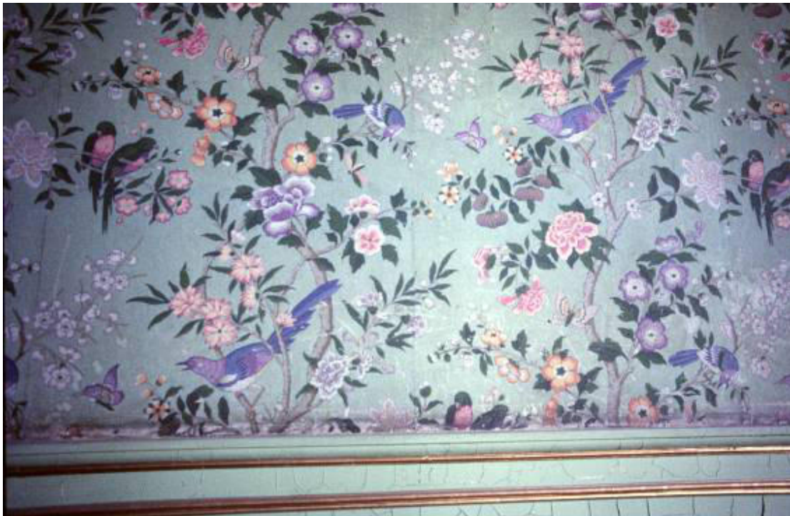
Fig. 54. R36, detail of the wallpaper and dado rail. (J.Penn).
