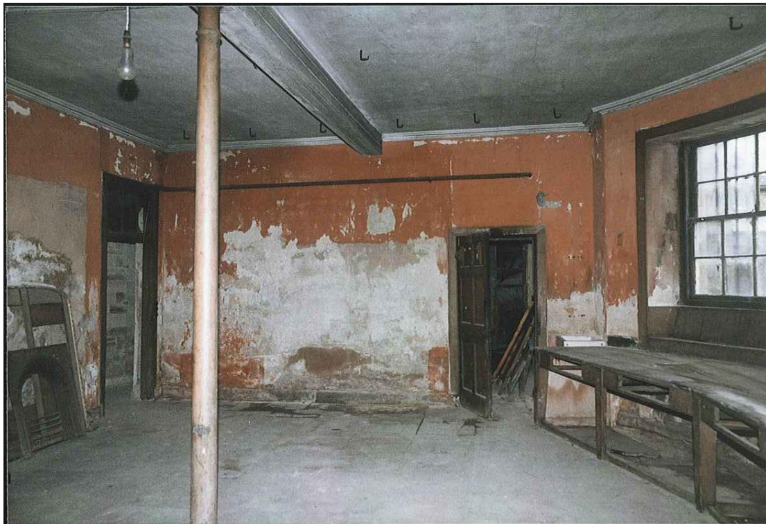
Fig. 50. R13 (kitchen) c.1984 looking south to door [43] on the right, door [52] and fire [50] left, and cast-iron column [70].(J.Penn).
