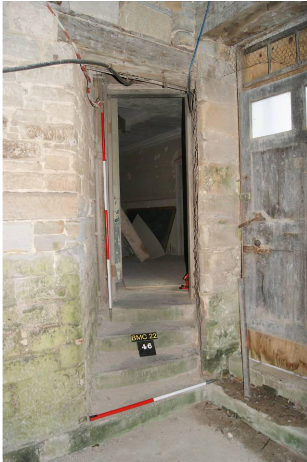
P57. R8 looking through [46] to the wall-passage to R2. This is proposed to be partitioned midway to form storage spaces.
