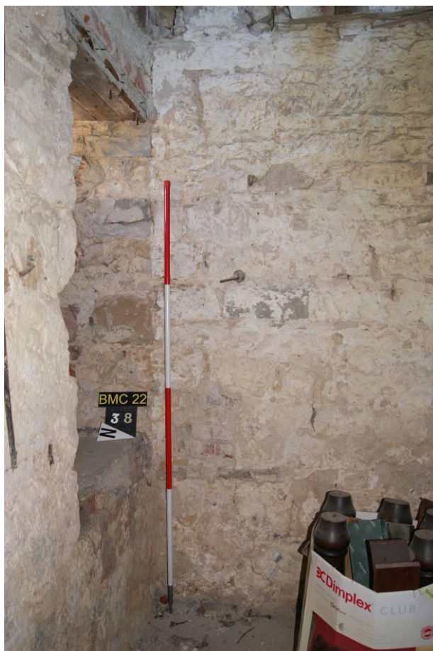
P50. R5. Looking west to the junction of the west and south walls at window [38]. There appears to be a butt joint between the two.
