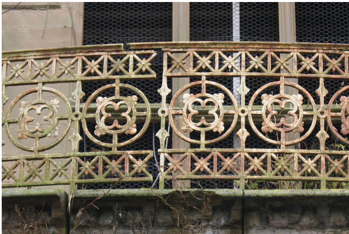
P7. Detail of the cast-iron balcony railing set into a moulded cornice, showing fracture due to structural movement.
