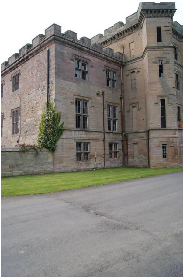
P4. East facade from the south showing the red sandstone masonry of the c.1892 addition, the Sitwell crest plaque below, and 'blind' windows in the Gatehouse.
