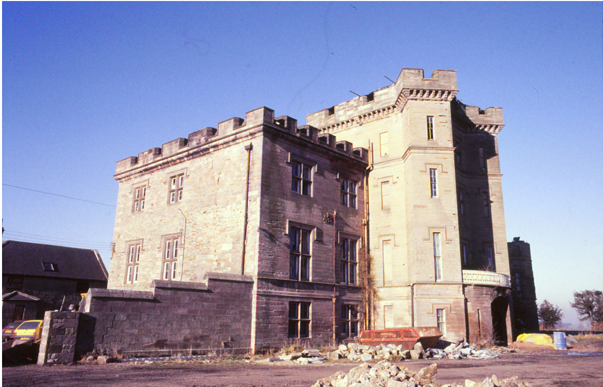
Fig. 39. The south-east angle of the South Wing with the Gatehouse, c.1986 with work on the roof underway. (J.Penn)
