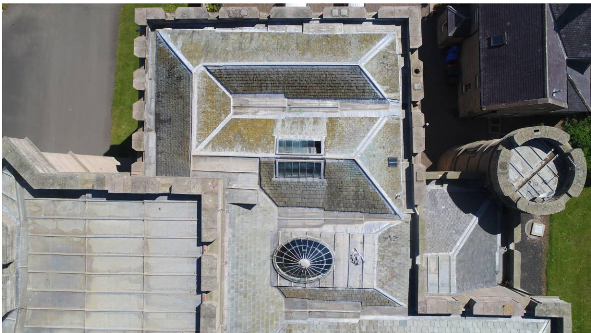
P36. Drone view of the South Wing roof and parapet of c.1892. The north-south slated roof is above R73. The south, The northern east-west slated roof is above R75, the southern with a rectangular skylight [315], is over the Service Stair R68, and has a hinged skylight [319] in the hip. The turret roof is above R40. The flat leaded roof at the south-west corner of the Gatehouse contains an access hatch [318]. The western parapet differs markedly in thickness from the West Range (lower right) and the c.1892 work. Capped and uncapped chimney outlets are
