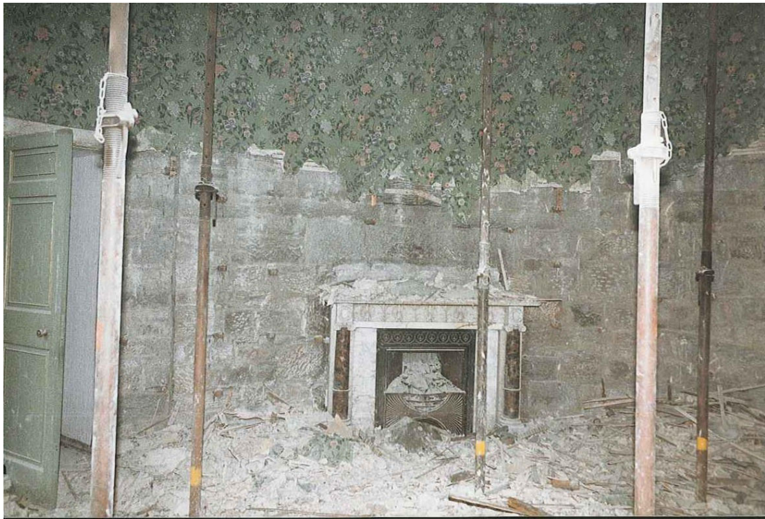
Fig. 55. R36, fire [175] c.1986 with removal of lath and plaster underway. Door [174] to R38 is on the left. Compare with P111. (J.Penn).
