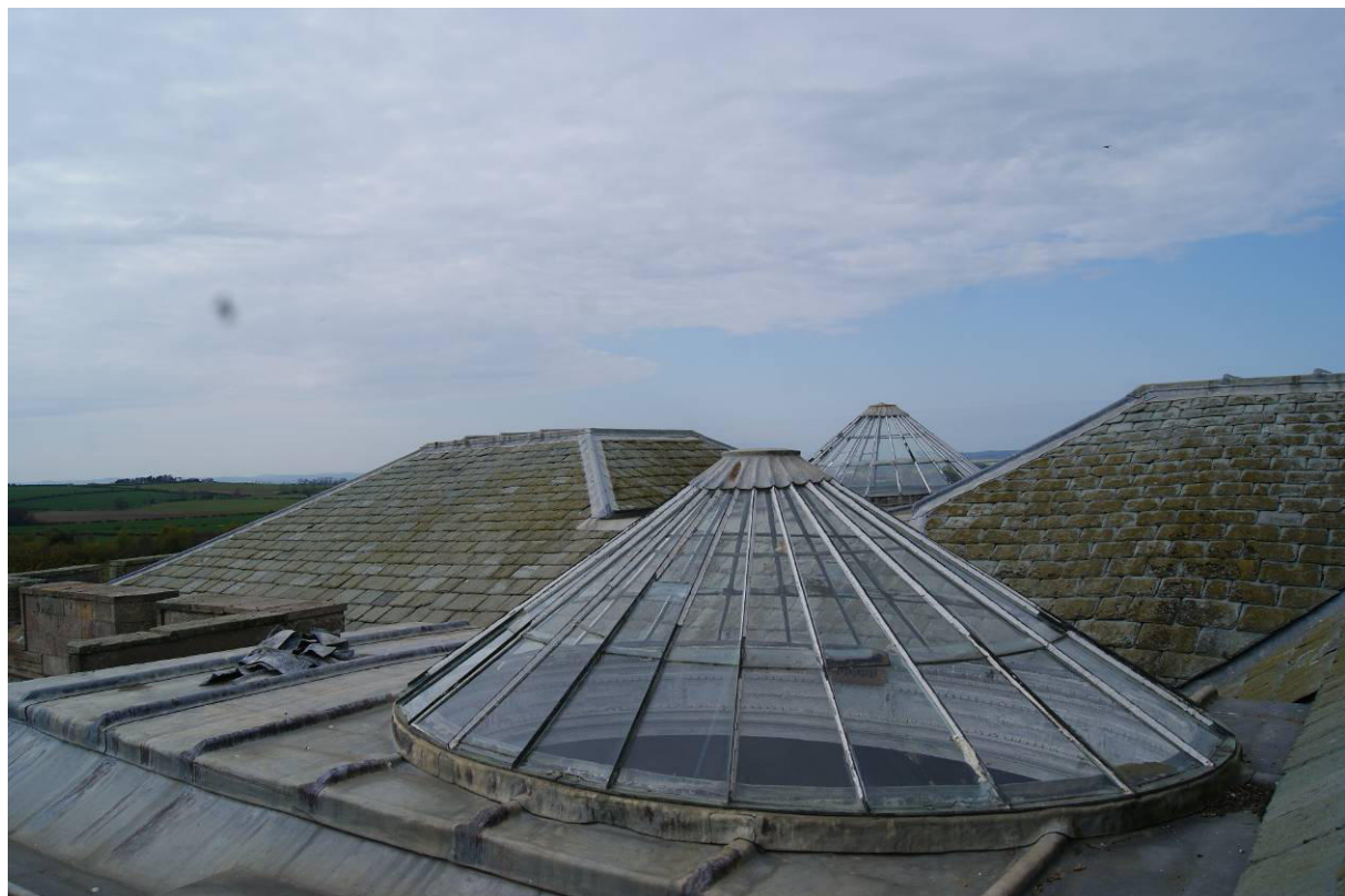
P38. Great Stair cupola [316] looking from the Service Stair roof-hatch [318] showing patch glazing repairs. The Oval Saloon cupola is in the background.
