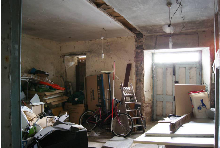
P44. R1 as it was in 2012, looking south-east. Showing scar of former brick partition.
