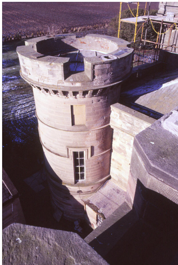
Fig. 44 . Looking down from the South Wing parapet c.1986 with the roof of the pump house abutting the south-west turret.(J. Penn)
