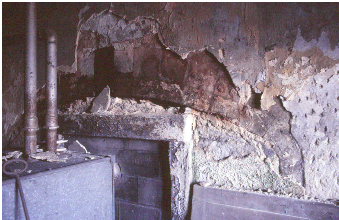
Fig. 52. R19 c.1986 with the arch of fire [63] just visible under later plaster and blocking for a solid-fuel boiler.(J.Penn).
