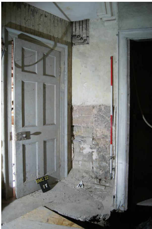
P46. R2, west end. Areas of the north wall stripped of plaster, showing a vertical joint between ashlar (left) and rubble masonry. A set of bell-cranks [109] is exposed above.
