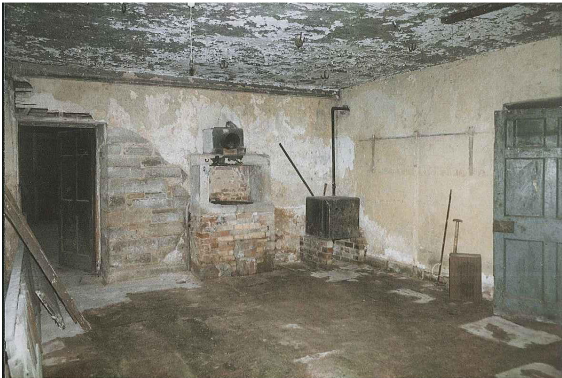
Fig. 47. R8 (scullery) c.1984 looking north-east to the copper [41] with door [43] to the kitchen on the left, and the demolished partition to passage R8.1 right. (J.Penn)
