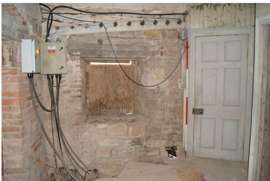
P48. R2. Looking west to window [33] with a line of servant's bells above and boarded-over 1980s excavation for electrical services below. Door [77] is on the right.
