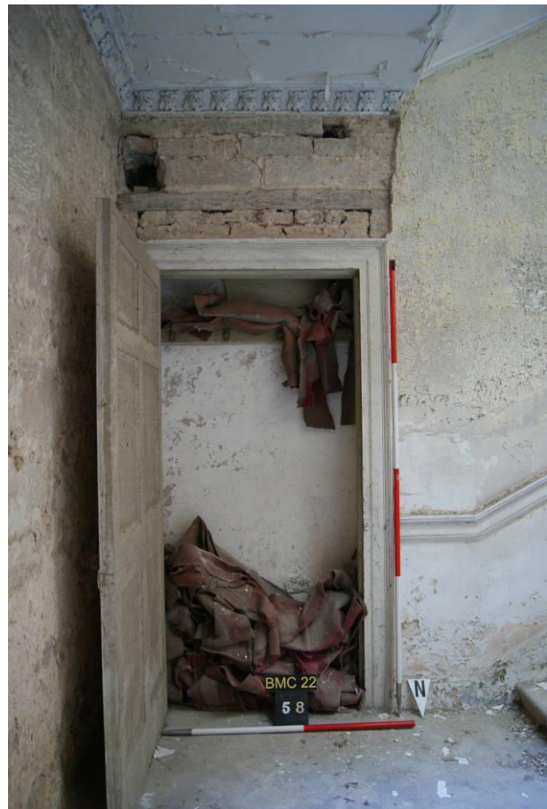
P61. R9, doorway to wall-closet [58] proposed to be opened as a doorway to the reconfigured areas of R5 and R6. This will involve removal of the rear of the closet.
