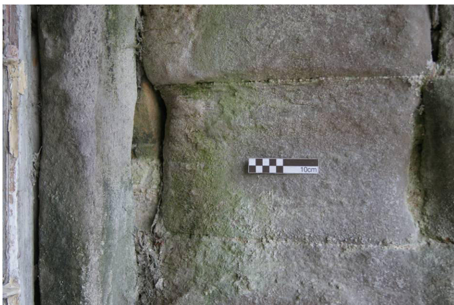
P14. East facade, north side of the porch showing its junction with screen wall [7], which extends behind the porch masonry.
