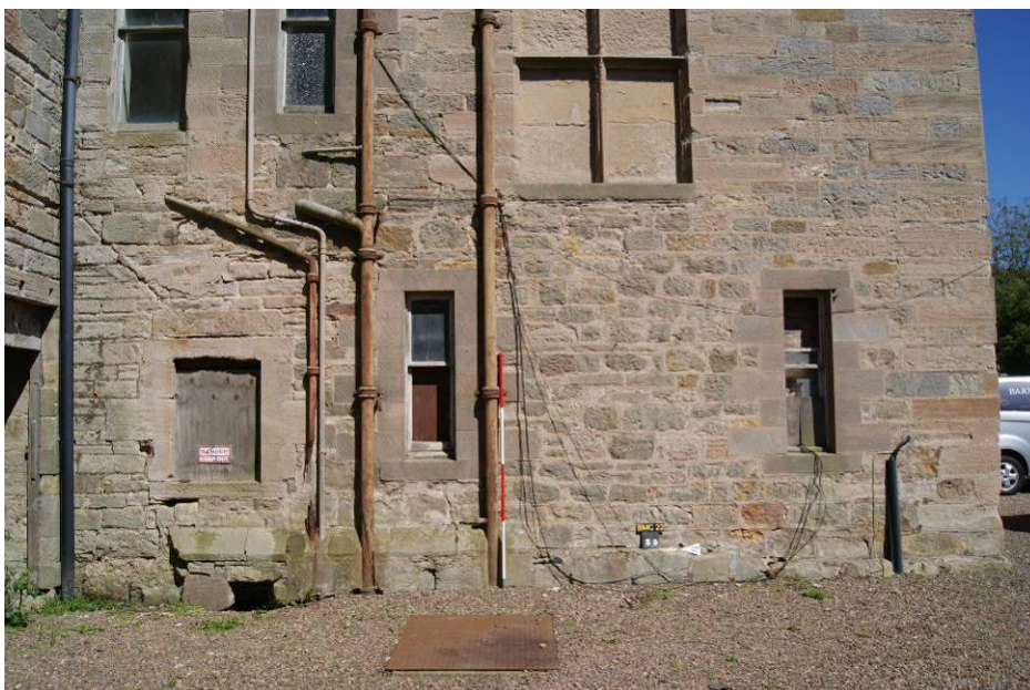
P25. South Wing, south-west facade, showing the remains of the medieval tower's chamfered plinth [39], c.1892 ground floor windows [33] – [35] and first floor windows [159], [160], and 1801-4 'blind' window [161].
