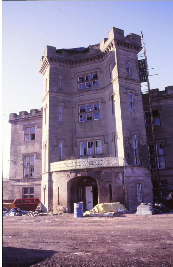
Fig. 41. Work on the Gatehouse underway c.1986. The timber-frame windows [169], [205] and [305] are still in position. (J.Penn)
