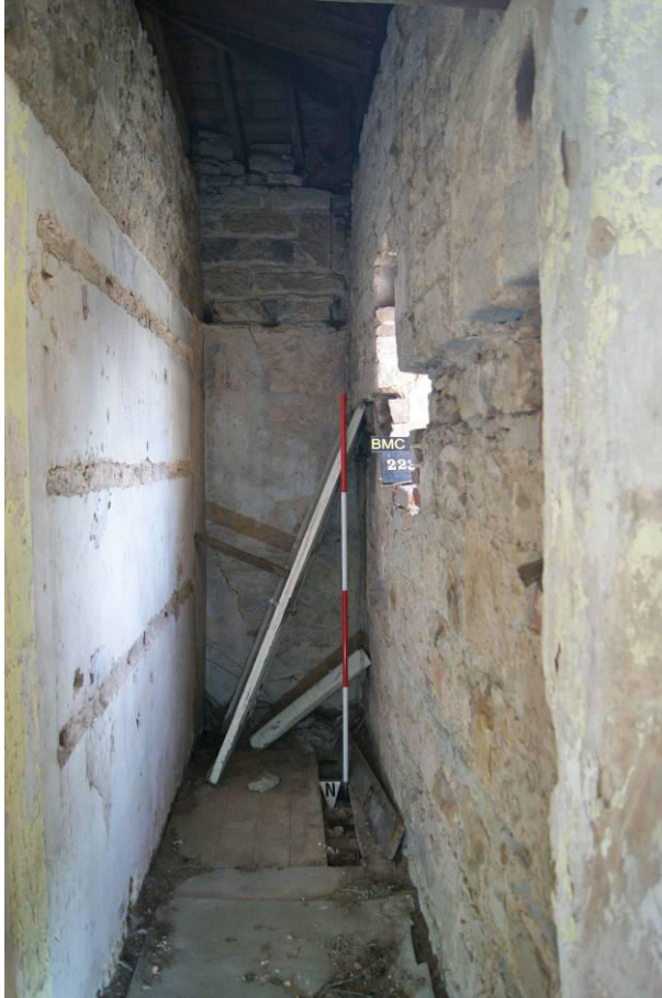
P159 R63. Looking south. Showing floorboarded end section and offset upper part of the west wall with window [223]. The offset wall may be as late as c.1892. The room may have been intended to carry another service stair but appears on the 1801 plan as a 'Water Closet'. In the current
