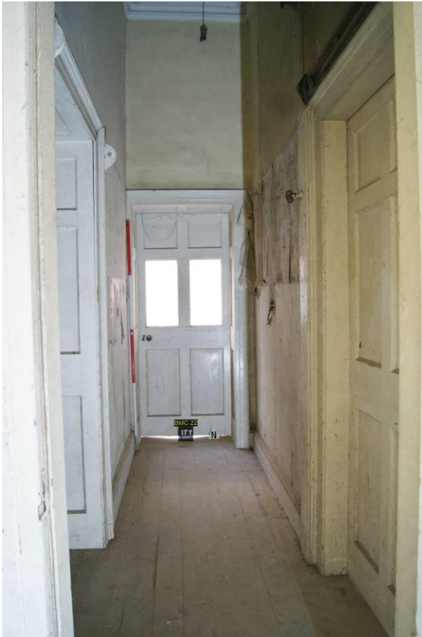
P103. R28 looking north to door [177] (1801-4). The stud wall (right) is proposed to be removed to accommodate a lift, and a new door inserted dividing the passage.
