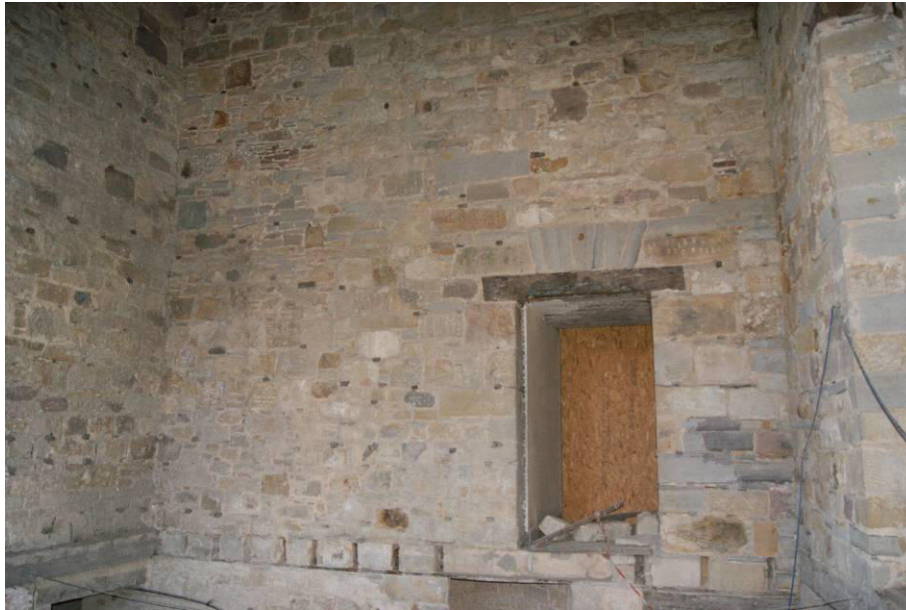
P115. R39 looking east to door [158] with sockets for removed floor joists below. The rubble masonry, stripped of lath and plaster, suggests either the survival of some earlier fabric, or reused material. New partitions are proposed along this wall-
