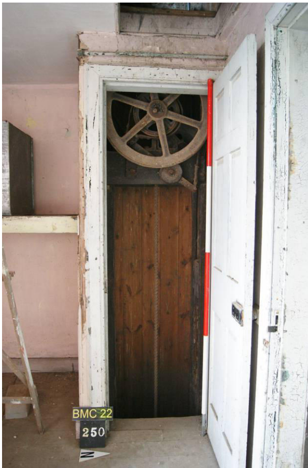
P146. R55. Head of the dumb waiter shaft with wheel and tackle. It is proposed to remove the door and enclose the shaft, with a 'viewing window' in the west wall of R52.
