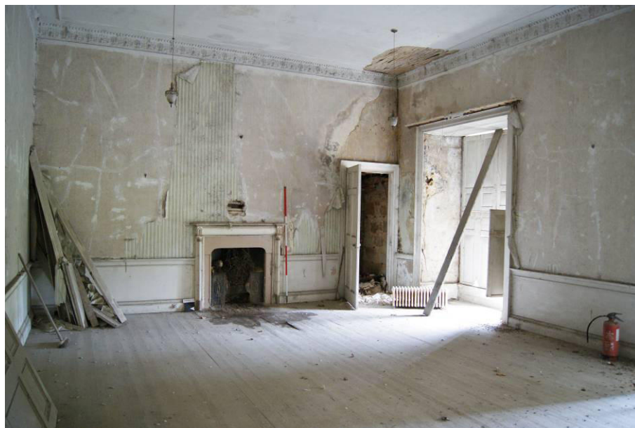
P128. R42. The same room view in 2012 for comparison. Closet door [126] is open and plaster in the reveal of window [125] is intact.
