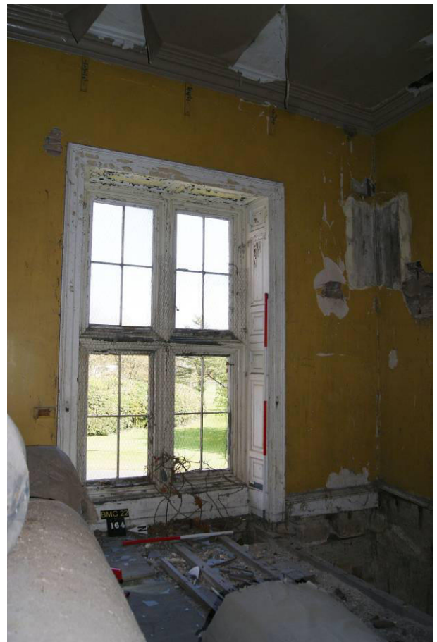
P104. R29 looking south-east with invasive creeper coming through window [164]. The southern part of the floor has been removed. This room is proposed to be reconfigured with a new partition.
