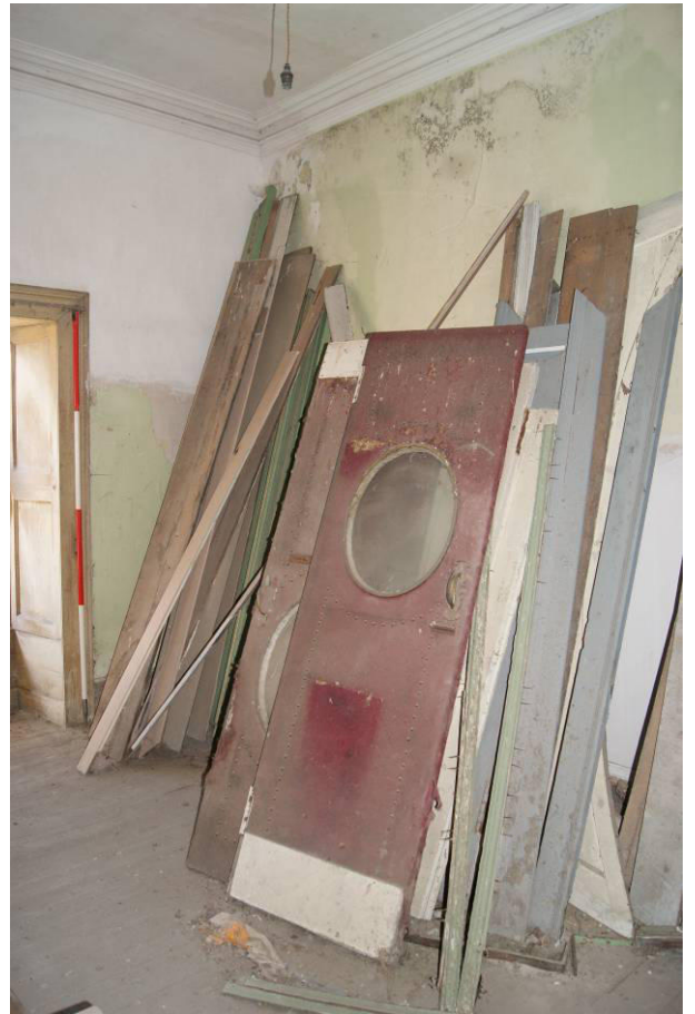
P138. R49. Showing some of the detached fittings including a pair of red baize-covered door leaves with oval windows and brass fittings (original location unknown).
