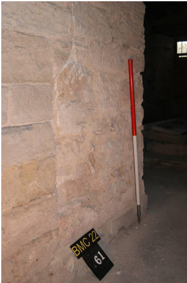
P75. R18, east end. 1801-4 masonry (left) butting the west wall of the late 16 th /early 17 th century range. The junction is the site of a proposed blocking wall.
