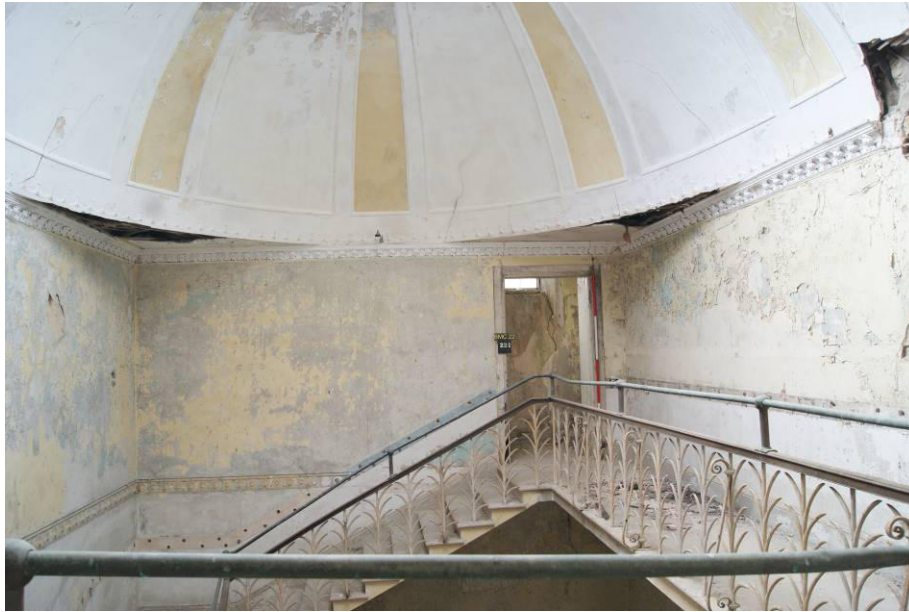
P151. R56 looking west, showing areas of lost decorative plasterwork on the spandrels of the cupola, and door [221].
