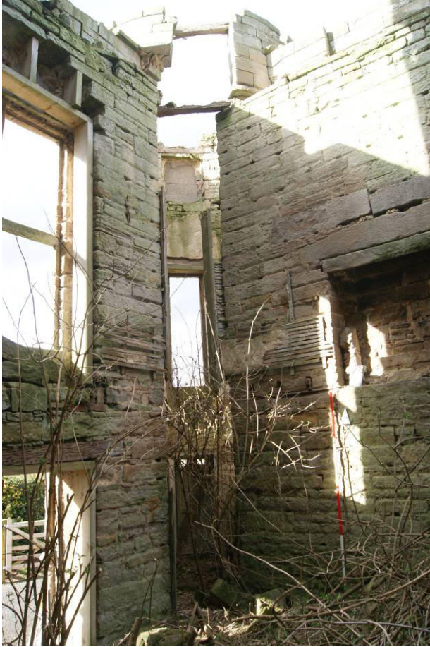
P94. R24. Looking north-west to turret rooms R25/48 showing unstable masonry at parapet level.
