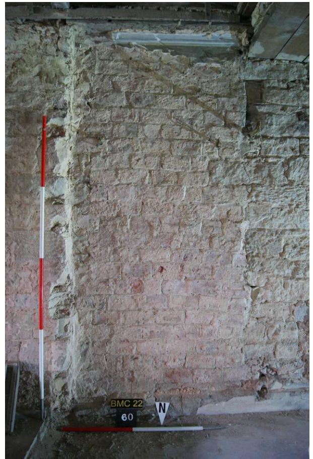
P76. R19, north wall showing on-edge brick infill of a pre-1801-4 doorway [60] which is proposed to be re-opened.
