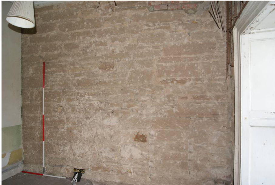
P145. R54. North wall stripped of lath and plaster. The western (left) side is the proposed site of a lift from ground floor level. There are traces of infilled holes forming a diagonal line, rising to the east, which may represent a former timber stair.
