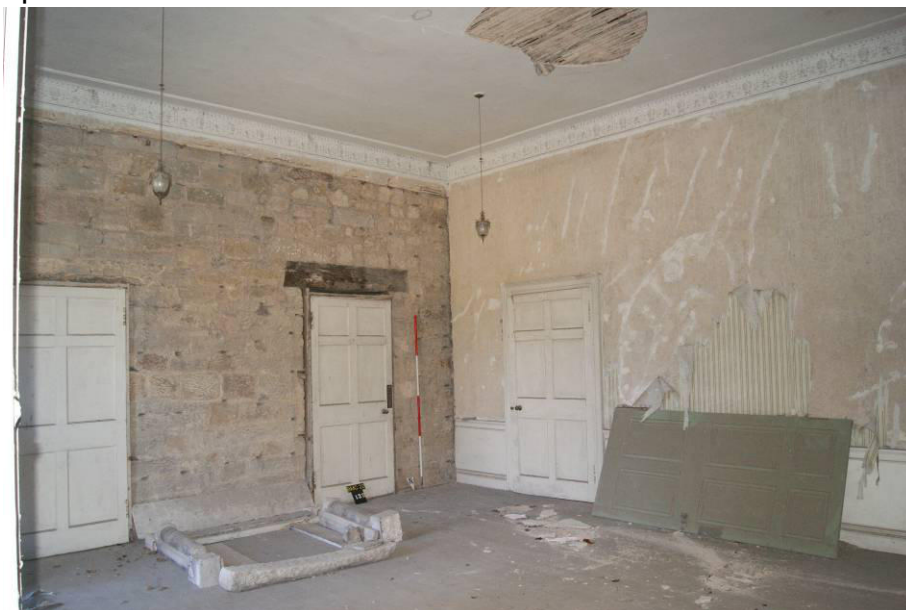
P130. R42 looking south-west showing area of fallen ceiling plaster. All three doors [121-3] are proposed to be retained. The fireplace surround lying on the floor belongs to fire [175]
