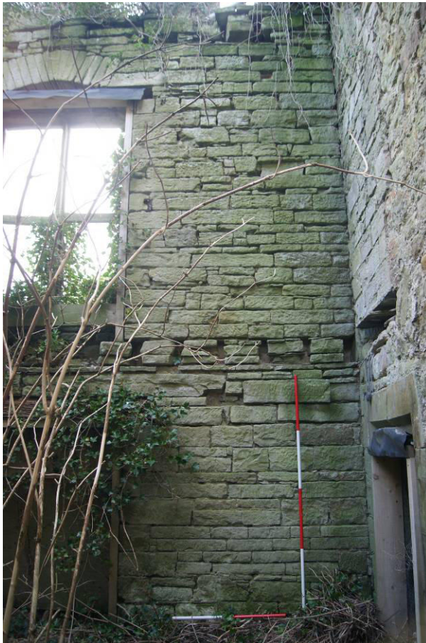
P85. R22. Looking to the junction of the late 16 th -early 17 th century north range (right) and the 1801-4 North Range, showing the butt joint.
