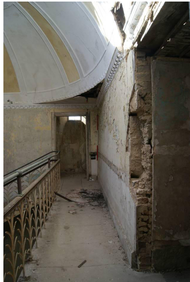
P153. R56. Looking west along the landing with door [235] on the right. Fallen plaster and rotted laths from the north-west spandrel are lying on the landing slabs.
