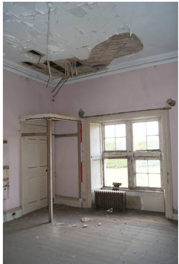
P142. R51 looking north-east. Door [254] in the north-east corner, currently sealed, is proposed to be reopened and a new partition inserted across the room.
