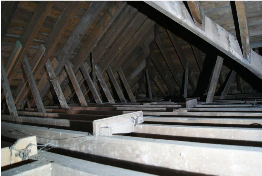
P179. Attic space R73 above R51 and R54. Looking south with a series of cast brass service bell-cranks mounted on sections of floorboard. This also shows roof repairs with bracing pieces to rafters, most of which have bolted-on replacement ends. This is all part of the c.1892 raising of the south wing.
