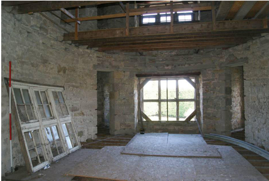
P154. R57. Room view looking east to window [205]. The modern replaced floor joists are partly decked with chipboard panels. Lintels above the doors have been replaced in cast concrete. The complete internal window frame with glazing rests against the north wall
