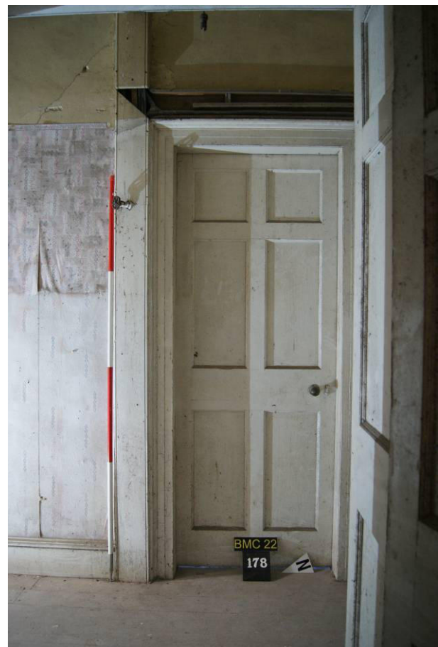
P102. R28 looking east from Service Stair door [182] to door [178]. Door and adjoining stud partitions are proposed to be removed
