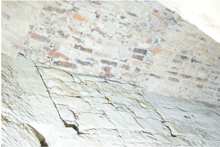
P95. R8.2 Blocked opening [185] at first floor level in the east side of the mural stair. A rough patch of brickwork in the vault appears to be associated. Possibly a pre-1801-4 feature.
