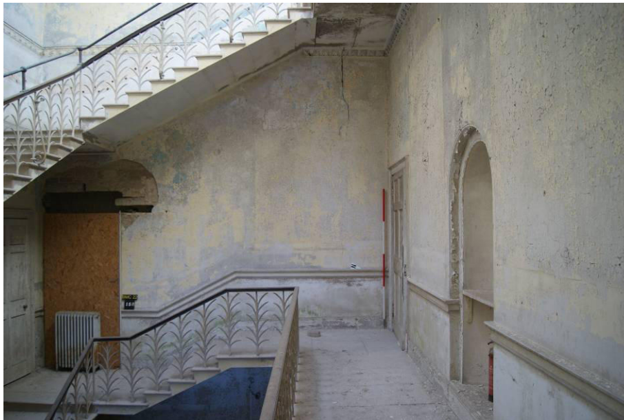
P109. R35, Great Stair first landing looking west, showing cracking in end wall plaster. Door [158] (left) with lintel missing and plaster damaged is proposed to be reinstated. Door [118] and alcove [120] are on the right.
