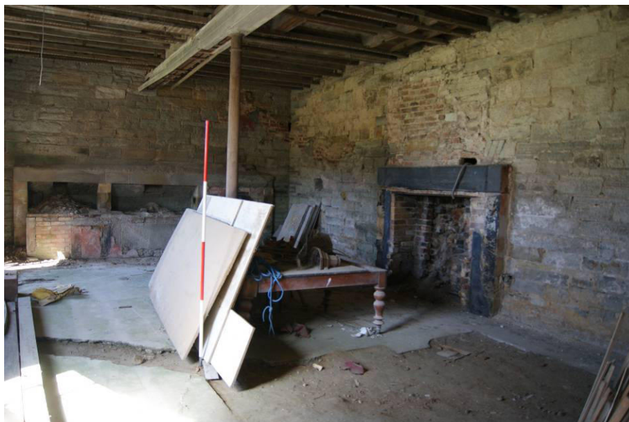
P65. R14. 'Kitchen' on the 1801 floor plan. General view looking north to the stewing range [48] and fire [50]. In the foreground the line of a backfilled 1980s service trench cuts across the cement screed flooring. Timber panels lean against the cast-iron column [70] supporting the floor above.
