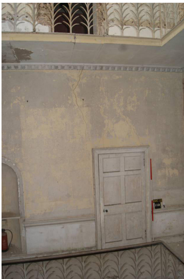
P110. R35, looking north from the second flight of the Great Stairs to door [119]. Note the displaced slab of the landing above.
