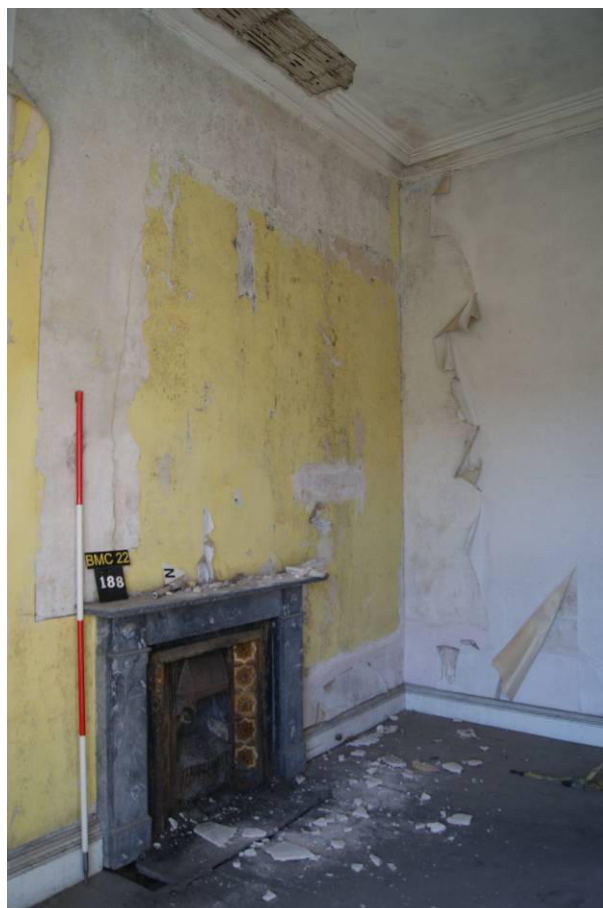
P99. R26, part of the c.1892 remodelling, looking north-west showing loss of ceiling above fire [188].
