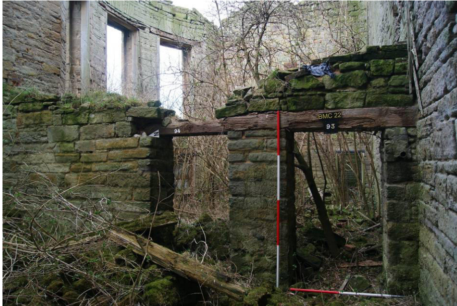
P92. R24. Looking east to the dividing wall with R22 and doors [93] and [94], which was reduced to first floor level in 2013.
