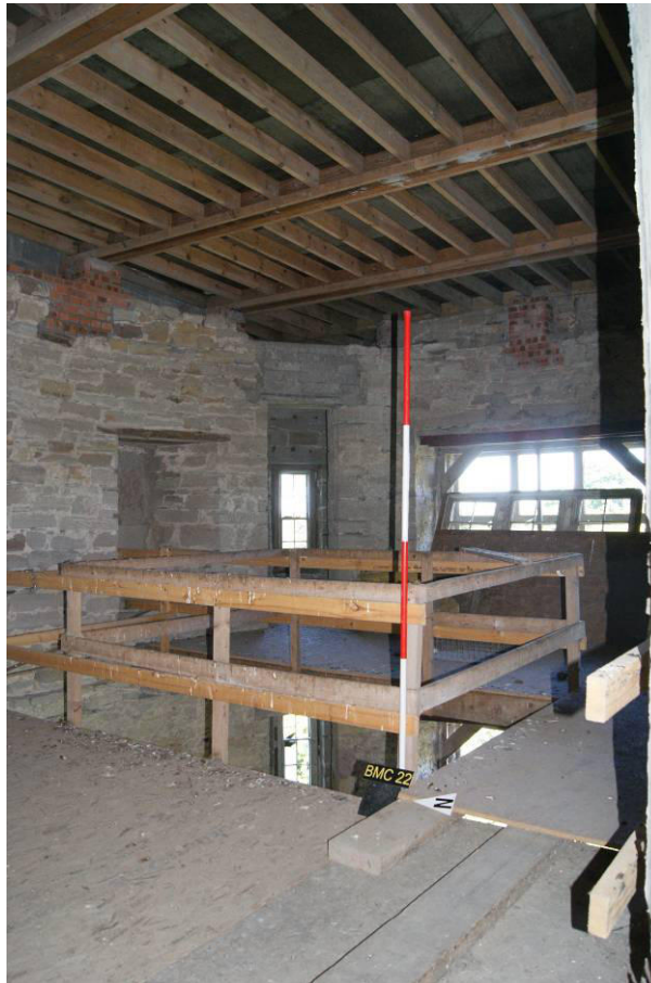
P167. Gatehouse, R69. General view looking north-east to window [305] and turret room R70. Little perceptible change has occurred since 2012. More chipboard decking panels have been laid and bird infestation continues.
