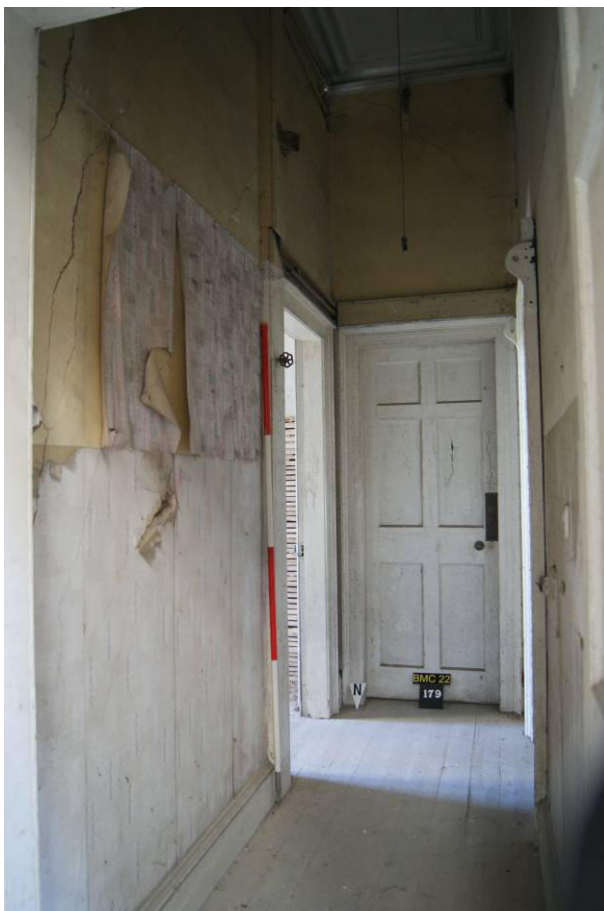
P101 R28 looking south to door [178] to R30 (left) and [179] to R29. The stud walls (c.1892), with 20 th century wallpaper, are proposed to be removed and the spaces reconfigured.
