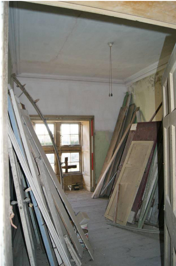
P137. R49 looking south. The position of a removed fire is shown by the grey plaster beside window [225].
