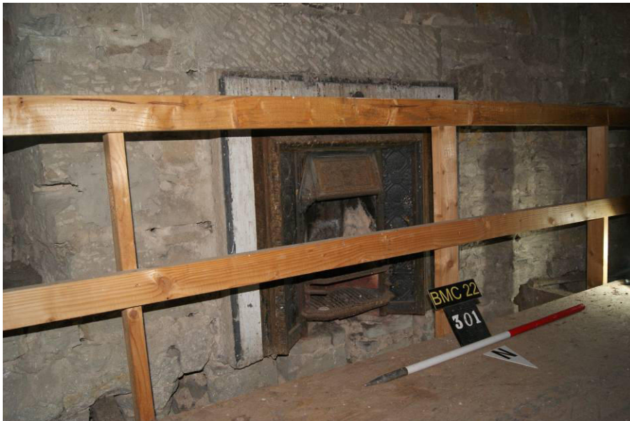
P168. Gatehouse, R69. Fire [310], with modern railing and chipboard decking. All walls have been stripped of lath and plaster. The fire has a late 19 th century grate. This room is proposed to become a bedroom, with the fire retained as a
