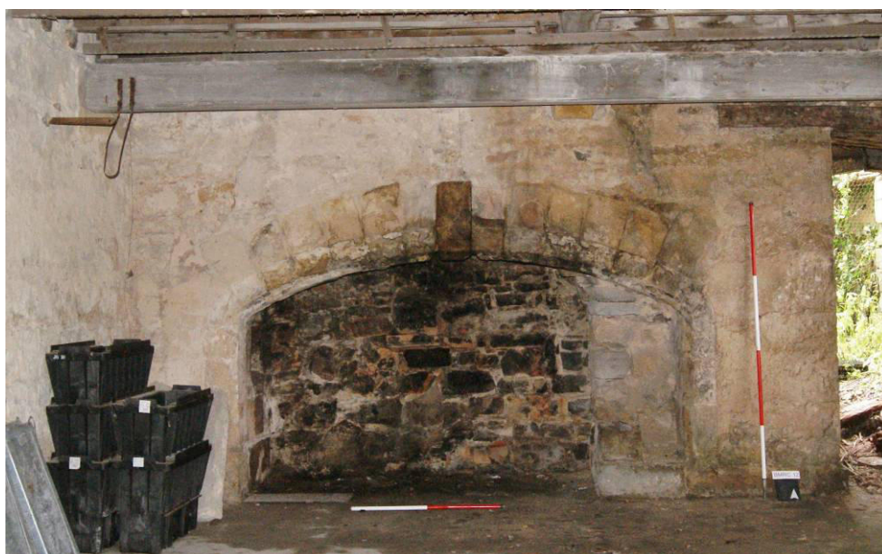
P82. R19. 'Servant's Hall'. The same fire [63] photographed in 2012 when the arch was intact.
