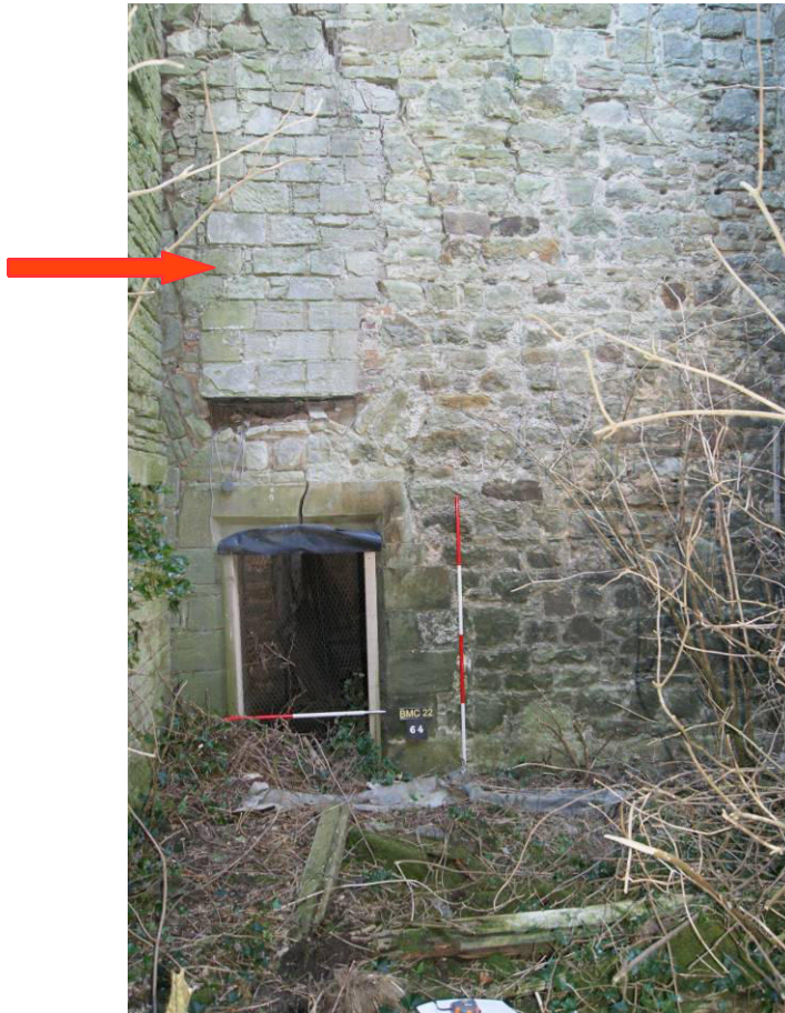
P129. North Range. R44. Doorway [128] (arrowed) from R42 inserted into the north wall of the late 16 th /early 17 th century range in 1801-4 and blocked in the 1950s. This doorway is proposed to be reopened to access a rooftop patio area above R20.
