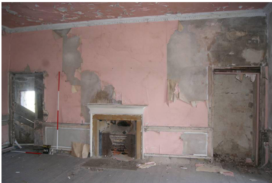
P158. R62 looking north showing wall closets [239] far right and [241] far left. Fire [24] has a stone surround, possibly 18 th century, behind a later timber surround. This will be retained in the proposed conversion.
