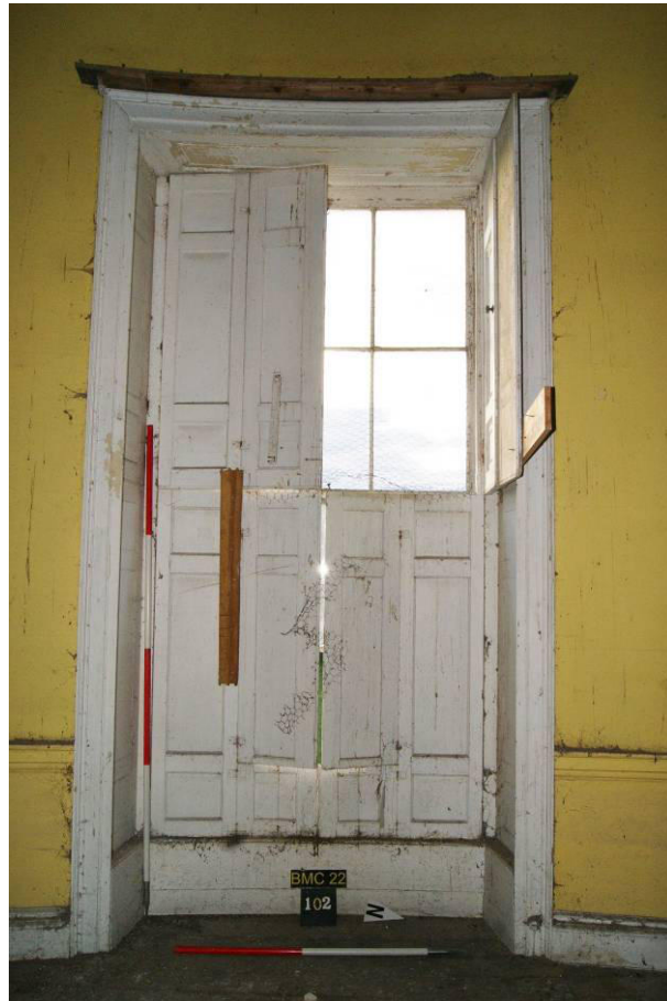
P136. R43. Window [103] with original shutters and sashes with some panes of thin early 19 th century glass surviving. The shutters, sashes, and fittings will be
