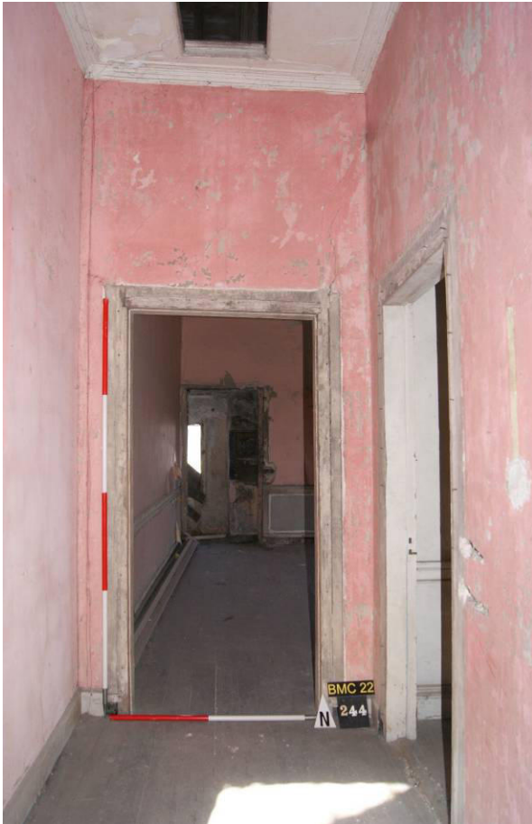
P156. R60 looking north. The door ahead [244] will be retained, but that on the right [237] will be blocked. Hatch [236] is visible in the ceiling.
