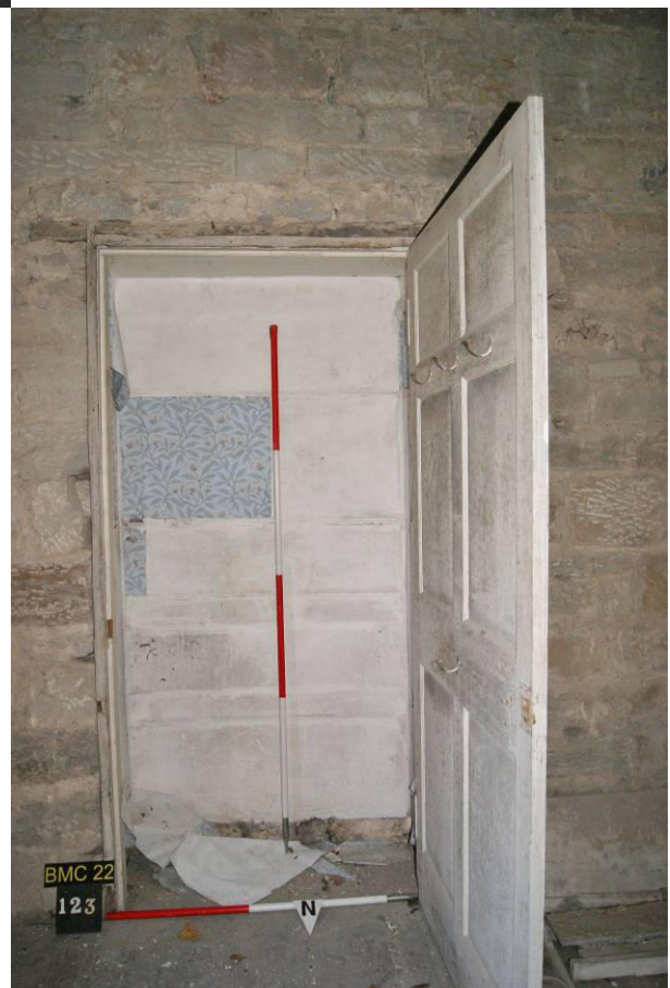
P132. R42. Door [123] to wall-closet R42.1. The rear of the closet is proposed to be broken through for an access to R36 in the Gatehouse. There is 19 th century grafitti on the plaster.
