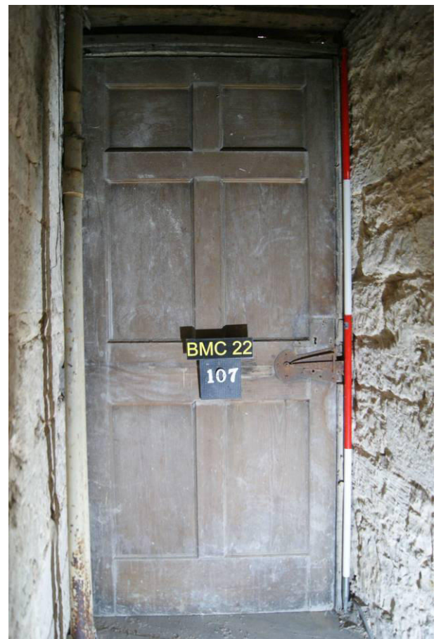
P97. R8.2 Service door [107] at the head of the mural stair, opening into the passage linking R42 and R41. The leaf has a spring catch (detail P98) and
