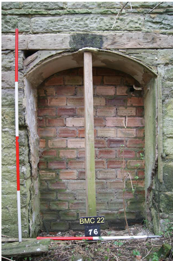
P89. R22. Door [74] to service passage R16 with 20 th century brick blocking, which is proposed to be removed and the passage blocked further south in the passage to create a W.C.
