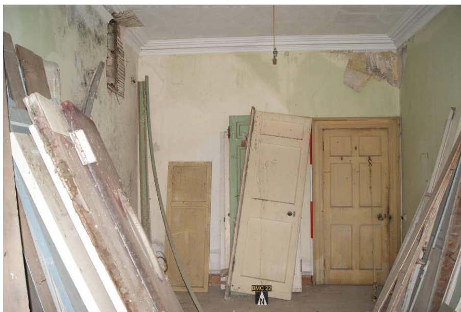
P139. R49 looking north. The existing door [246] is proposed to be removed and a new opening made further west, behind the stacked doors.
