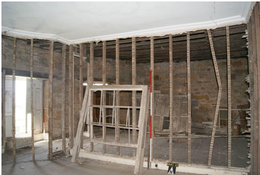
P160. R66 looking north-east to a stud partition stripped of lath and plaster. The framing looks recent but the partition corresponds broadly with that shown on the 1801 floor plan and the lath nails look hand-made. This suggests the partition belongs to the 1801-4 build. The frame of window [214] leans against it.
