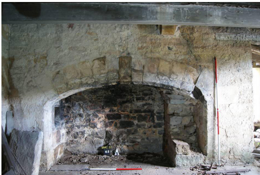
P81. R19 'Servants Hall' looking north to fire [63], showing loss of part of a right-hand voussoir of the arch and evidence of instability in the centre of the arch.
