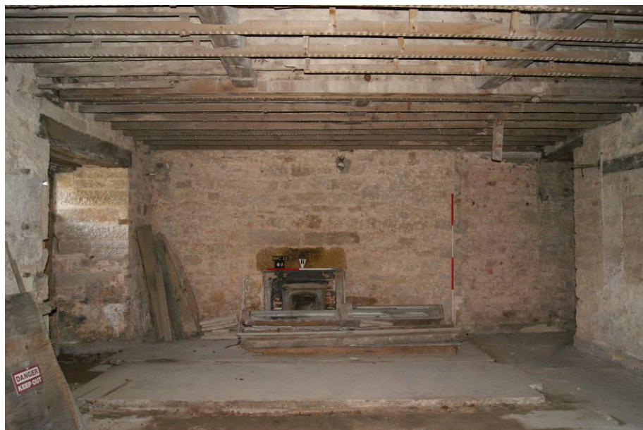
P77. R19 'Servants Hall' on the 1801 floor plan, looking south to fire [68]. Shows cement floors preserving the outlines of 18 th century partitions, overlying flagged flooring. These are proposed for removal. Brick blocking of [60] is visible (right).
