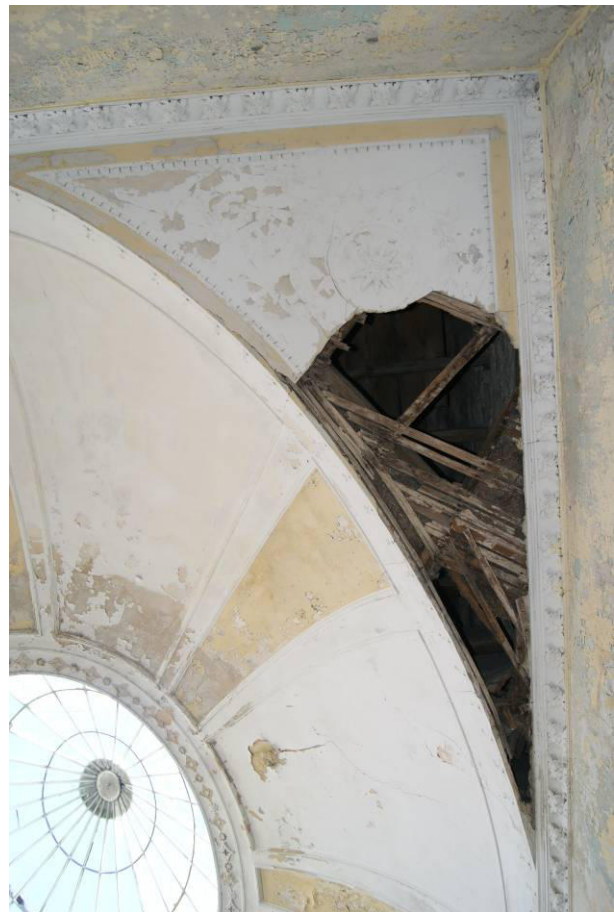
P147. R56. The second floor landing of the Great Stair, looking up in the south-west corner showing loss of decorative plasterwork to this spandrel of the cupola.
