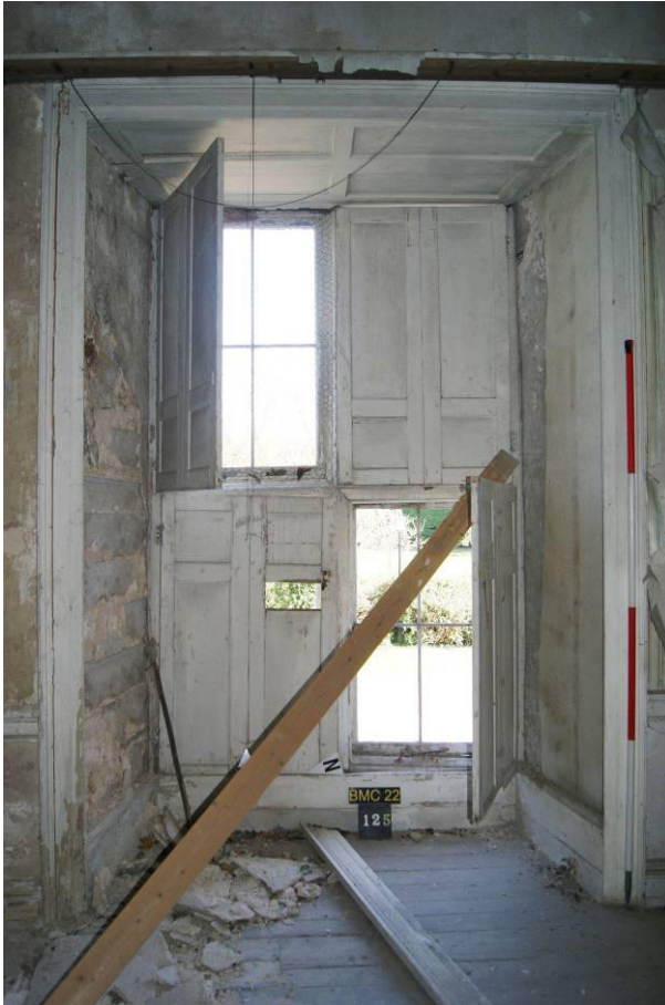
P131. R42. Window [125] showing plaster fallen from north reveal and delapidation since 2012.
