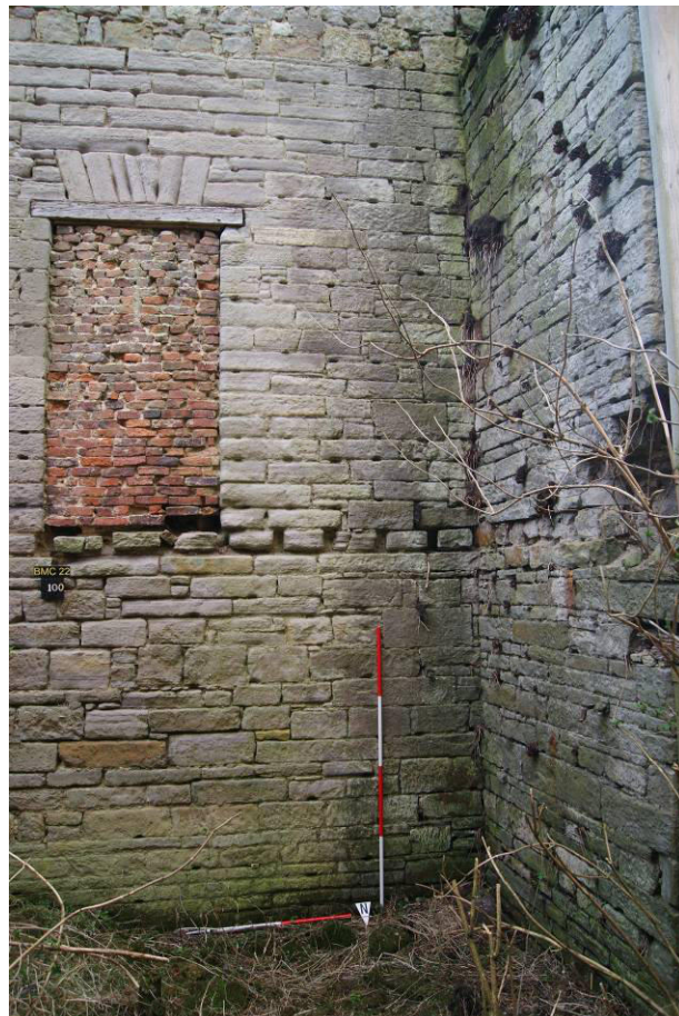
P93. R24, south wall showing first floor door [100] proposed to be reopened, with joist holes below and possible evidence for stitching the west wall of the 1810-4 north range. To earlier masonry
