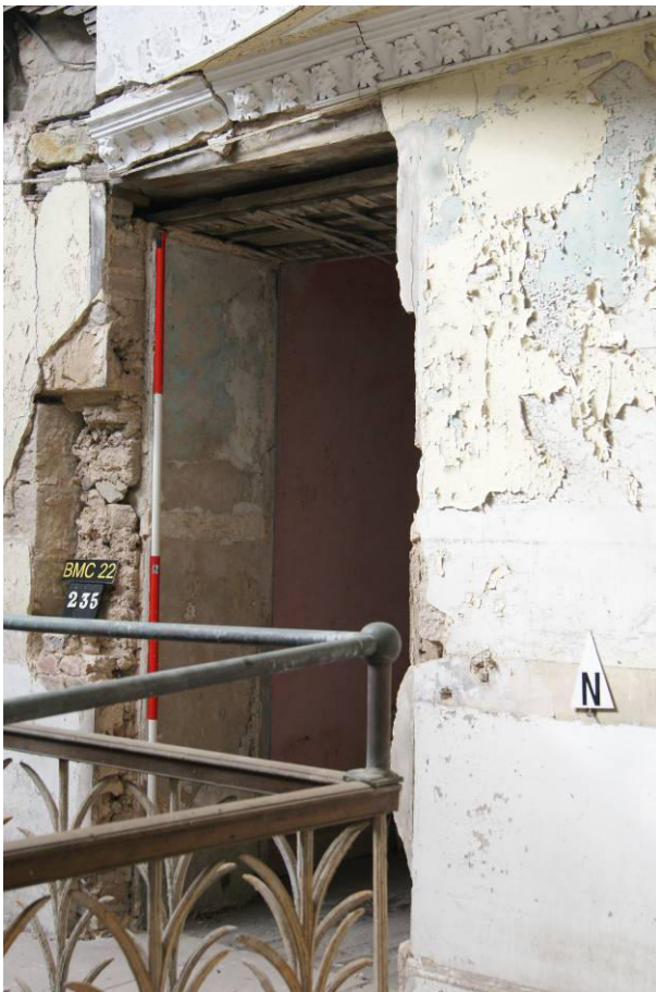
P152. R56. Door [235] showing that an earlier, wider, opening has been blocked. Also showing a loose section of the 1801-4 plaster cornice above.
