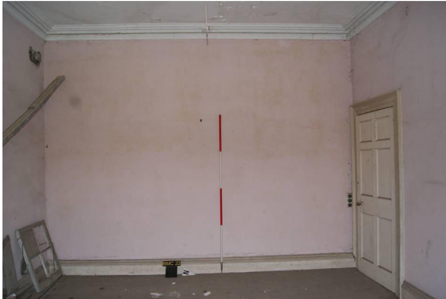
P143. R51 looking west to the site of the proposed new opening linking to R50. The wall is probably part of the c.1892 build.
