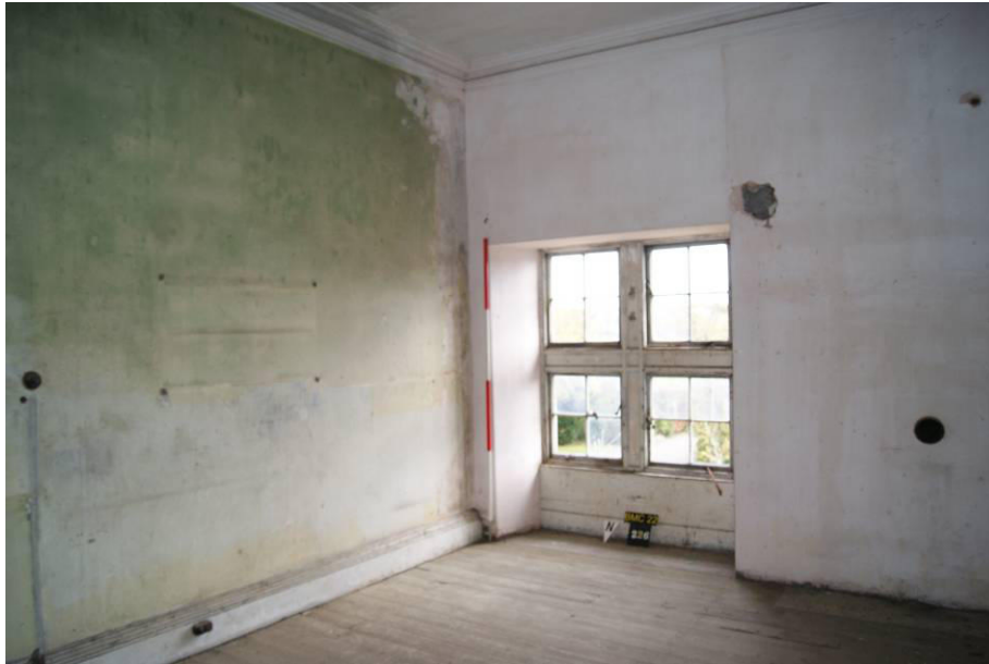
P140. R50 looking south-east. The east wall is proposed to be opened out into a wide opening linking to R51. The south wall and part of the ceiling above is late 20 th century plasterboard. The original fire has been removed.
