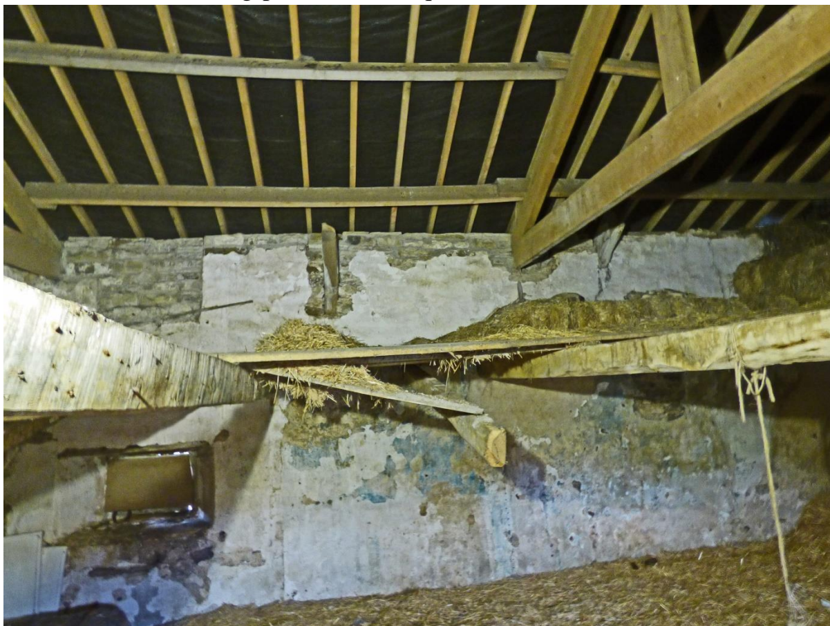
The Bastle-Derivative House; interior of north wall with collapsing second-floor beams, stubs of two upper cruck trusses and recent roof
