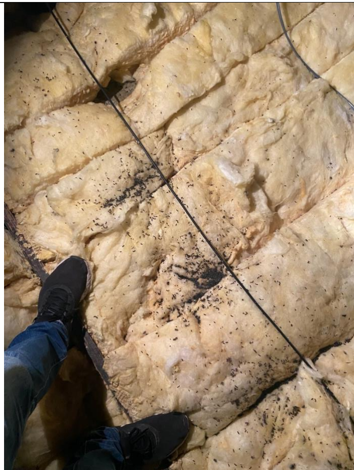
Photograph 2: Bat droppings inside roof void 1
