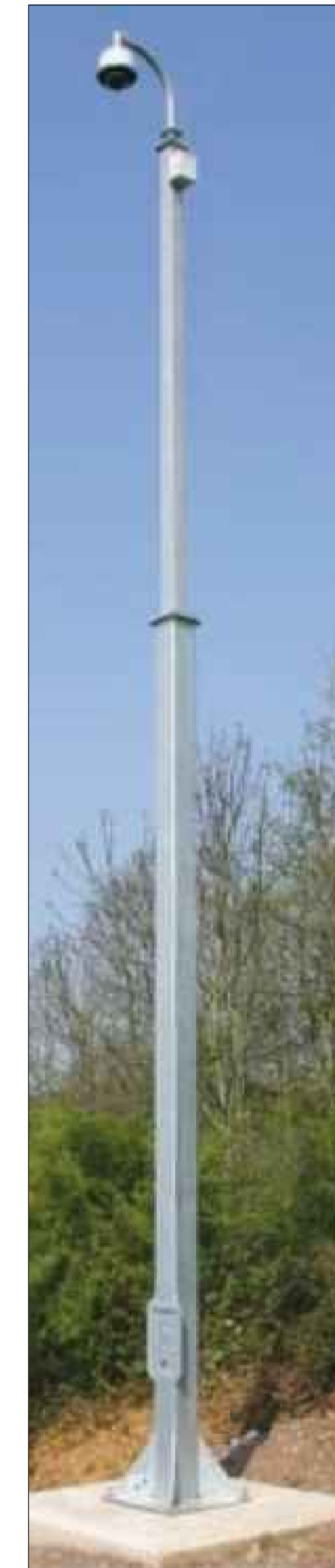
CCTV POST ILLUSTRATIVE PHOTO
