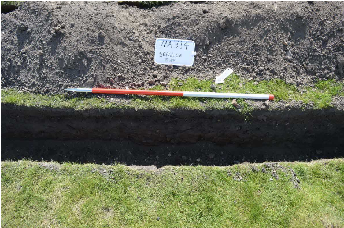
Plate 6: Service run –Looking Southeast.
