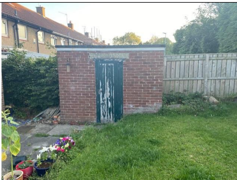
Photograph 7. Showing the north eastern elevation of the outhouse with various holes around the stone lintel of the entrance door.
