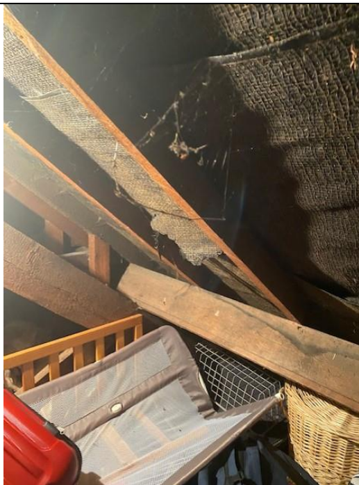
Photograph 11. Showing the accessible area of the loft with wooden framework and lined roof.
