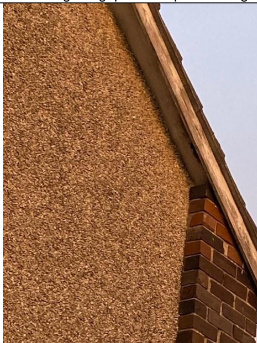
Photograph 10. Showing the water damaged to the fascia and soffit on the gable end.
