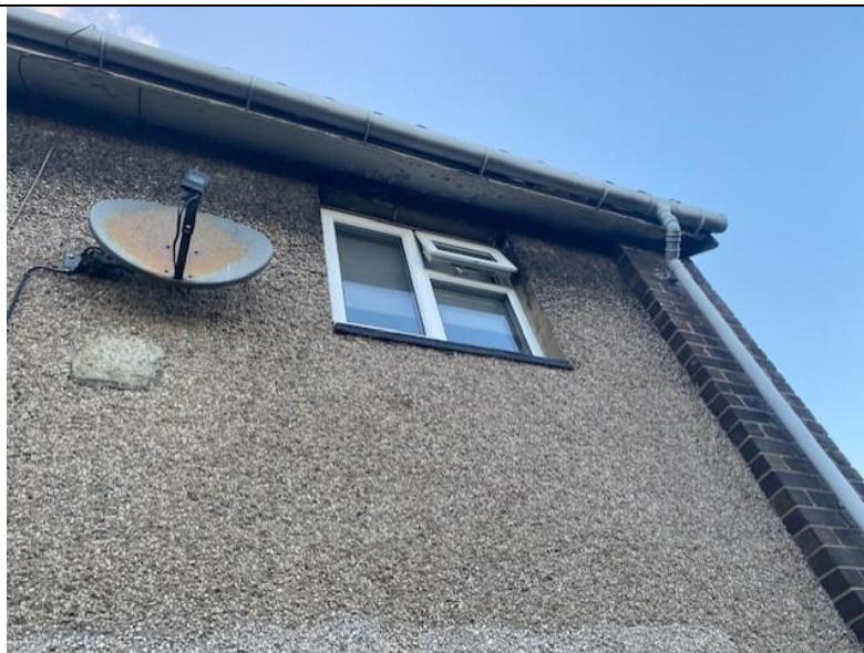
Photograph 3. Showing the pebble dashed walls, damaged wooden soffit and plastic rain water goods.
