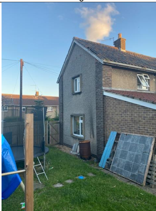
Photograph 4. Showing the north eastern elevation with the property, with damaged roof tiles on the rear elevation.
