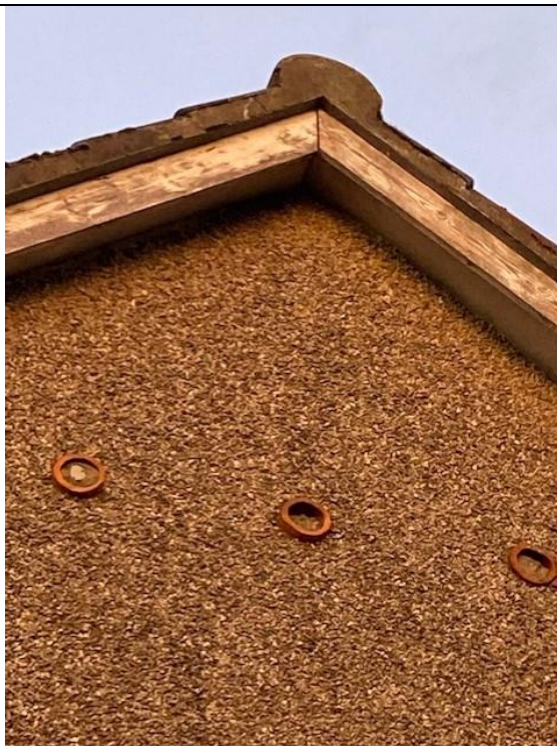
Photograph 9. Showing the gap at the apex of the gable end fascia.
