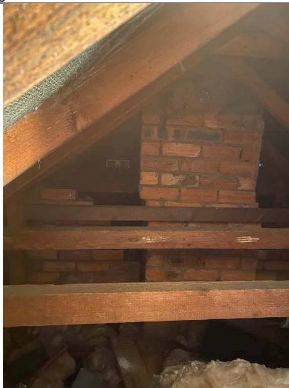
Photograph 12. Showing the view into the inaccessible area of the loft due to the chimney and timber framework.
