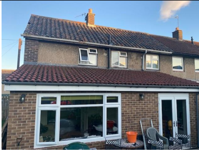
Photograph 5. Showing the rear/ north western elevation with the existing single storey extension.
