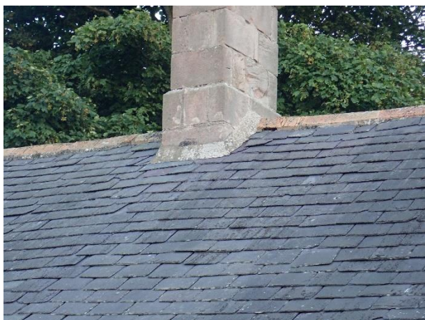
Gap near the chimney
