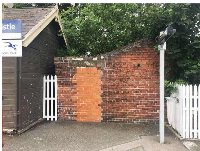
Figure 3: Platform 1 - Former Gent's toilet block with collapsed roof
