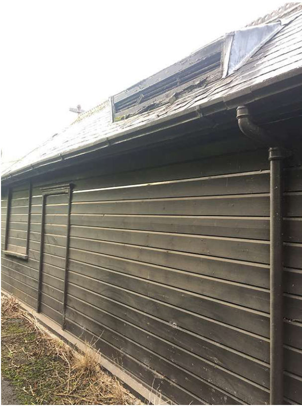
Figure 28: Platform 2 - Deteriorated ventilation dormer above existing toilet area
