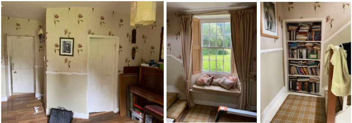
Existing internal images of Ground Floor eastern room - far right image of bookcase is location of original door to house. Proposed works to raise the lintel were outlined in the Heritage Report produced by Sarah Dyer that accompanied the existing LBC permission (Sarah Dyer).
