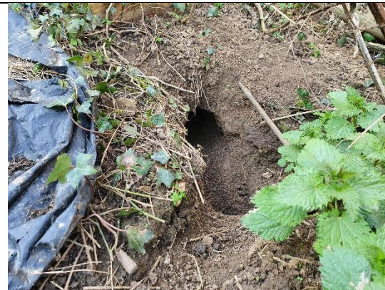
Photograph 4: Rabbit holes to the rear of site.
