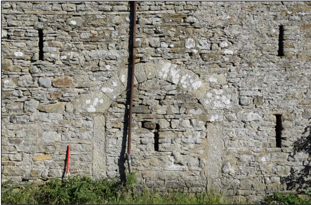
Photograph 33: Detail of the central door, with its unusual pointed arch. The break in the masonry runs diagonally above the right-hand side of the arch
