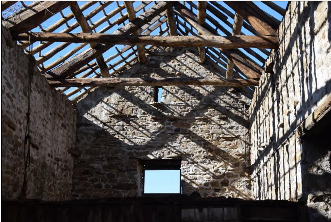
Photograph 37: The hay loft at the west end. There are more through stones here than on the outside faces of the walls. Note the crude roundwood timber of the replacement roof
