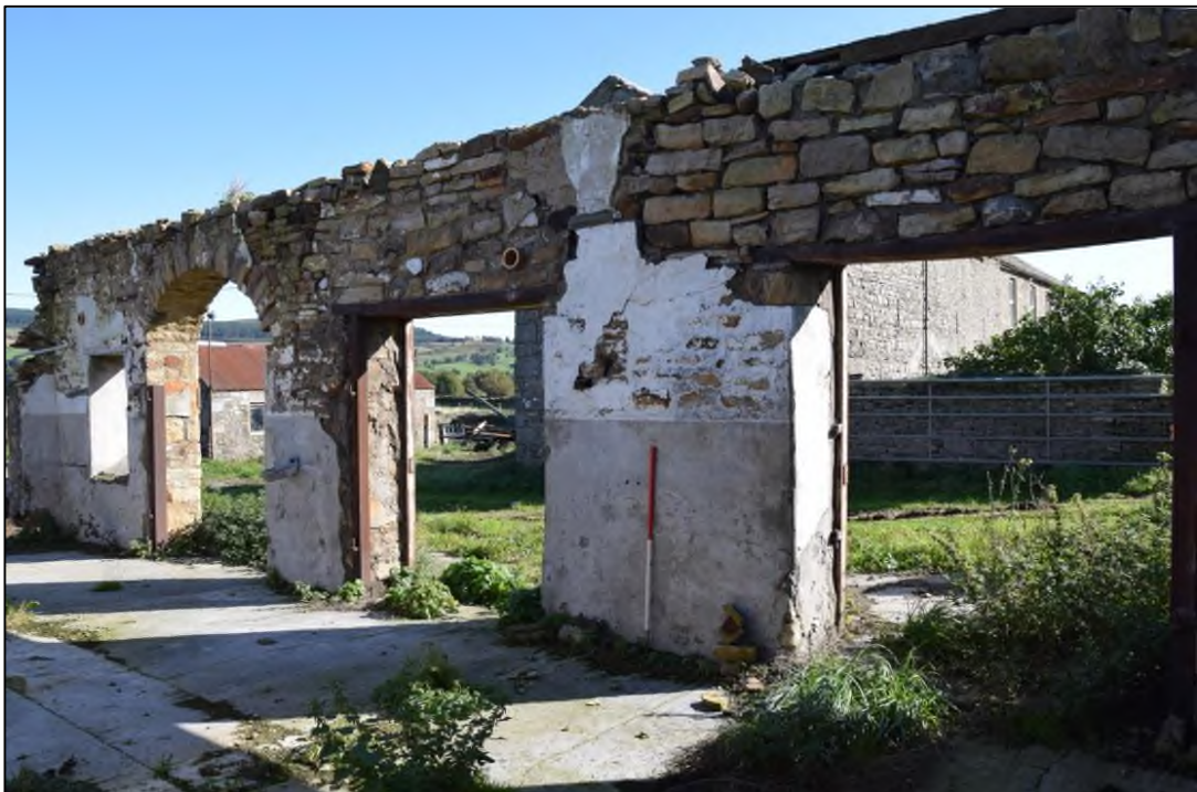
Photograph 58: Much of the upper part of the east wall has been rebuilt in recent times
