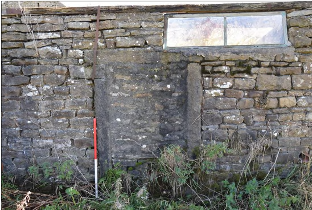
Photograph 52: Detail of the blocked door, later reduced to a window, in the west face of building 4
