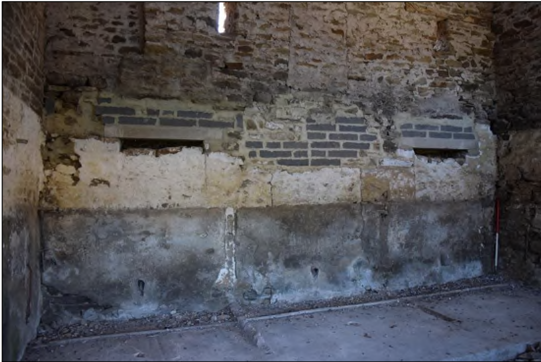
Photograph 21: The south wall of the byre in the west extension. The arrangement of stalls, the wall finishes and the recent repairs are the same as those seen elsewhere in building 1
