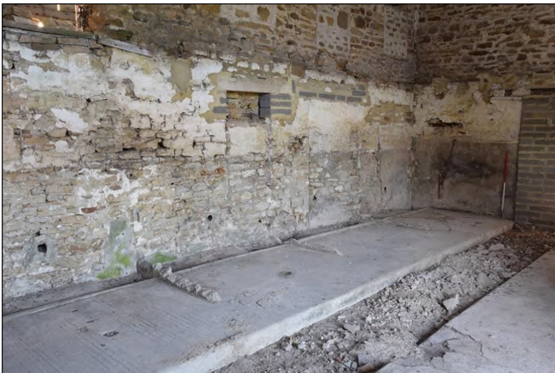
Photograph 16: A view looking south-west in the old part of the building. Older masonry fills the first-floor windows, above the recent repairs
