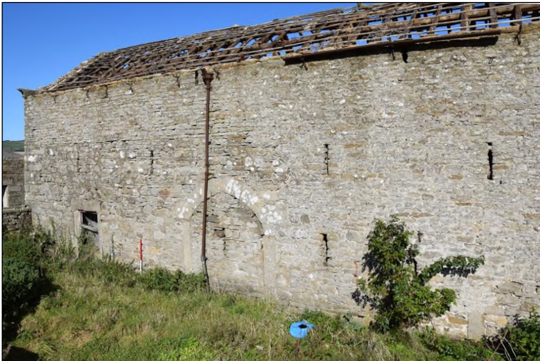
Photograph 32: The small door at the far end was matched by another at the east; the lower jamb can be seen below the shrub at the right
