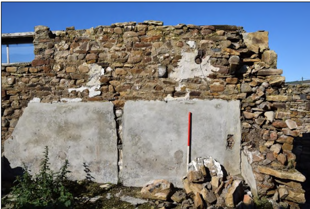
Photograph 56: The stubs of two joists can be seen above the cement render at the north-west corner of building 4
