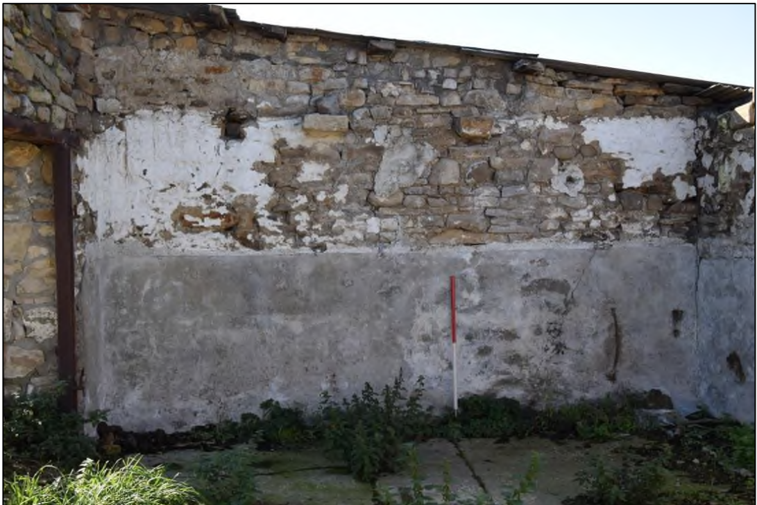
Photograph 62: Cement render on the south wall. The whitewash above indicates the line of the old ceiling
