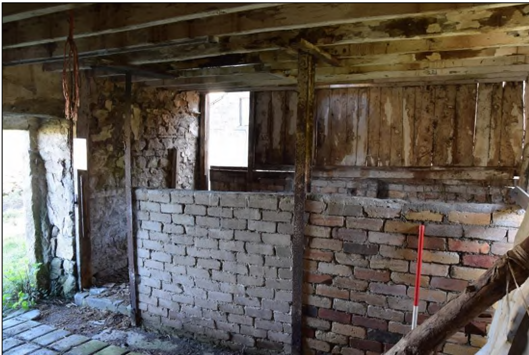
Photograph 38: A view looking north-east in the byre, with steel I-beams supporting the ceiling
