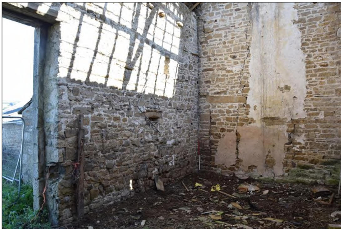
Photograph 44 (below): The east end of the north wall, with a small blocked window that is now covered by a lean- to shed outside
