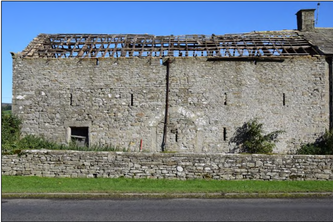
Photograph 31: The south face of building 2. The change in fabric can be seen as a neat horizontal line above the left-hand pair of breather slits
