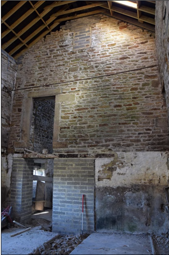
Photograph 23 (left): The west face of the internal wall, formerly the end of the building
