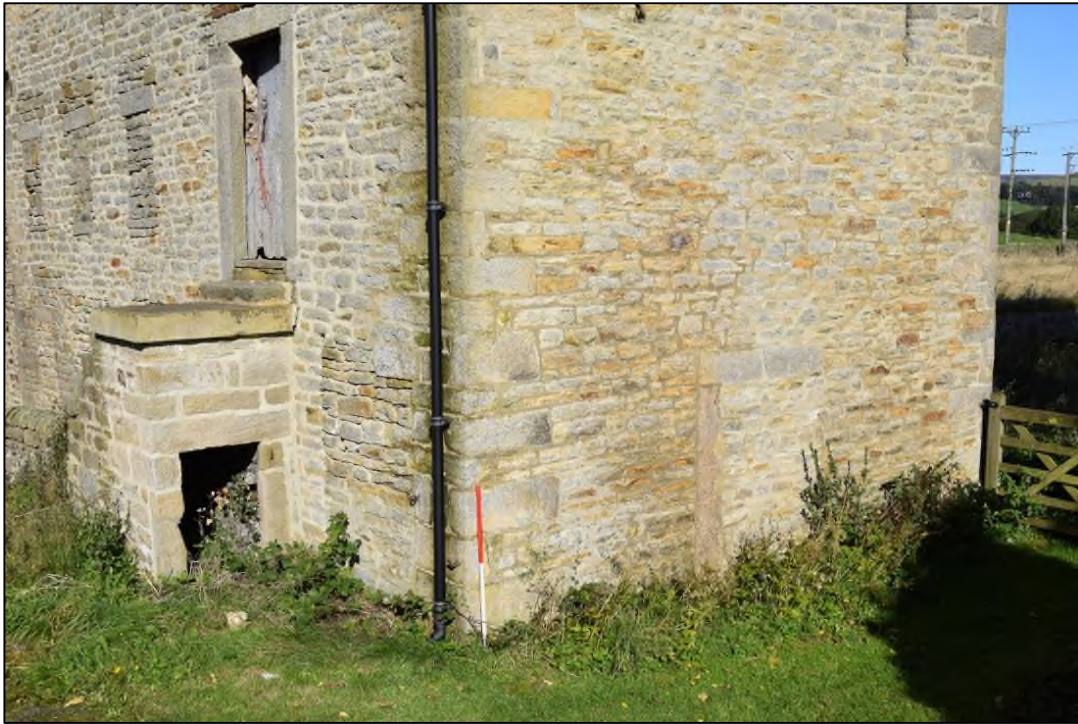
Photograph 5: The blocked opening at the east end of building 1. Recent repointing is apparent, as is the rebuilding of the stone staircase
