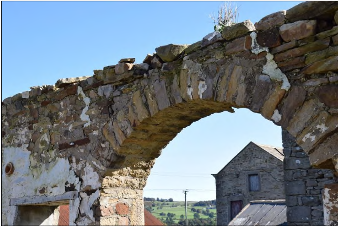
Photograph 61: The arched door is also a recent alteration. There are no traces of similar arches on the rest of the wall
