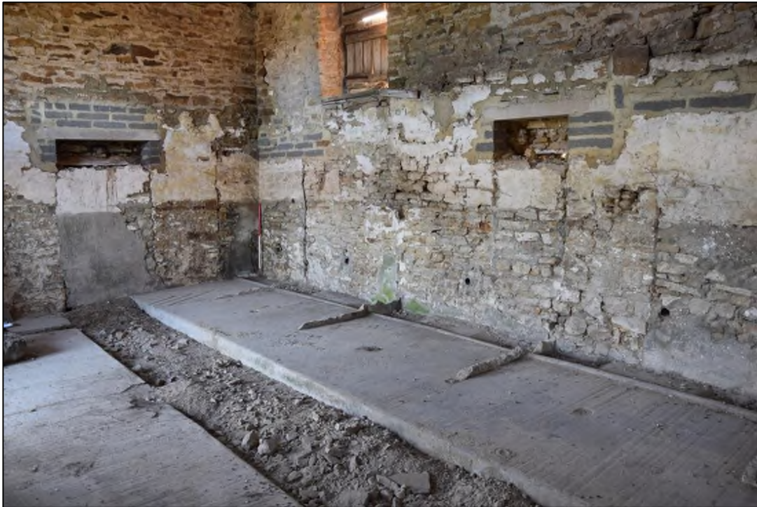
Photograph 15: Inside building 1 are the remains of 20th-century cow stalls and a large floor drain. Recent repairs to the door and window lintels can be seen. A view looking south-east
