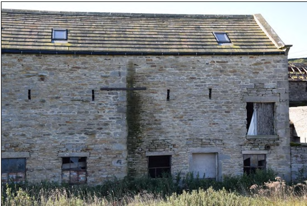
Photograph 12: The north face of the extension, with the reinforcing iron band across the junction
