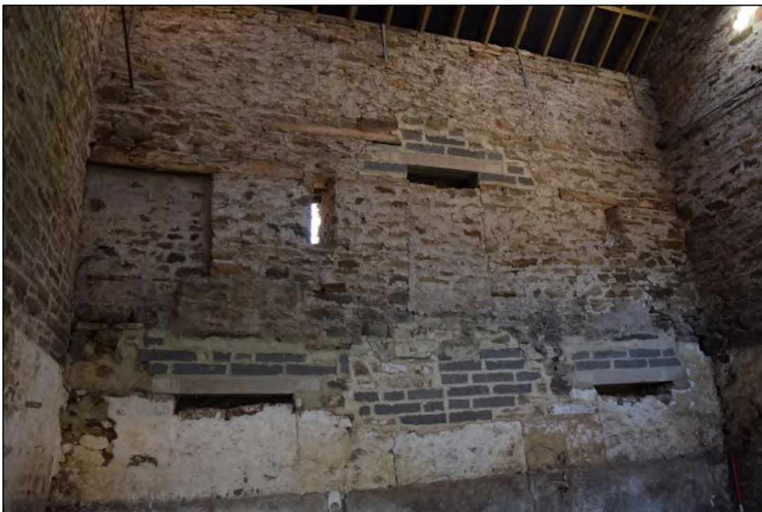
Photograph 22: Blocked openings, breathers and repairs in the upper floor of the south wall
