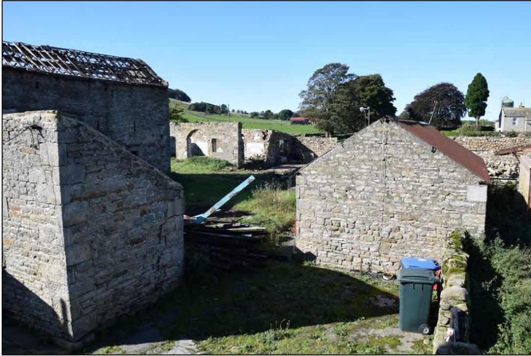
Photograph 63: A view looking south-west across the yard at the west end of the steading. Building 5 is at the right and 4 in the background; building 3 is at the left
