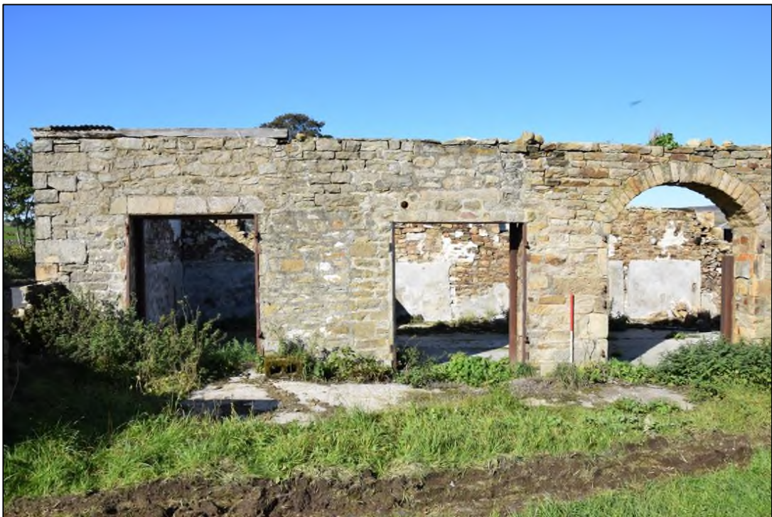
Photograph 48: Steel frames support the doors at the south end of the building's east face
