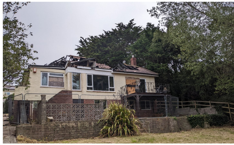
Rear elevation. Wide glazed windows facing south to views. Prefabricated steel framed terrace, block/brick retaining walls creating a divide between house and garden level.
