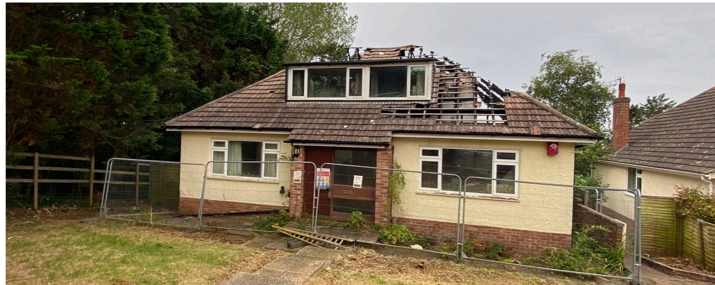
View of front elevation. Large mansard north facing window, white UPVC windows and flat concrete tiles
