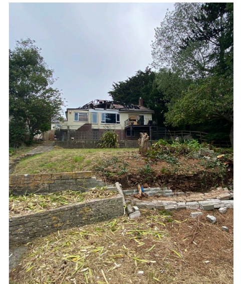
View of rear elevation. Existing garden retaining walls requiring repairs
