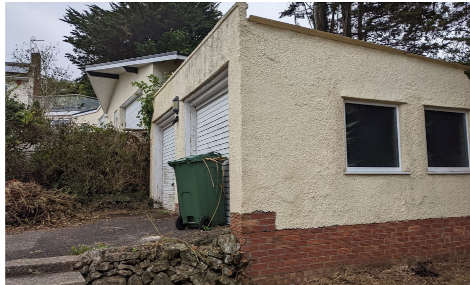
South side of double garage (opposite woodrising). On an elevated position than the main house. Brick base with render above and side windows. Northern neighbour shown beyond on elevated landscape.
