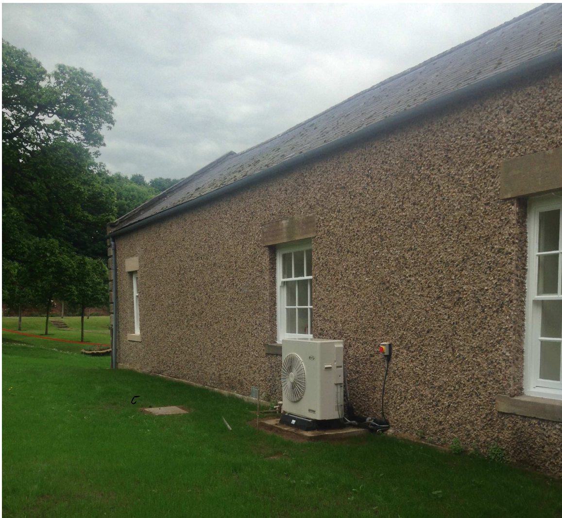
AIR SOURCE HEAT PUMP INSTALLATION
