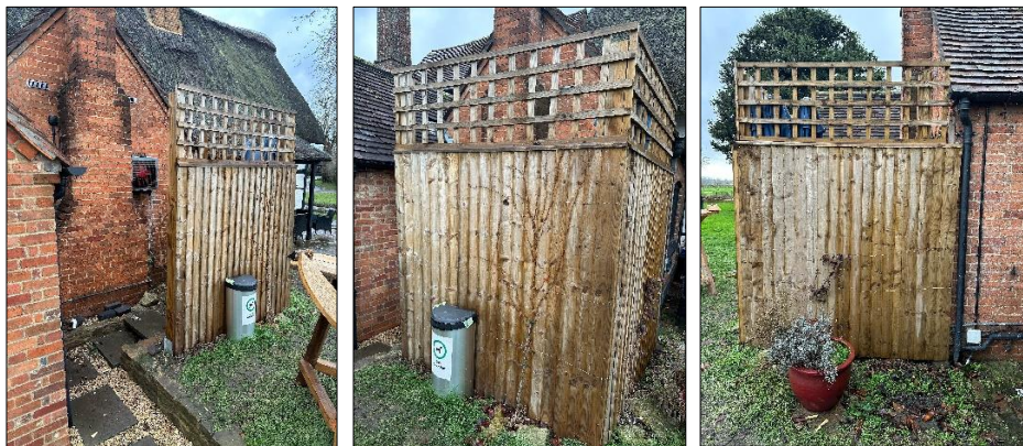
Fencing around the air conditioning unit
