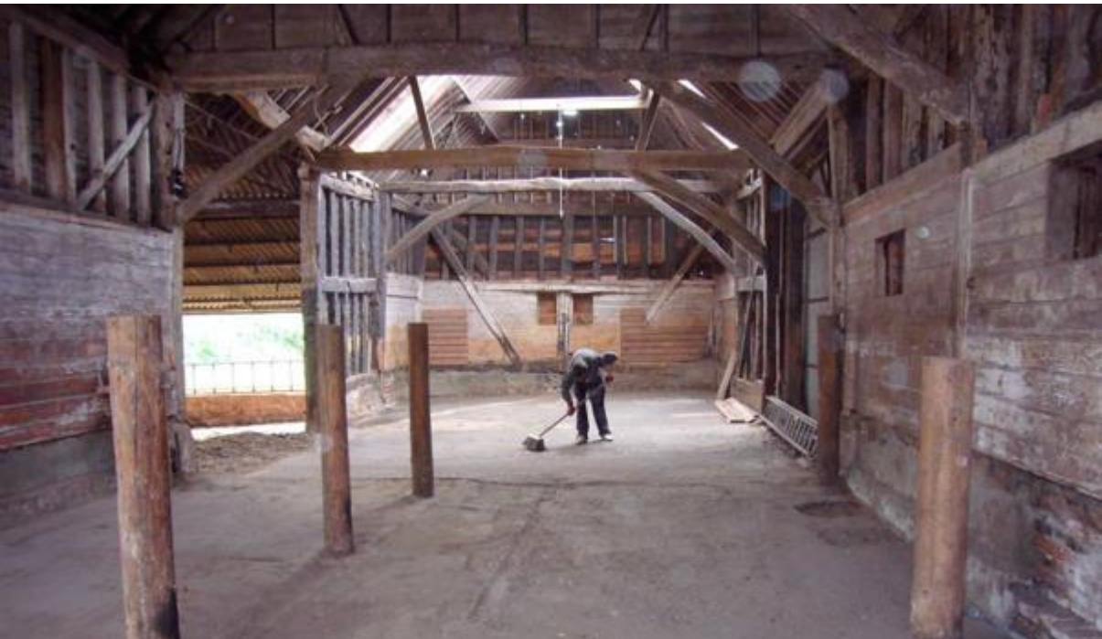
Photo 6 – Internal Photo of Heritage North Barn, from E, showing ventilation openings that are currently boarded over
