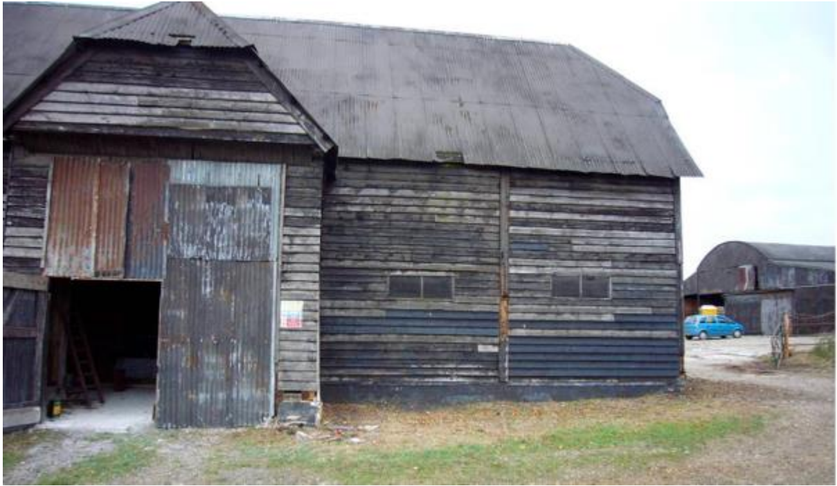
Photo 3 – South elevation of Listed Barn showing makeshift midstrey doors. Dutch Barn can be seen to NE
