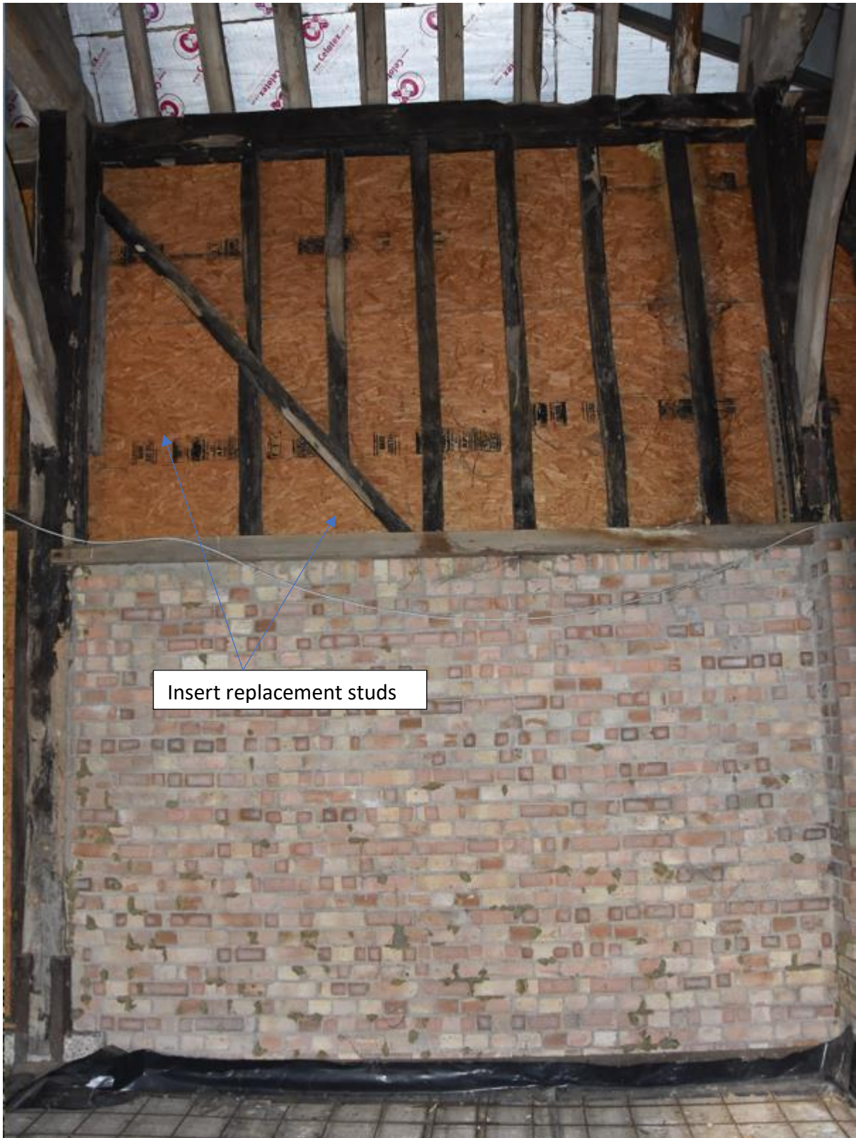
Fig22. Bay 4 North Wall
