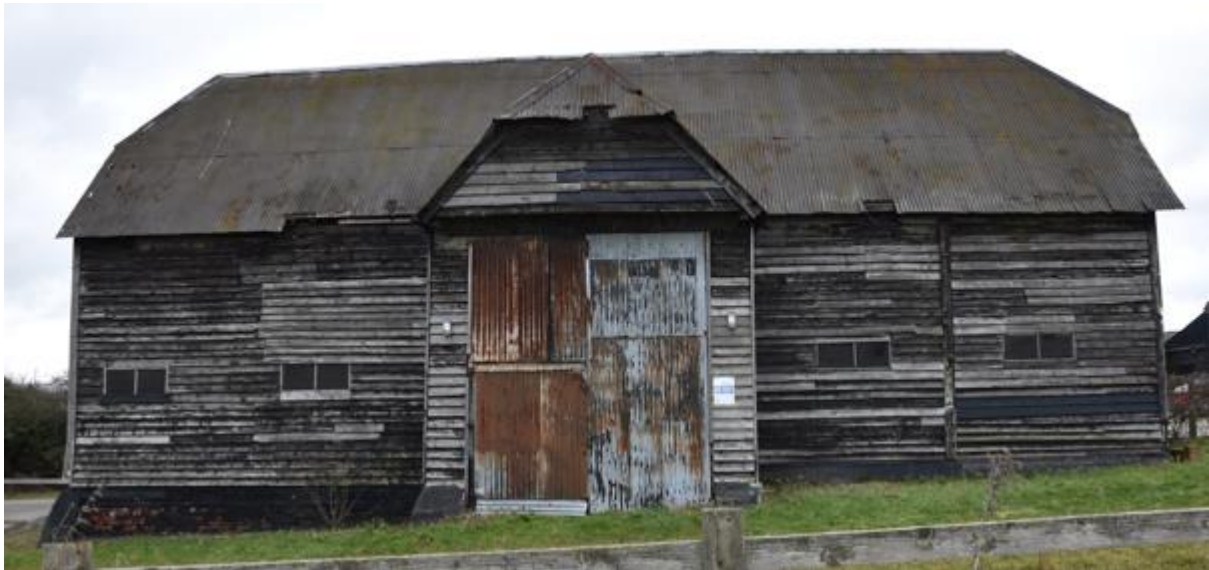
Fig1. South Elevation – Repair projecting top plates. Replace Corrugated Sheeting with slate. Install new metal gutterwork & downpipes. Glaze doors and ventilation gaps. Replace cladding with large section sawn weatherboarding in black.
