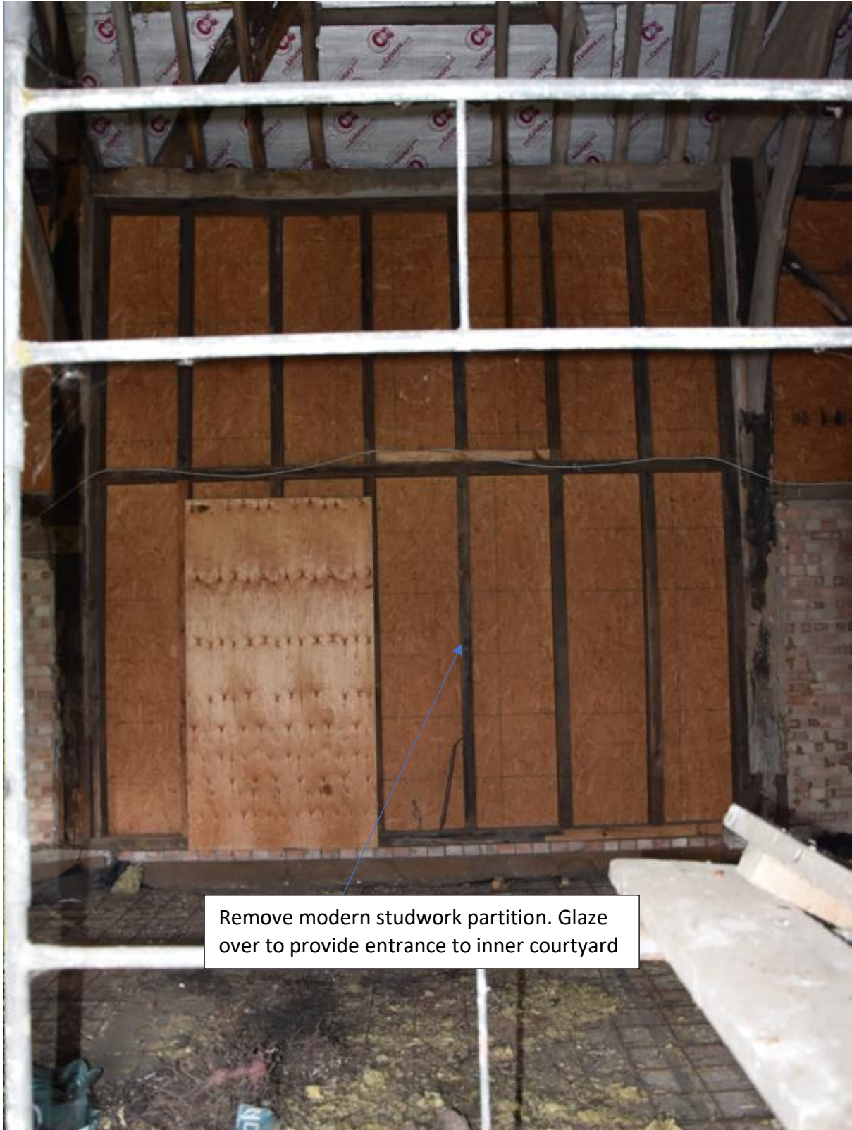
Fig24. Bay 3 North Wall
