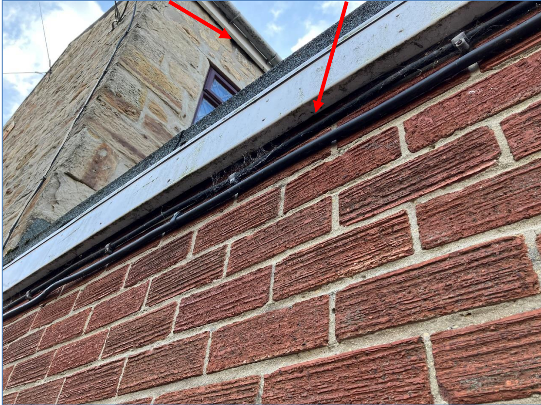
Photograph 3 – Gaps visible at first floor soffit. No gaps at ground floor extensions
