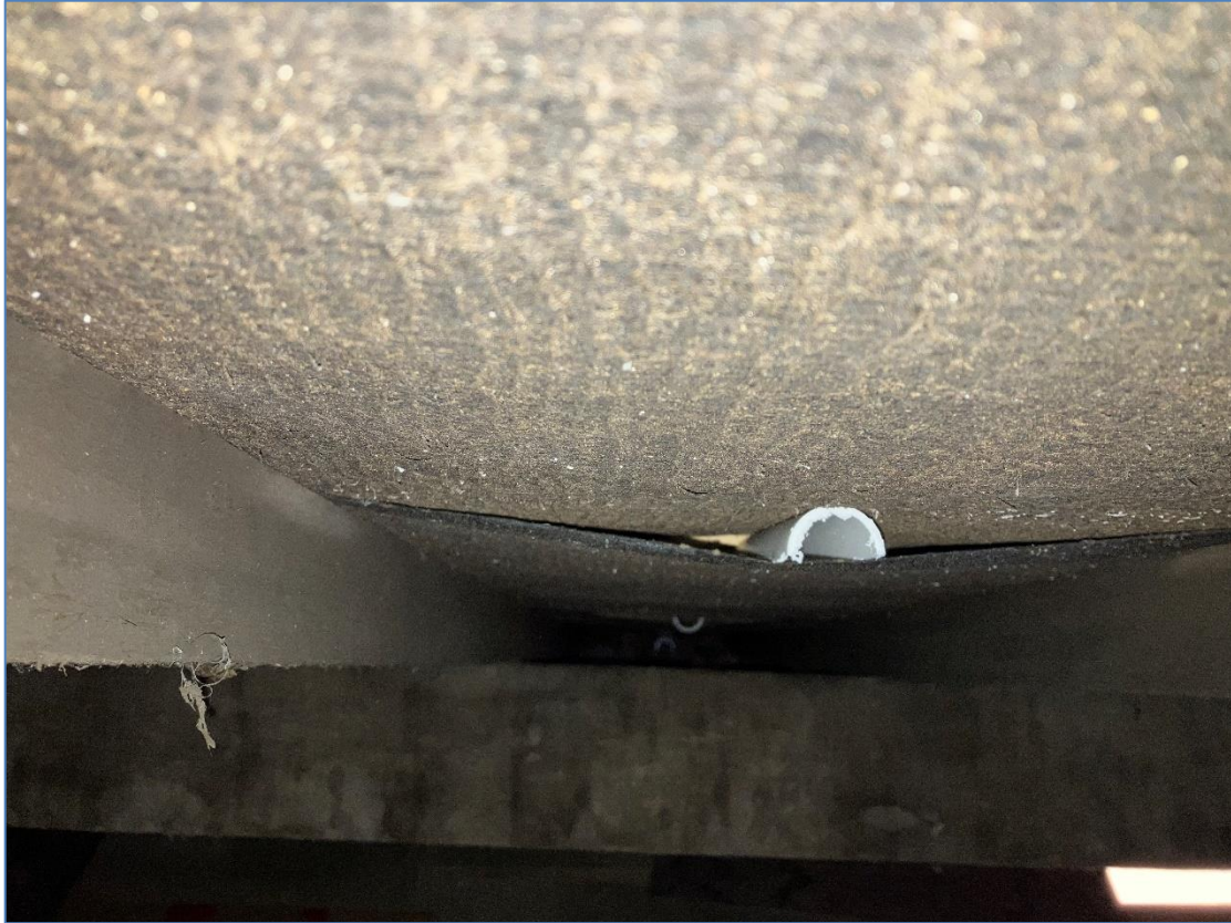
Photograph 5 – Ventilation in the roofing membrane which would allow bats access to the roof void
