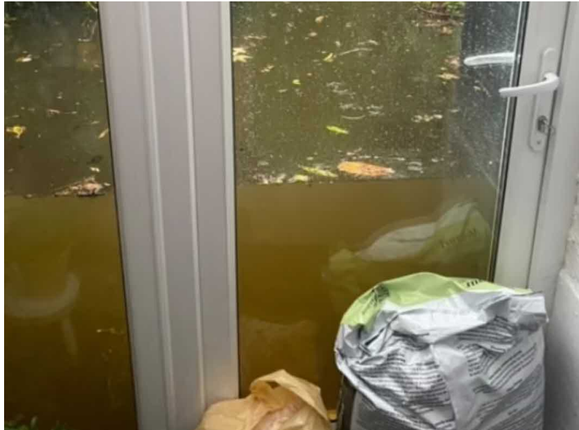
Figure 8: UPVC doors under flood conditions. These appear to offer reasonable flood resilience
