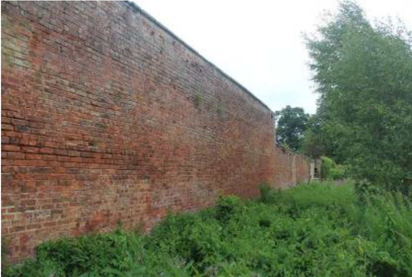
Garden wall looking ENE, showing change in wall height away from outbuildings to N.
