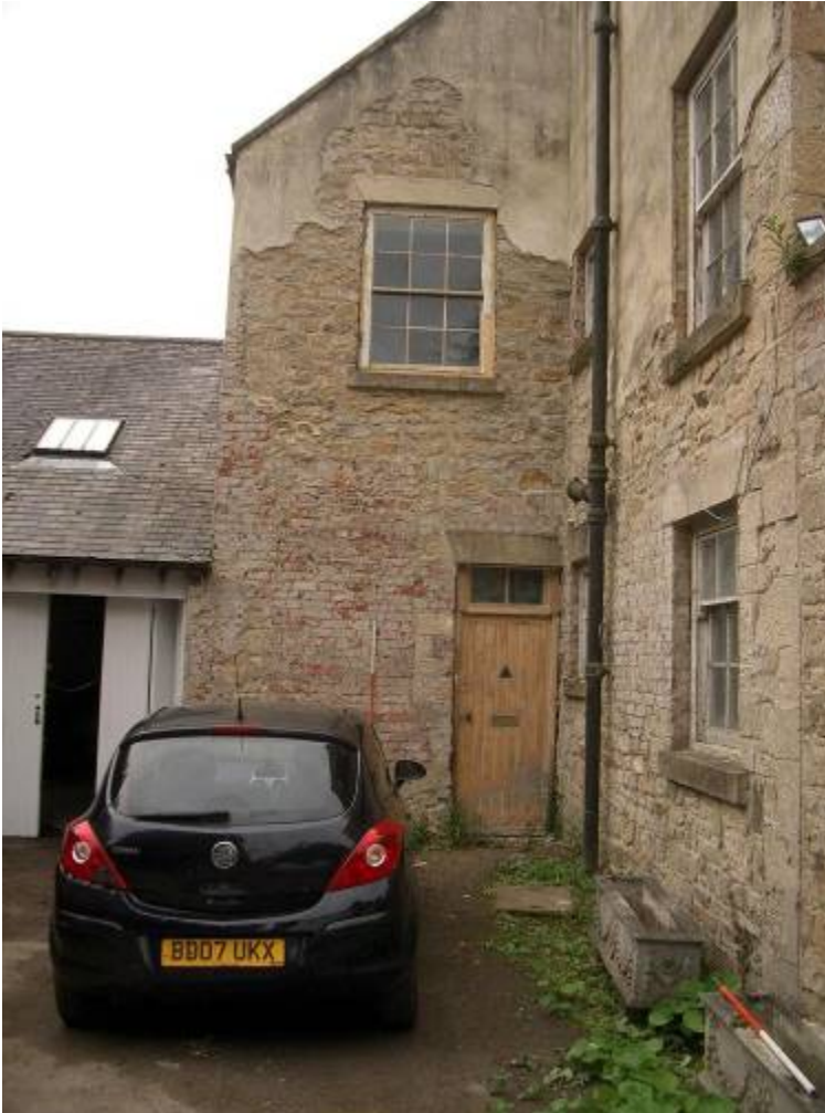
W end of C18 double span block in rubble stone. Note no quoins and ragged brickwork up LH return and poss. brick blocked opening behind car. W31 No horns on sash
