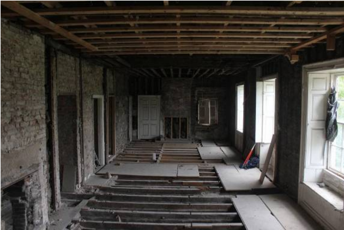
General view looking east from breach in W wall. FP8 L. foreground
