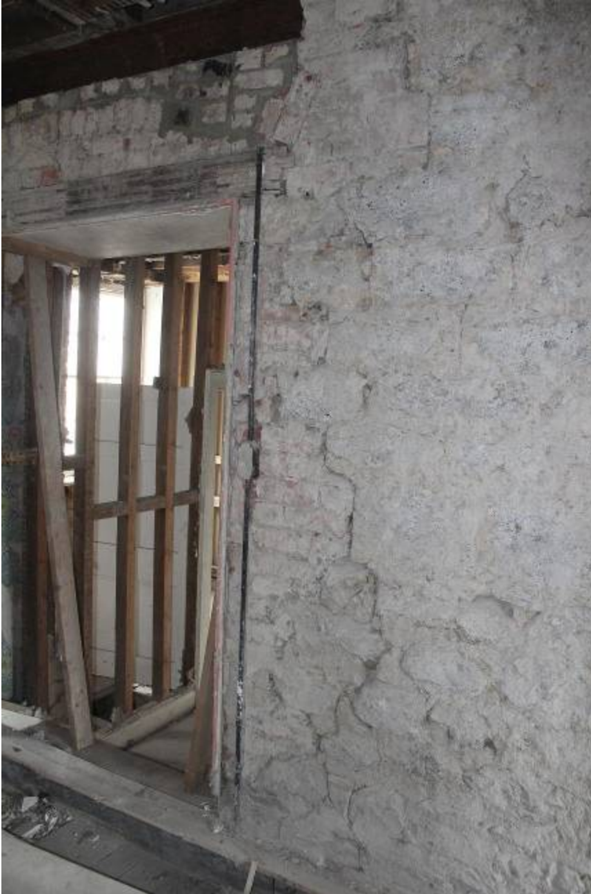
Ragged break in rubble stonework of late C18/early C19 build to R, Brick infill and relieving arch over change in level of corridor and beam above 1880's work
