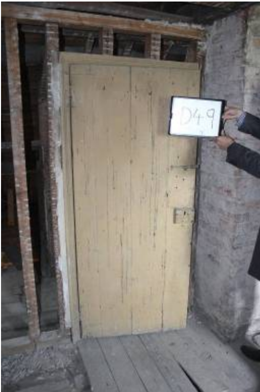
D49 room side. A much simpler and earlier (hinges) plank door, perhaps contemporary with FP13
