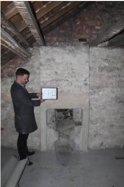
FP13 A modest C18/early C19 hob grate for coal burning. Note 1880's brickwork above where this gable was raised for adjacent extension
