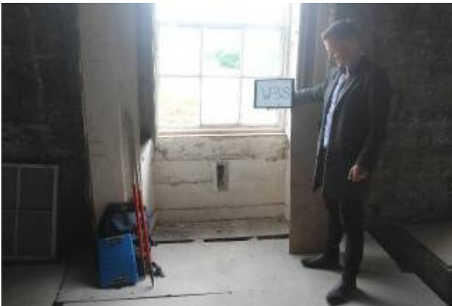
W38 A sink was installed below the window in the C20 bathroom
