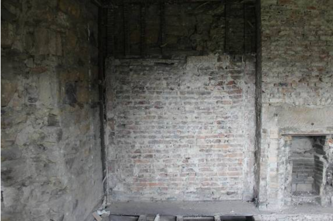
Brickwork panel infilling former doorway (now corridor cupboard served by D22) on N wall to L of FP8
