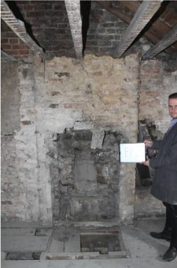
FP12 ?C18 hob grate here orig. , as FP13, but modified for C19 CI fireplace (fixings and outline).
