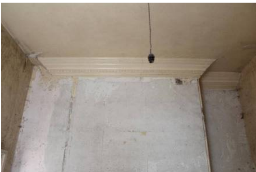
Cornice above FP2. Removed for ?1930's "Cloaks" partition (left) and continues beyond WC partition (right).
