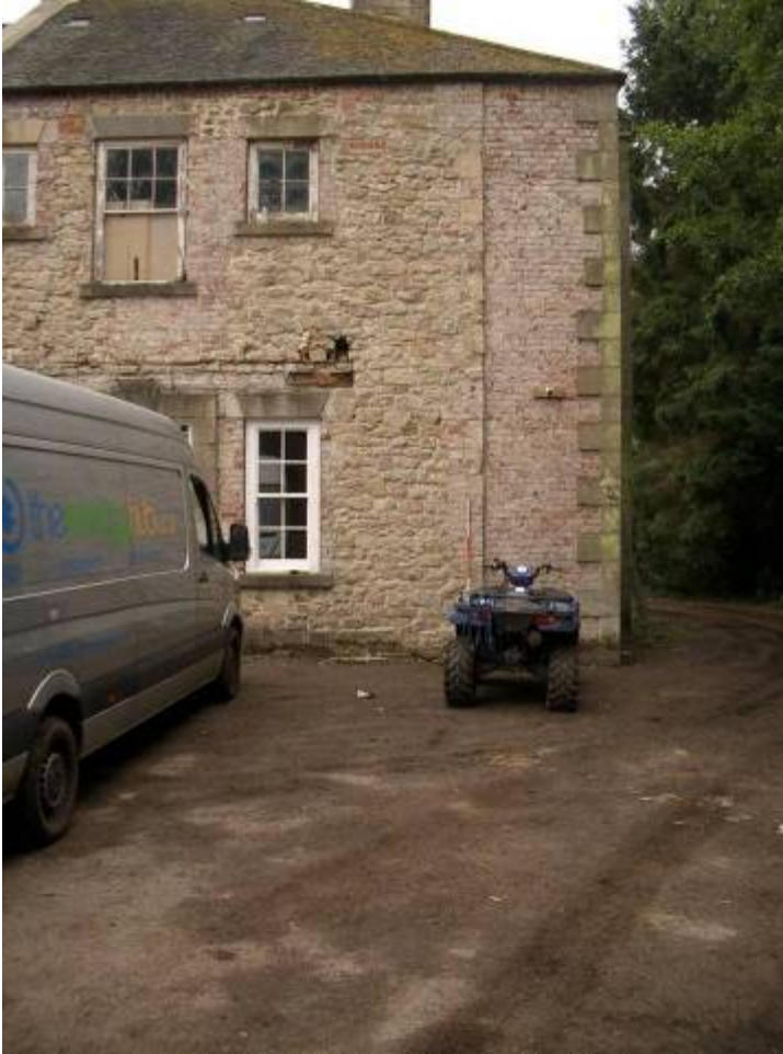
Cut back return of lost NW range. Sockets for previous FF joists above embedded timber. 1880s brick addition to R.
