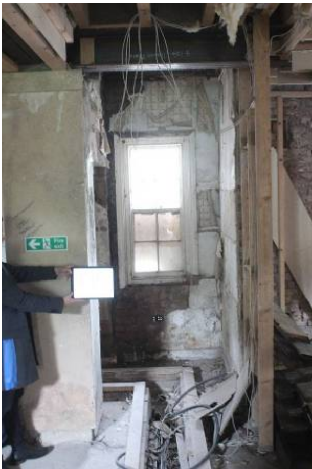
Location for P19, looking west. Note RSJ above and floor duct from previous works
