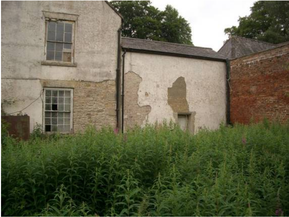
E wall of garage brick matches higher section of garden wall to R. D4 modern. Note old electrical insulators fixed to W32 (estate had own supply in 1880s)
