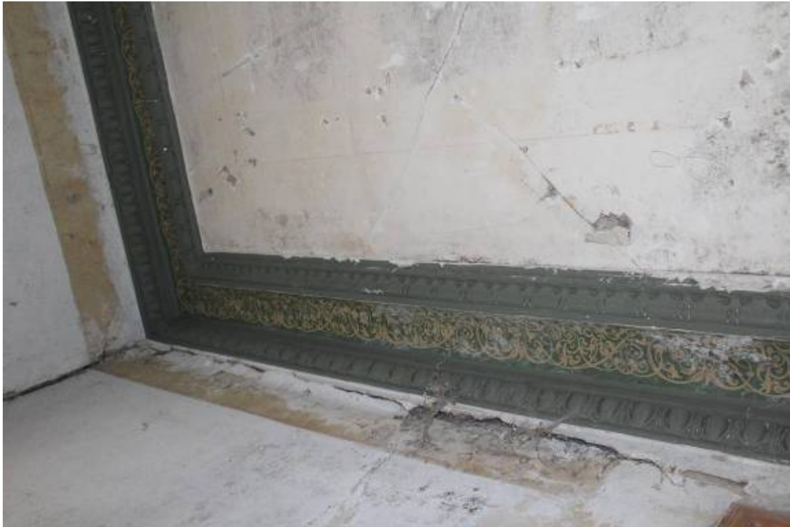
Cornice detail (badly damaged ceiling)
