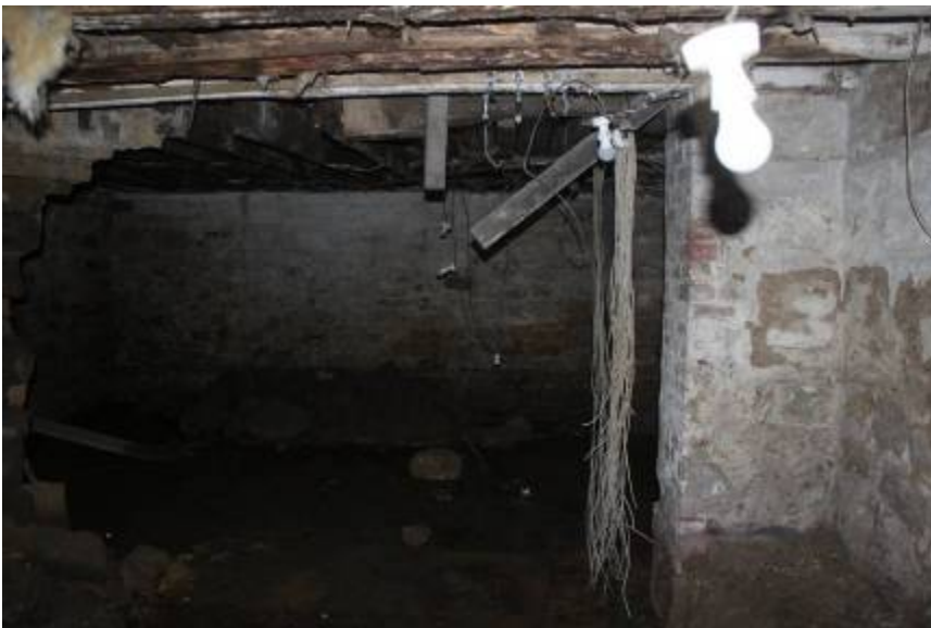
N side of doorway between 1840's cellar and 1880's cellar beyond. All of dividing wall to L removed leaving joists hanging
