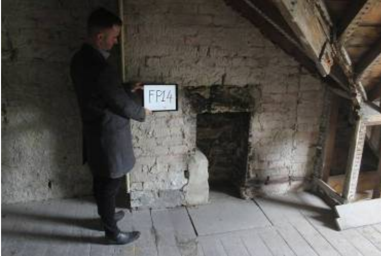
FP14 Modest 1880's attic bedroom FP. Note rot damage to roof timber to R.
