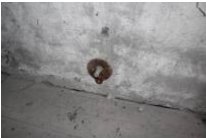
Fitting low down on N gable to RHS of chimney stack – tallies with external fitting - for wiring?
