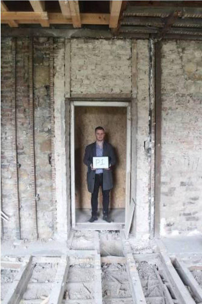
Bedroom side of D28, to be blocked (P1). Note blocked FP to R. C20 western bathroom partition in front of it
