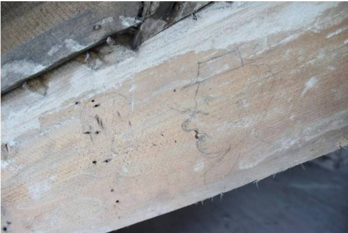
Graffiti on roof timber RHS W48
