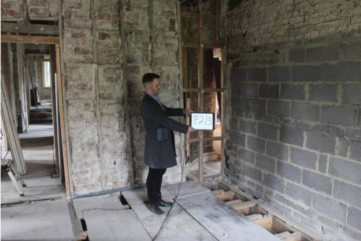
Location of airing cupboard in NW corner (removed). Proposals 2 and 3. Blockwork to R. over modern intervention to open up areas below. Old brick above
