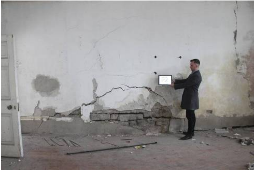
Settlement cracking in E wall due to breach made in cellar below Proposal GF2
