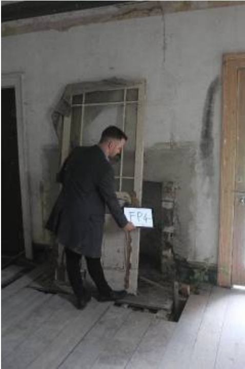
FP4 (removed). Is the door in front D13?
