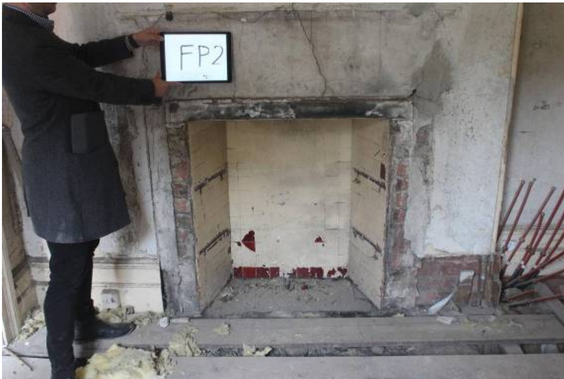
FP2 1930's tiled insert to original construction hearth? The pipework to R is from an attempted modern underfloor heating installation. Some skirting surviving
