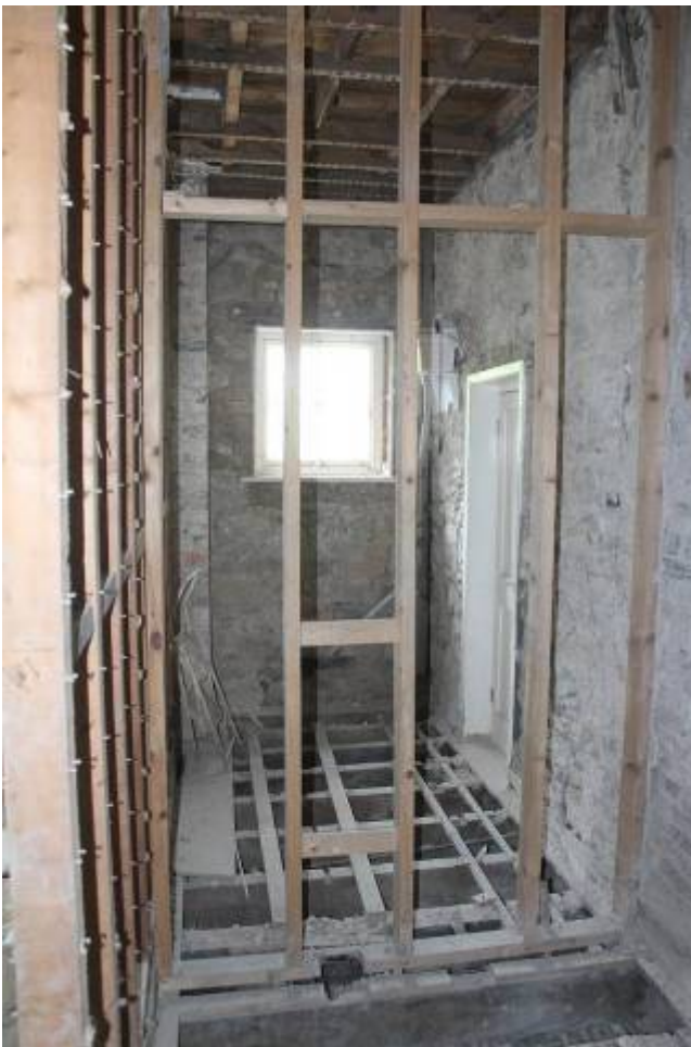
Looking N into northern bathroom. Inserted W30 and high level cistern suggest 1930s alteration
