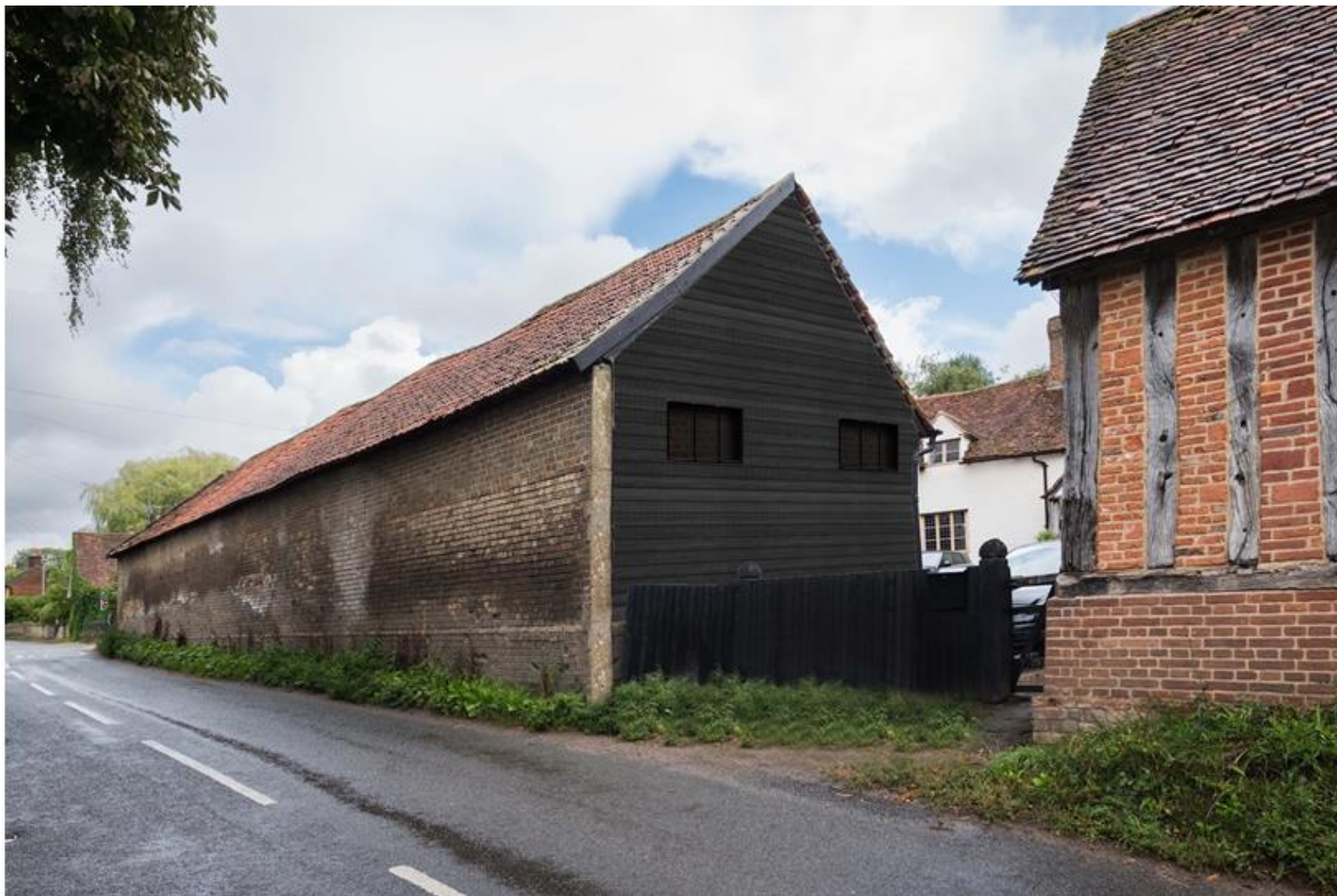
Figure 2 Proposed view of south gable end with render removed and horizontal timber boarding repaired/reinstated.
