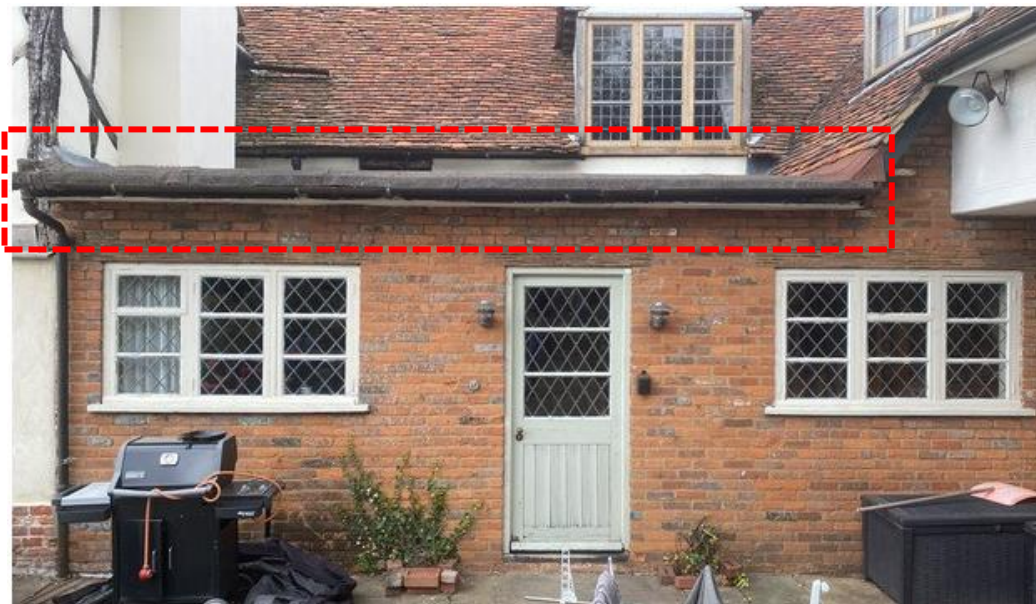
Above: Photos of the flat roof extension and area of mineral felting to be replaced.
