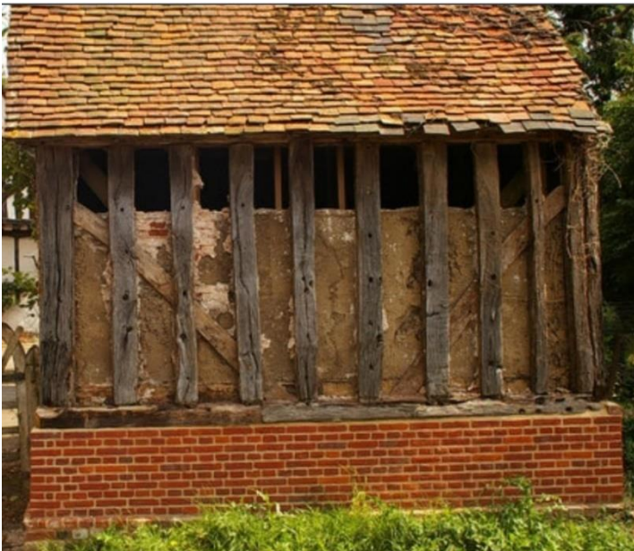
Above: The west elevation of the Granary whilst repair works were undertaken c.2018
