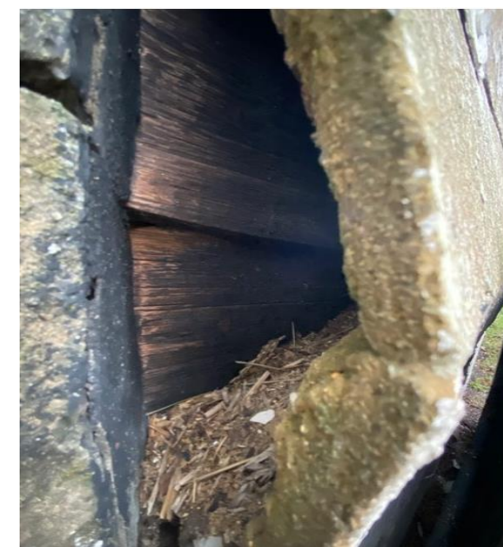
Above: Photos of delaminating cement render and underlying timber weatherboarding
