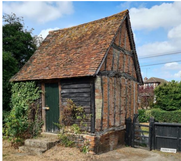
Above: View of the east and north elevation showing exposed timber frame and weatherboarding
