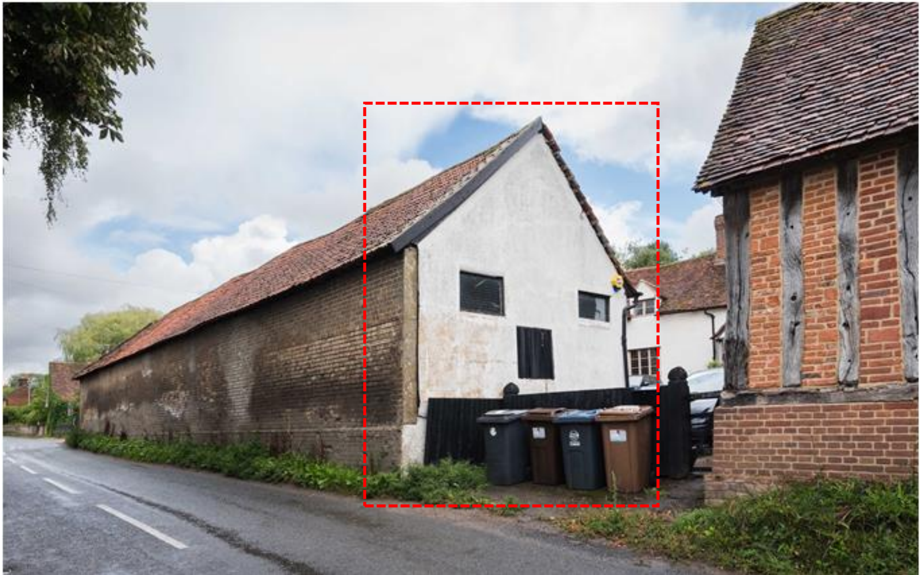
Figure 1 Existing view of south gable end with delaminating cement rendered finish. Extent of works indication in red.
