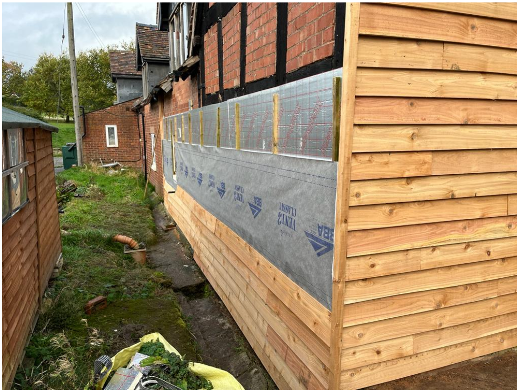
Showing insulation and breather membrane on West elevation and completed over boarding on South elevation.
