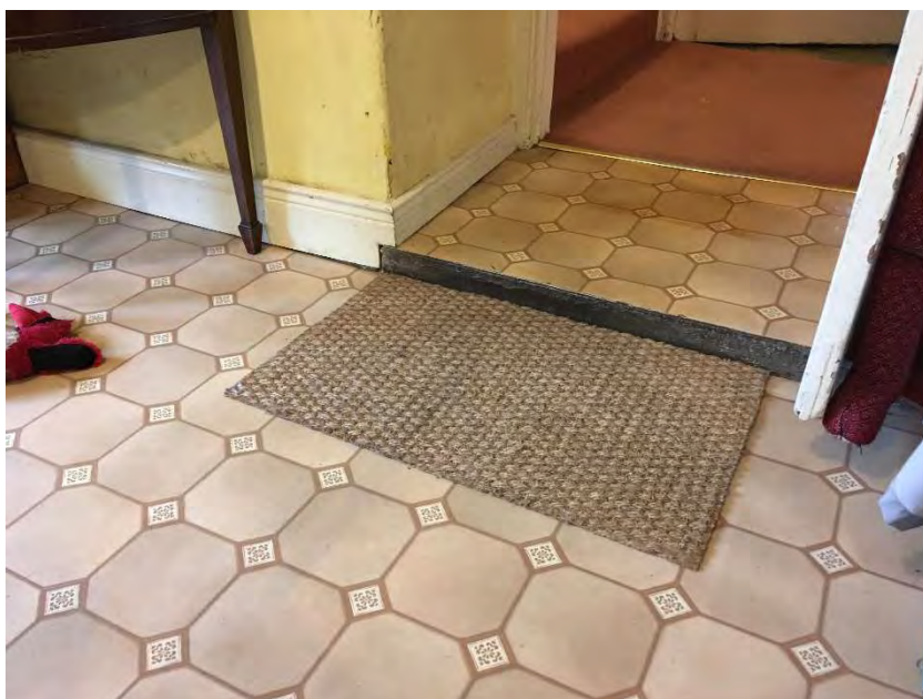
Photo 12 Vinyl flooring to kitchen over cement screed with 70mm step up into north wing.
