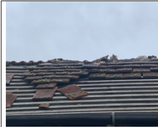
Photo 7: Example of the slipped and missing tiles on the south-western elevation.
