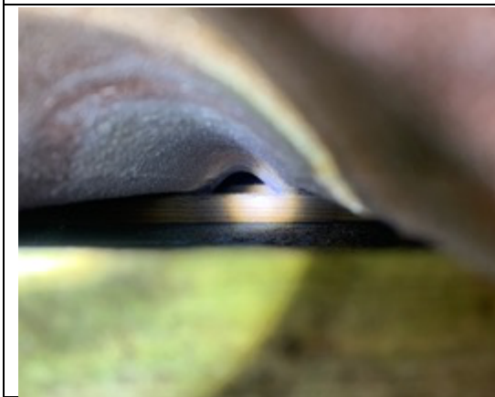
Photo 9: Showing the inside gap below a Tuscan tile, and roofing baton that may obstruct bats from roosting deep within the space.
