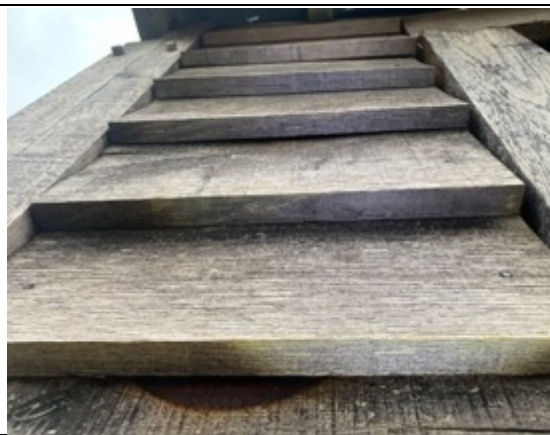
Photo 10: Example of wooden cladding in good condition with minor gaps on the south-western elevation.
