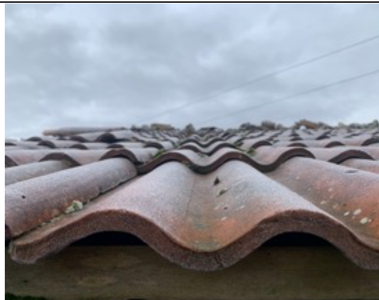
Photo 8: Gaps on the bottom of the Tuscan tiles that lead into the space between the roofing membrane.
