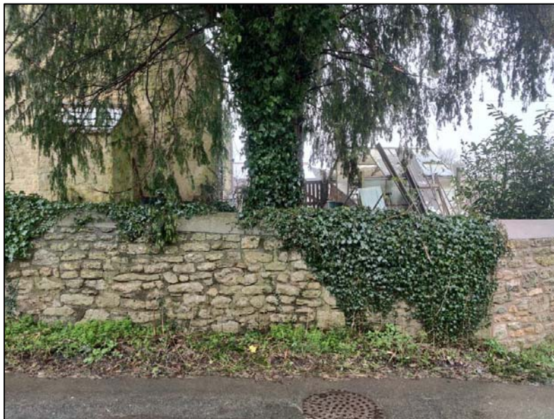
Figure 1: The yew tree is likely to cause cracking of the retaining wall over time.
