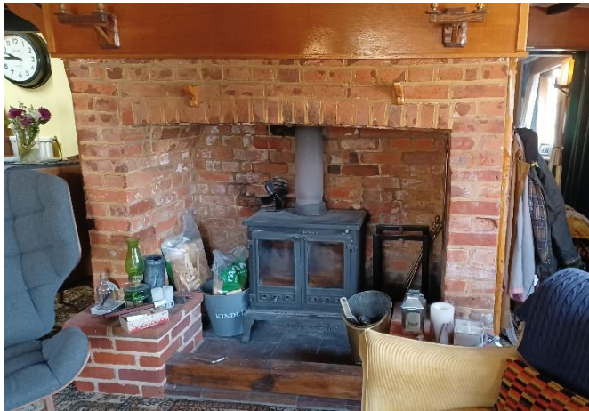
Figure 12 The rebuilt brick fireplace in the room west of the baffle entry
