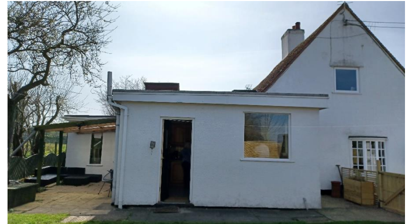
Figure 13 Historic range on the right. Flat-roofed side and rear extensions are twentieth century and do not contribute to significance
