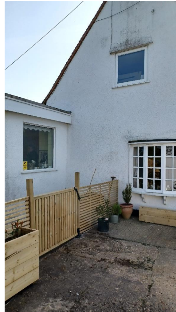
Photo showing junction of existing old and new, bow window to be replaced with new timber sash
