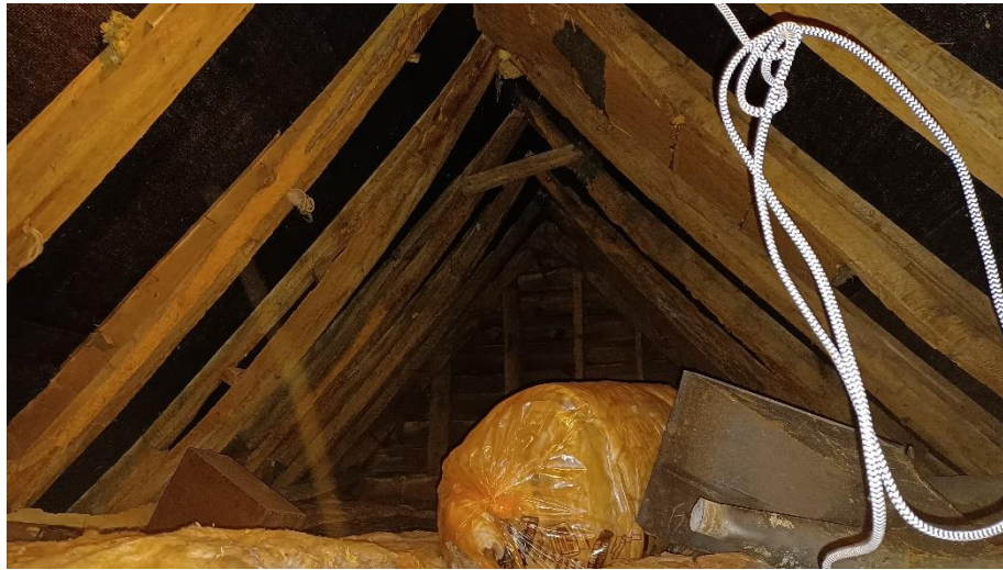
Figure 10 Upper part of historic roof structure, visible in loft space above Inglenook
