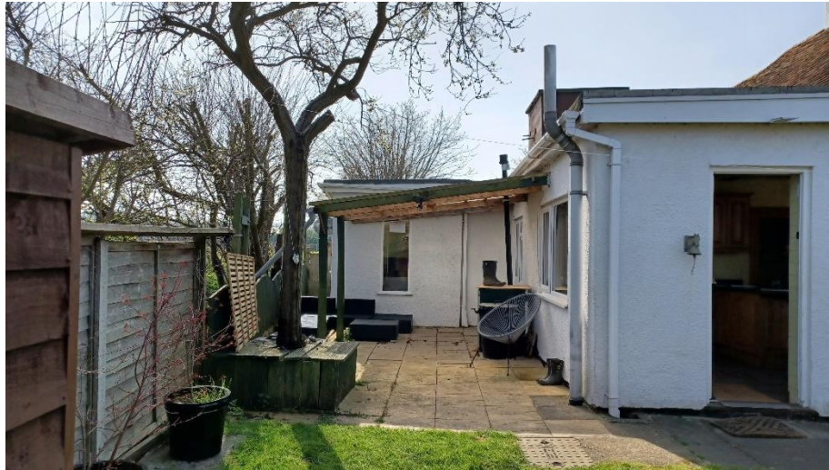
Image looking at rear or east elevation, box on top of roof is water tank, to be removed. New single storey extension to partially infill yard space.
