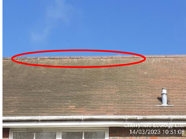
Figure 10: Example of small gaps along ridge where mortar is missing
