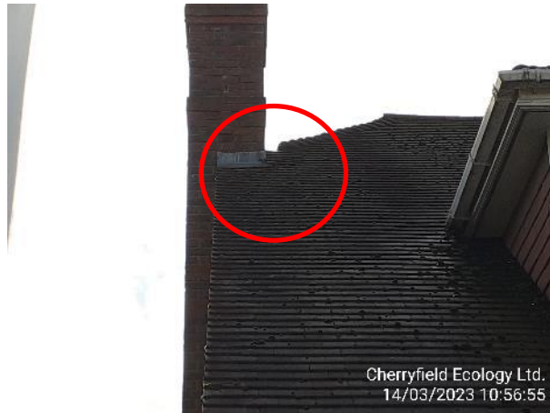
Figure 11: Example of loose tiles around chimney
