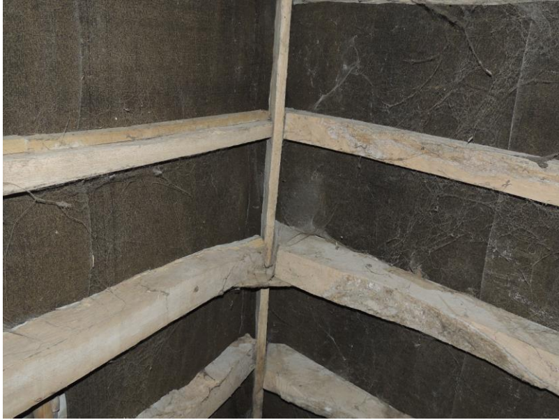
Photo 15: Note cobwebs on rafters
