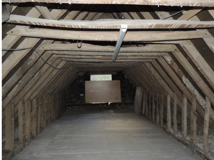
Photo 12: Looking southwards on upper floor. Note cluttered roof structure
