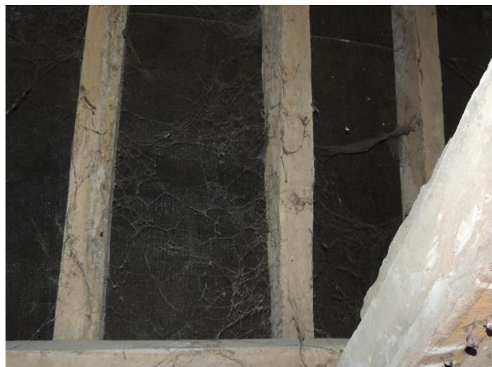
Photo 14: Note cobwebs on rafters
