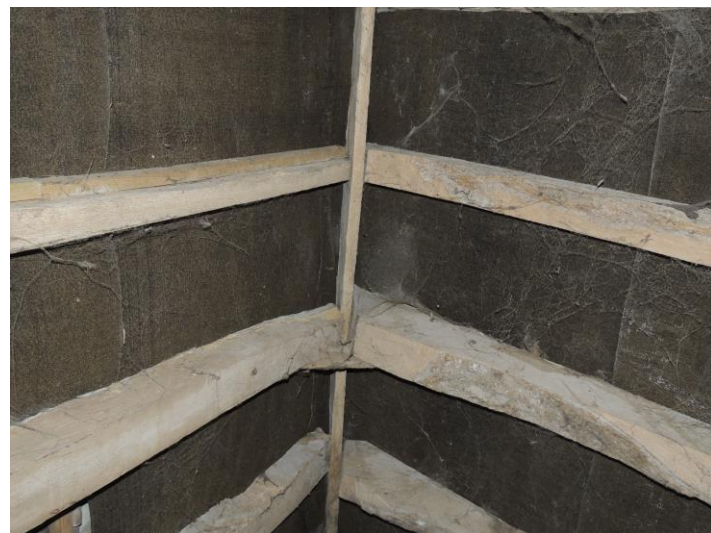
Photo 15: Note cobwebs on rafters
