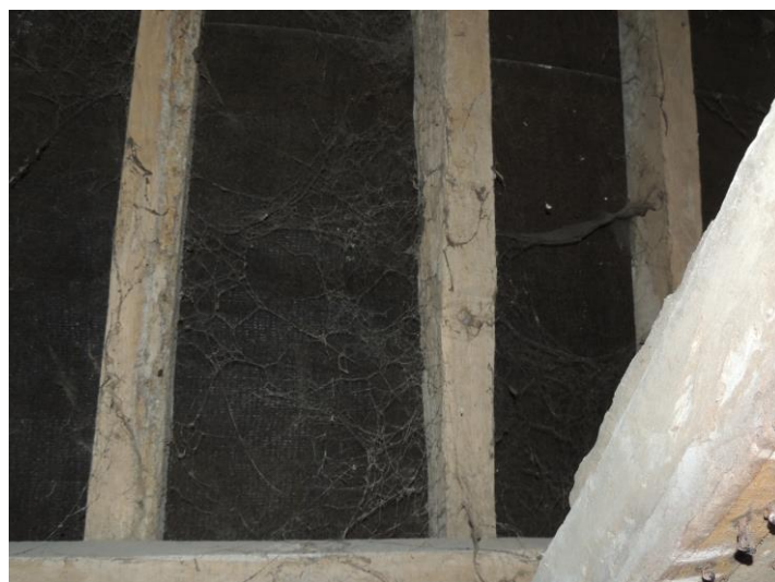
Photo 14: Note cobwebs on rafters
