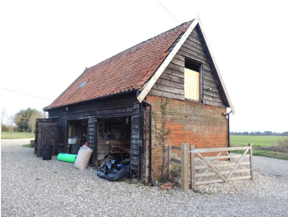
Photo 1: Southern (gabled) and western elevations. The proposal is to convert to residential use. Note extent of gravel
