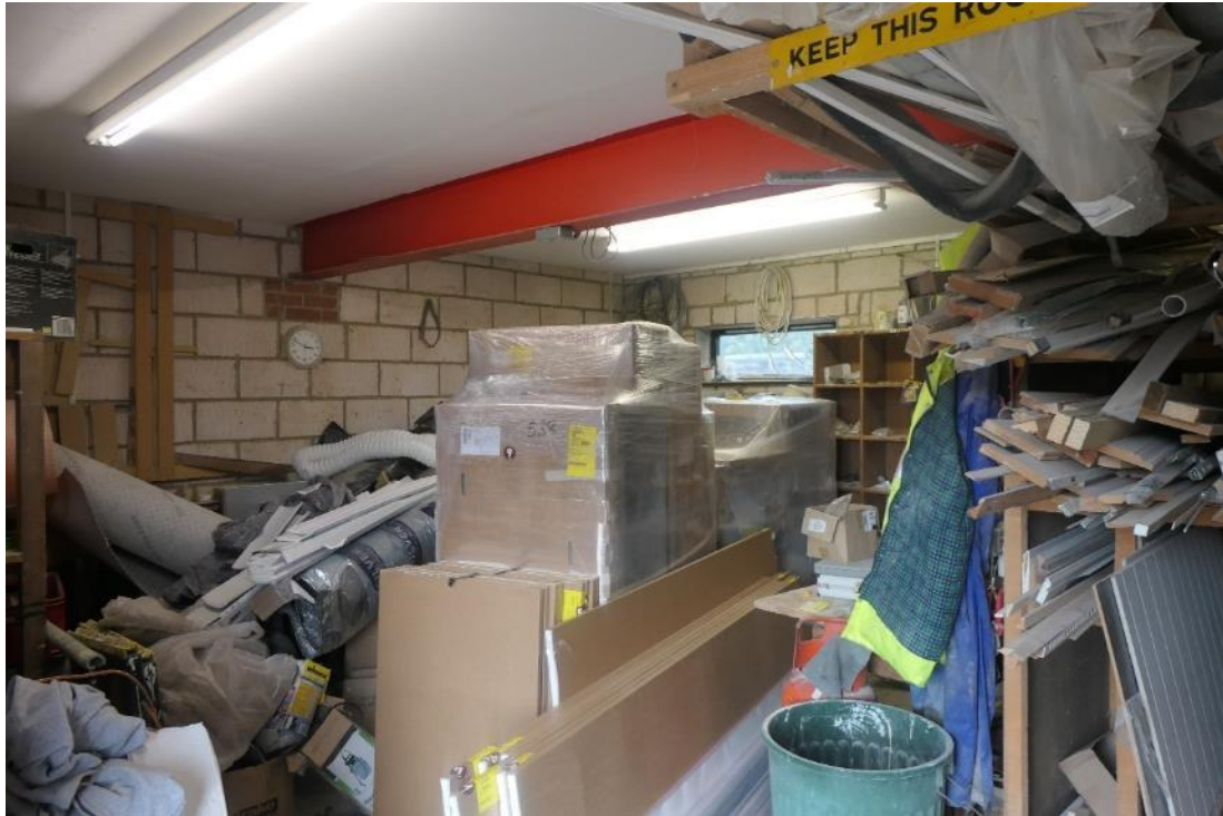
Photo 3 , internal view of the lower level of the building used for storage.
