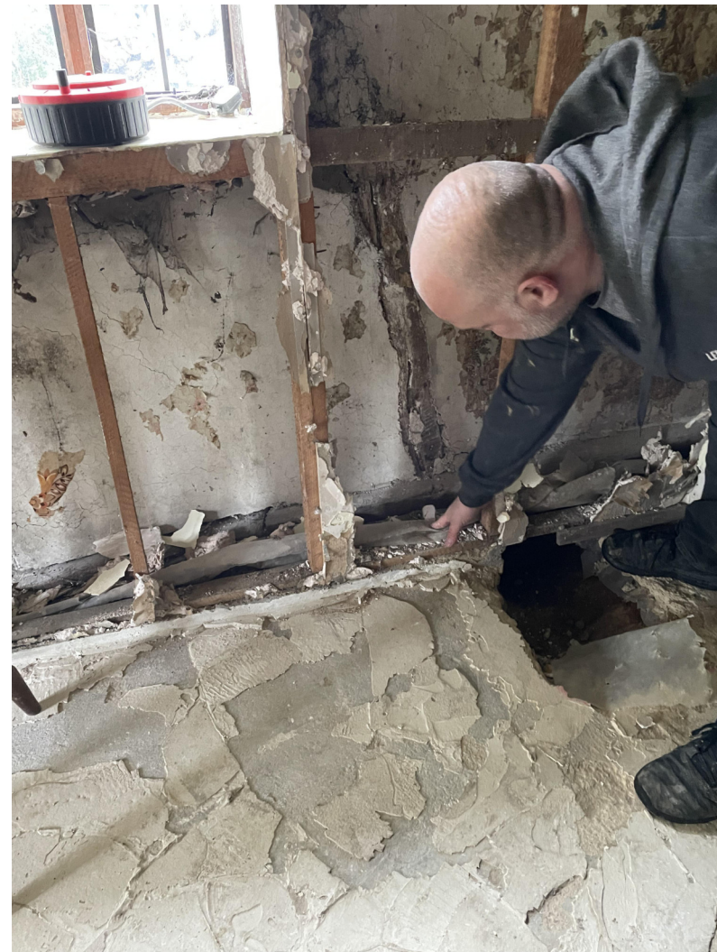
5) Replace missing or damaged soleplate.
