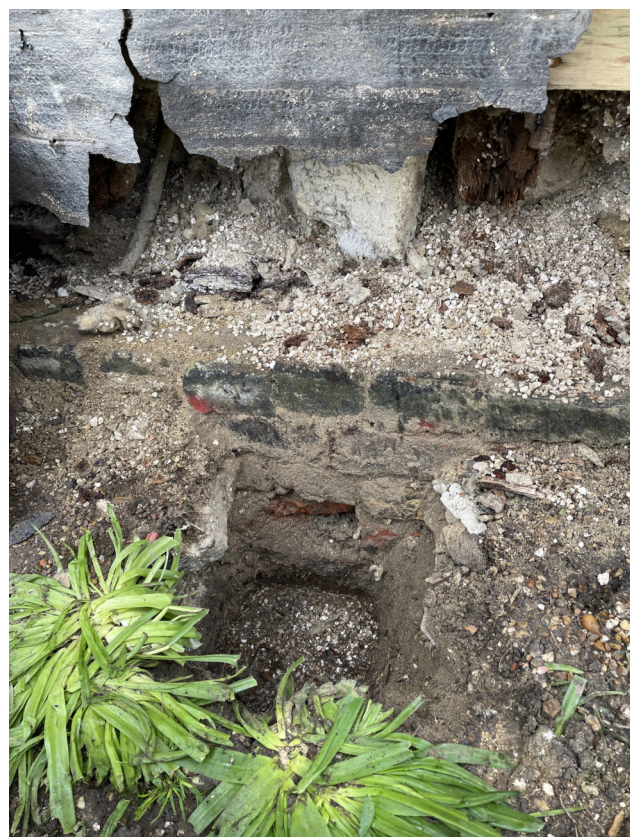
5) Replace missing or damaged soleplate.
