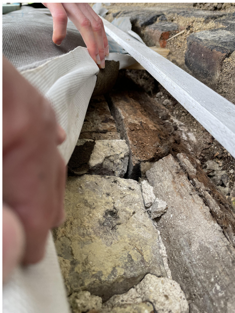
5) Replace missing or damaged soleplate. Note - Replace from present plate joint.
