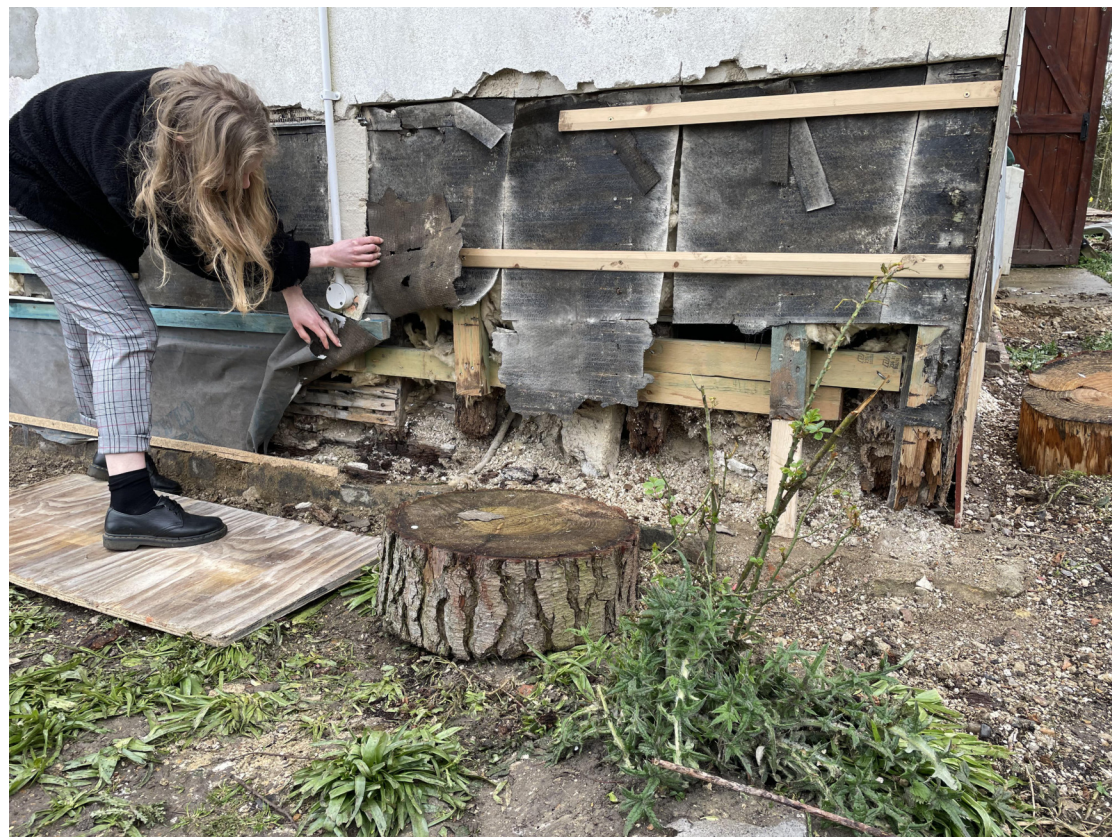
5) Replace missing or damaged soleplate. 6) Re-tenon studs and post and fit to new plate.
