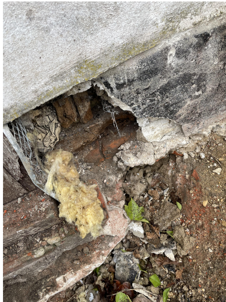
5) Replace missing or damaged soleplate.
