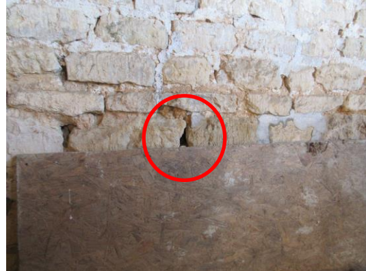
Photograph 2: View of the crevice in the stonework where the bat was found
