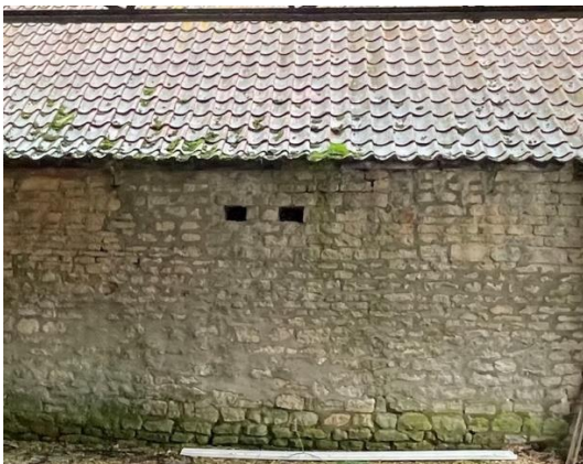
Photograph 53: Holes within western elevation of the stone barn of Building F
