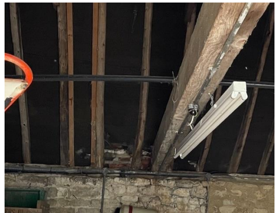
Photograph 54: Rips in the felt lining of the stone barn (Building F)
