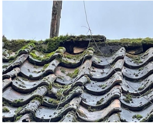
Photograph 13: Lifted ridge tile on Building D
