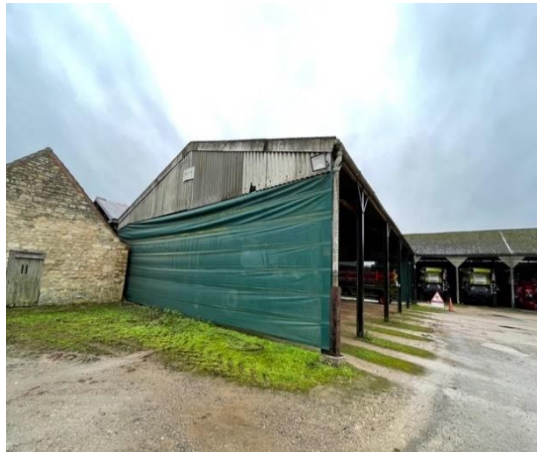
Photograph 21: Fine netting on the eastern elevation
