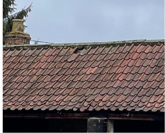
Photograph 50: Missing pantile on Building D
