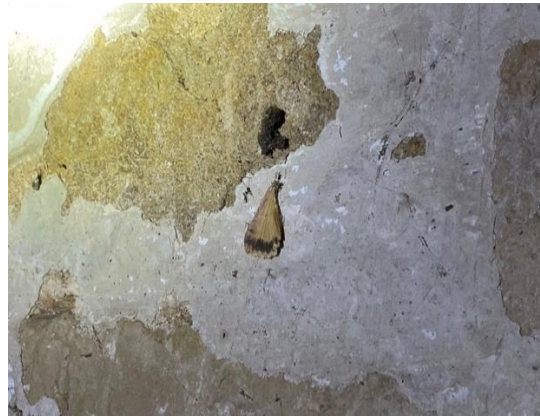
Photograph 58: Moth wing on internal wall of Building G
