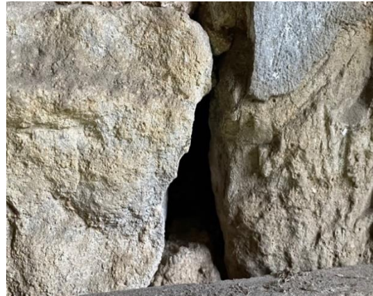
Photograph 46: Further view of gaps in northern elevation of Dutch barn (Building A)
