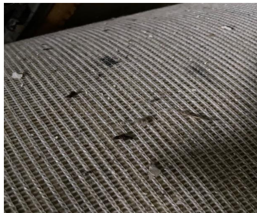
Photograph 59: Bat droppings noted at southern end of Building H
