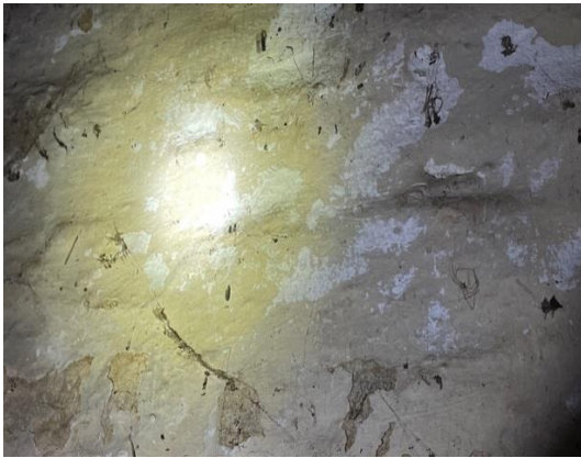
Photograph 57: Bat droppings on the internal wall of Building G
