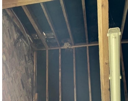
Photograph 61: Swallow nest within Building H
