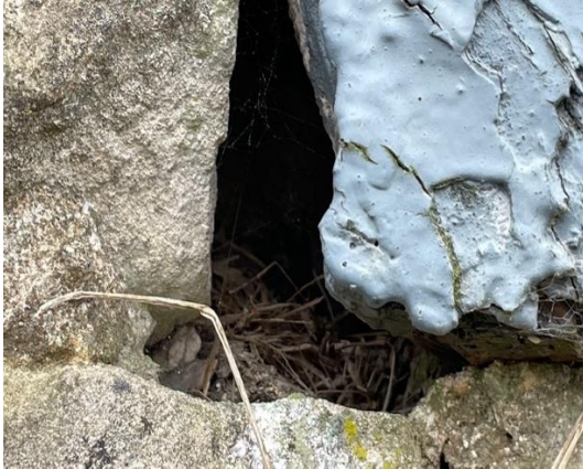
Photograph 60: Nesting material within the stone wall of Building F
