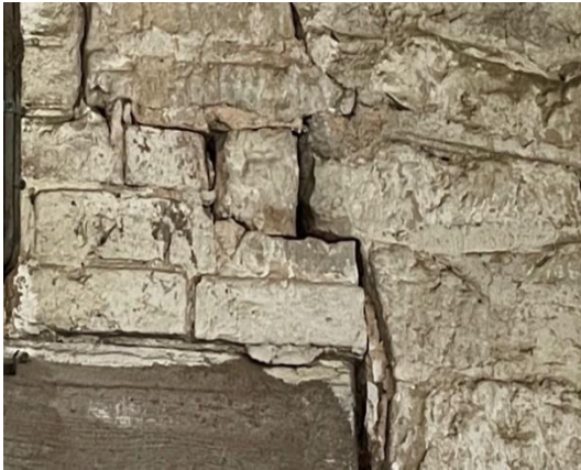
Photograph 45: Gaps within stone wall on the northern elevation of the Dutch barn (Building A)
