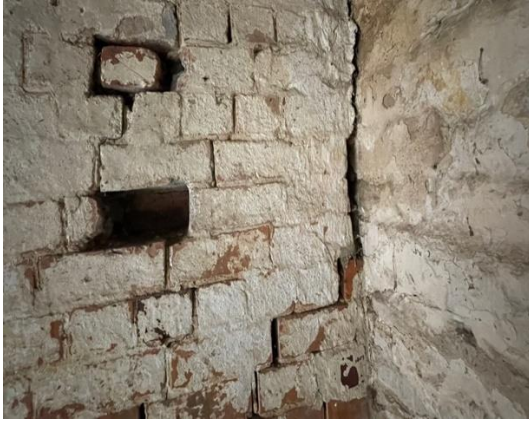
Photograph 55: Holes & niches in brickwork of Building G
