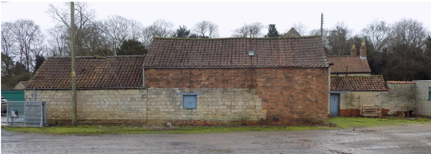
P12 – looking south from the farmyard towards the north elevation of Barn 7, which although shown on the 1799 Enclosure Award Plan has been substantially overbuilt with brick.
