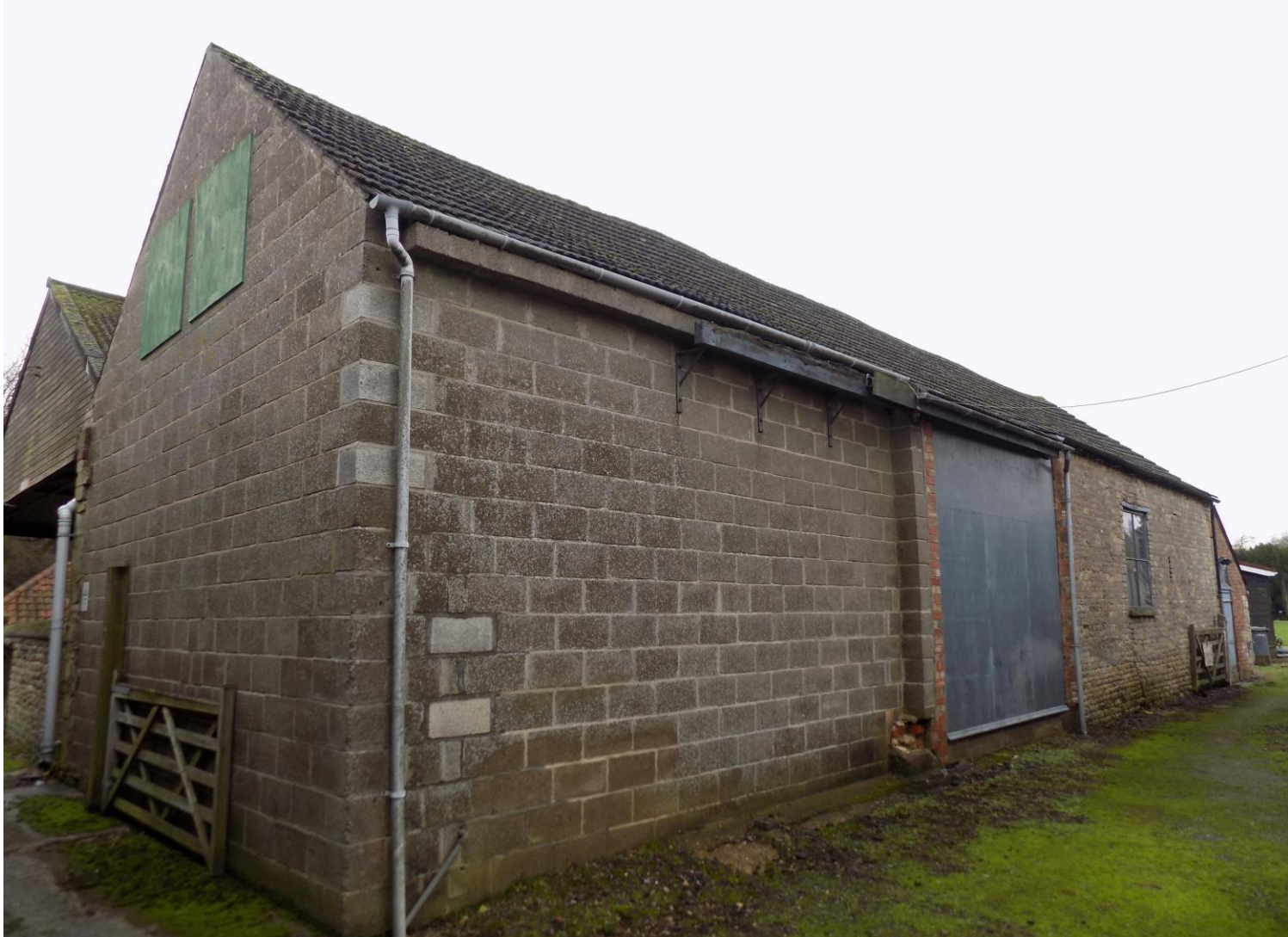
P21- east gable and part of north wall of the early 18 th C threshing barn have been rebuilt with breeze block in the late 20 th C, however, tradition form is maintained
