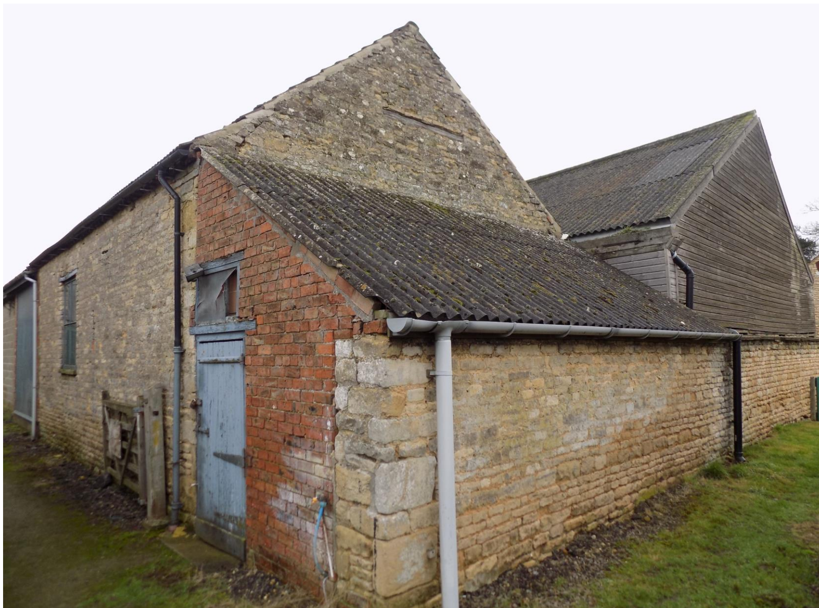
P22 – north west corner of the early 19 th C threshing barn, with a slightly later lean-to with red brick infill.
