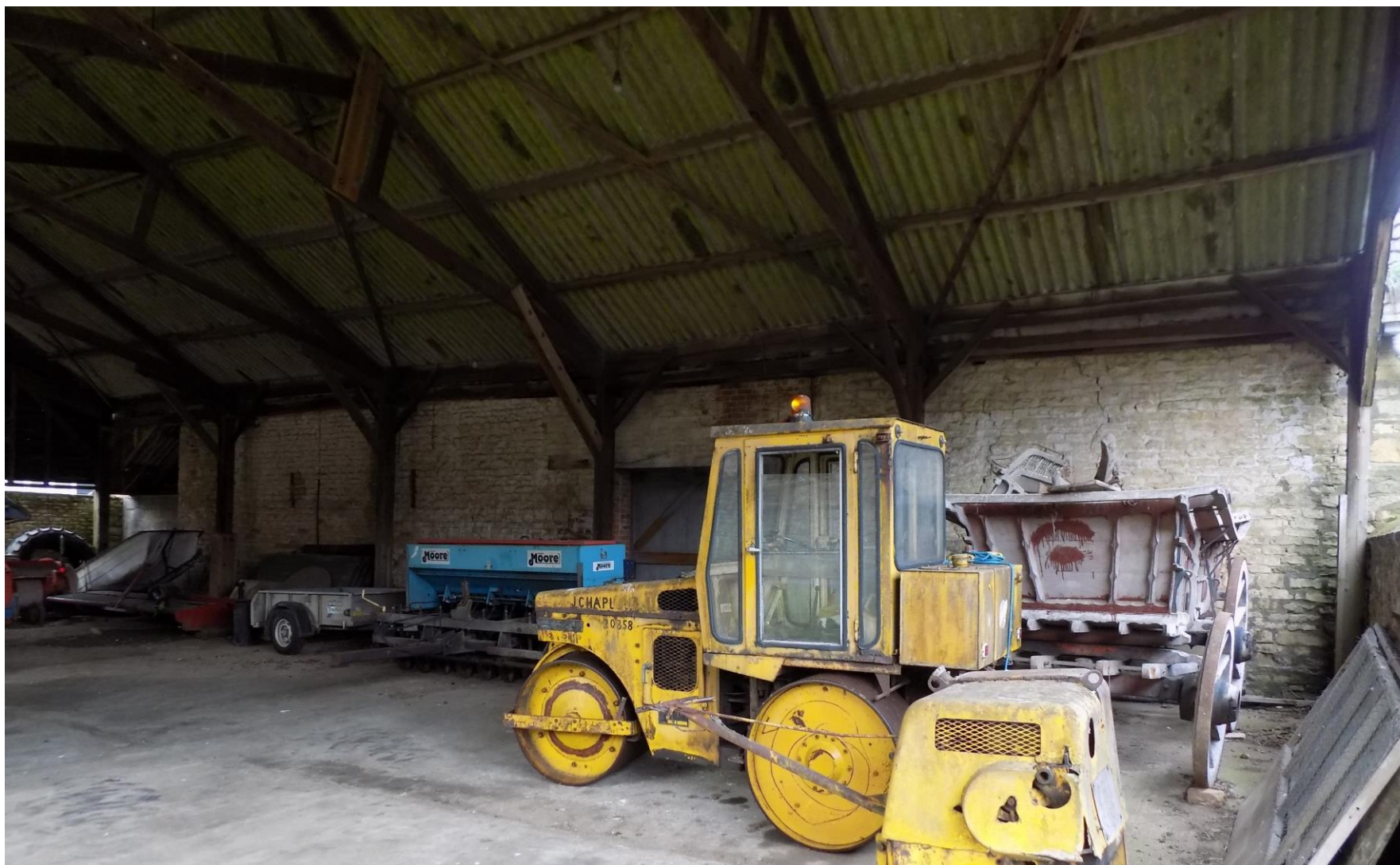
P18 – post 1956 English Brothers timbe frame roof, unusual construction, set directly beside the south elevation of the early 19 th C threshing Barn.
