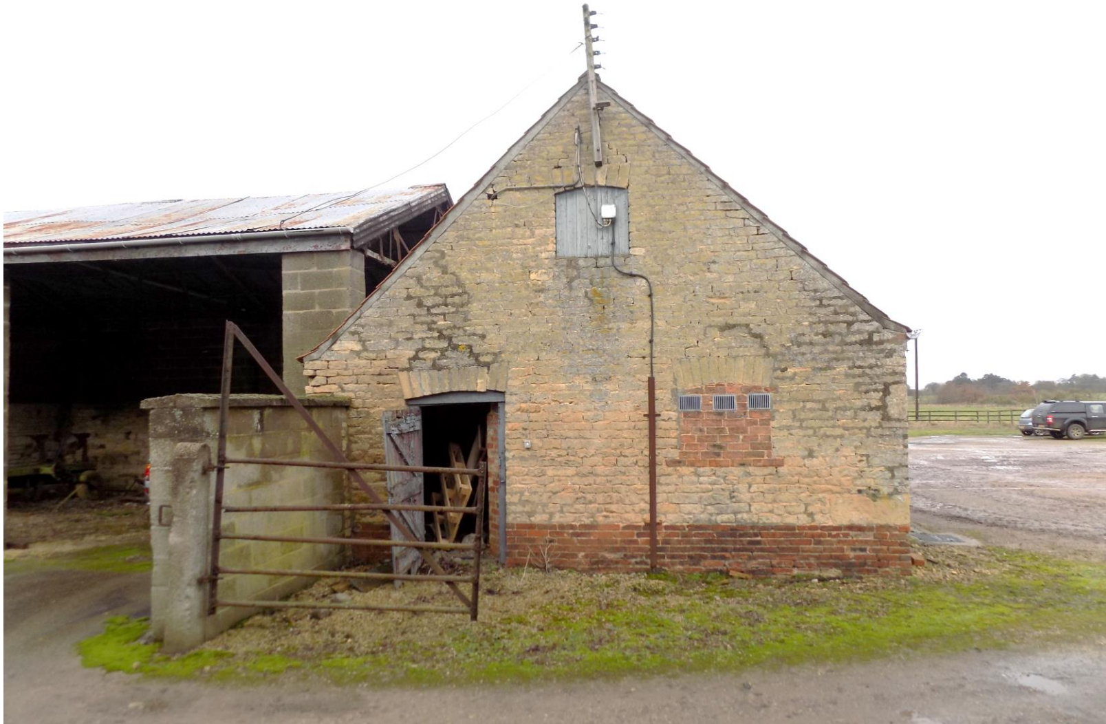
P15 – south gable of Barn 6 (section 1 early 19 th C), brick base, and roughly course limestone above. A modern open fronted shed sits in close proximity.
