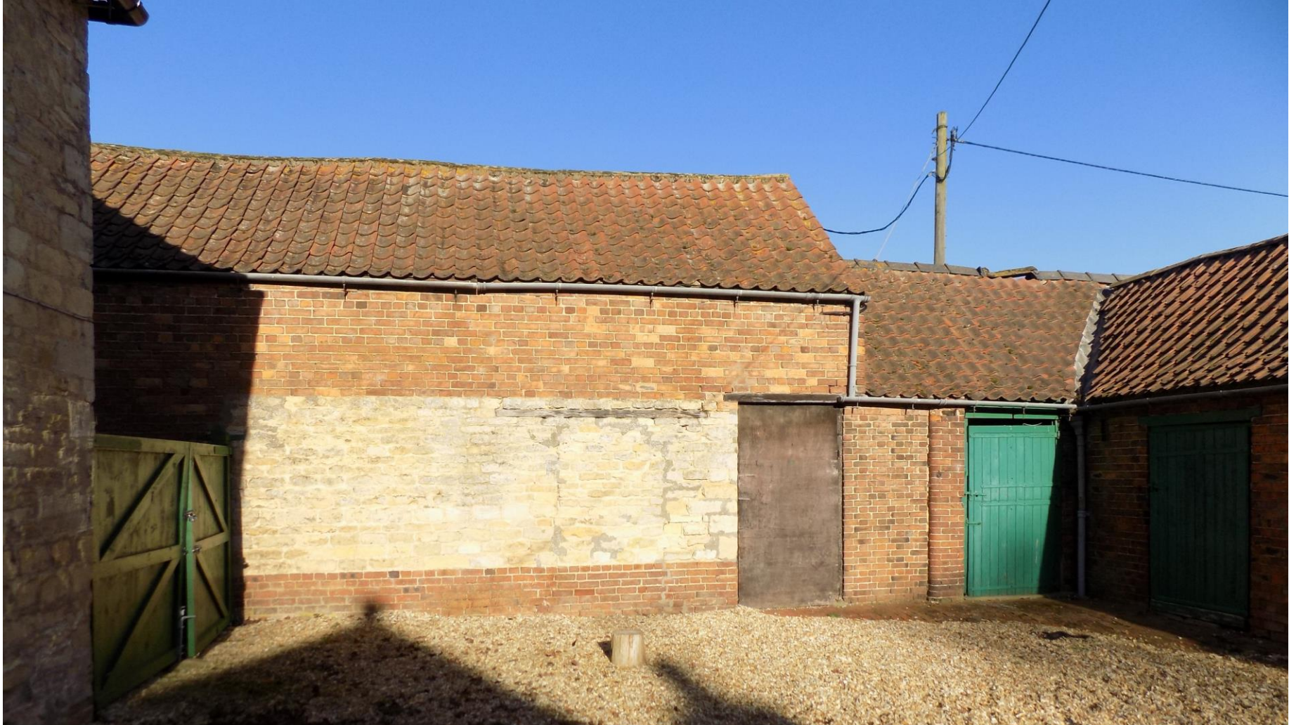
P5 – south elevation of Barn 7, facing courtyard to Village Farmhouse. Note the stone and brick construction.
