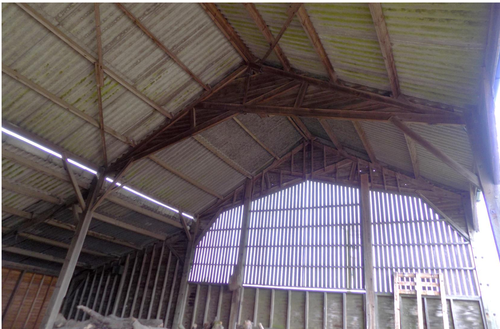
P24 – Interior of Barn 5 has a complex structural timber frame. English Brothers have, since the early 1900's produced structural timber buildings of innovative design. This structure is not without some merit for a building of its type.
