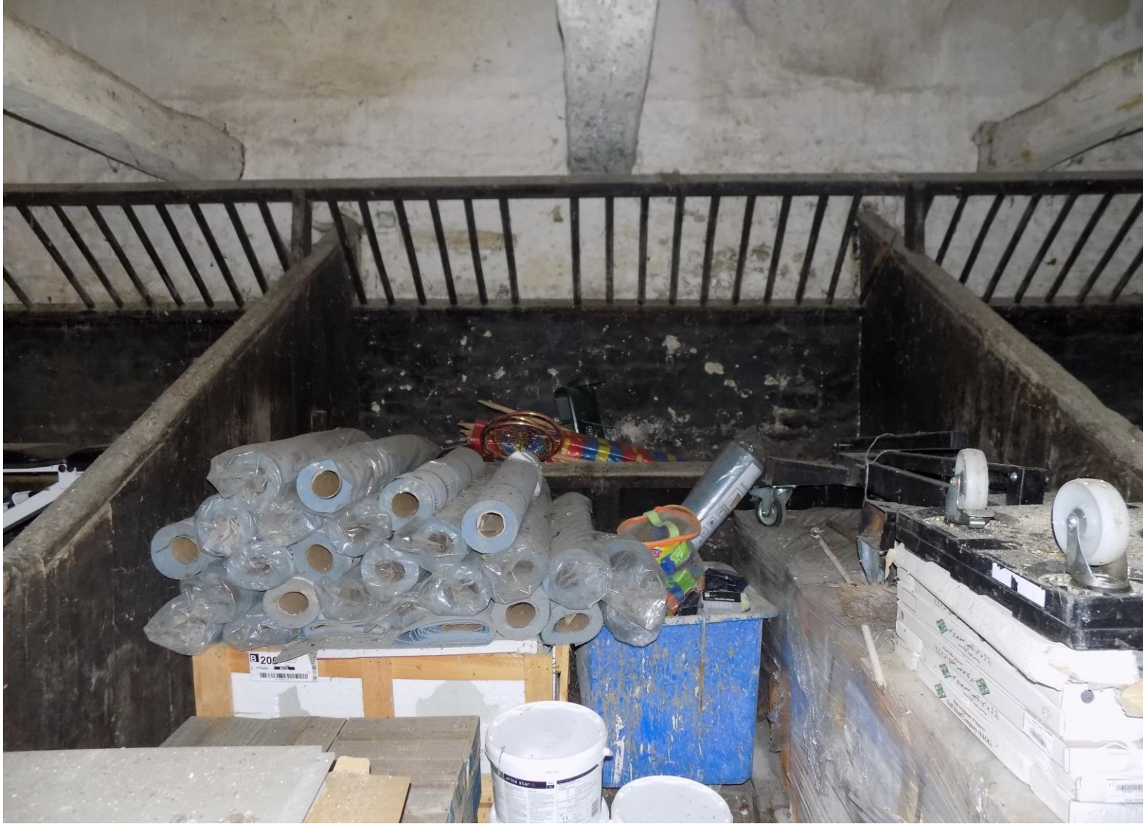
P37 – timber stalls, feed racks, and black painted walls. Detritus obscures brick feeding trough behind.
