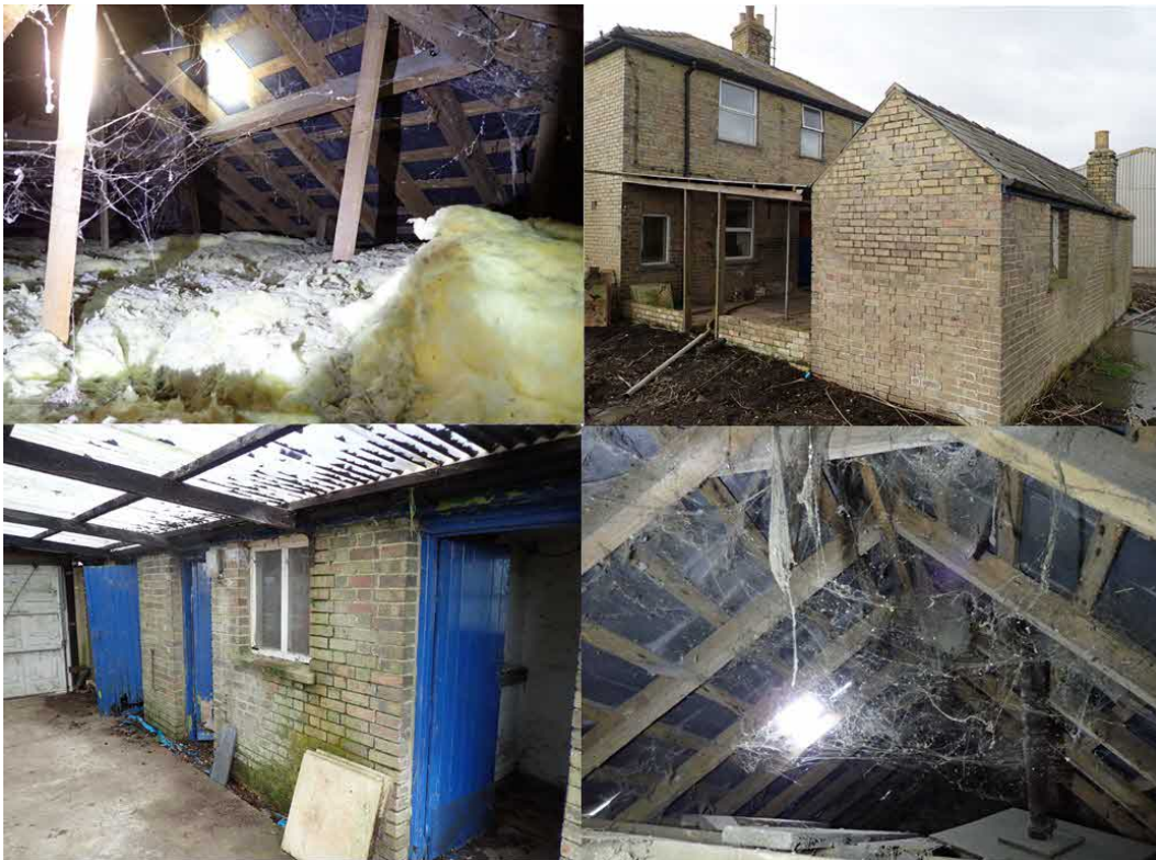
Photograph Group 2: (top left) Dwelling loft; (top right) Out-building from the north-east; (lower left) The outbuilding from dwelling; (lower right) Roof space of the outbuilding.
