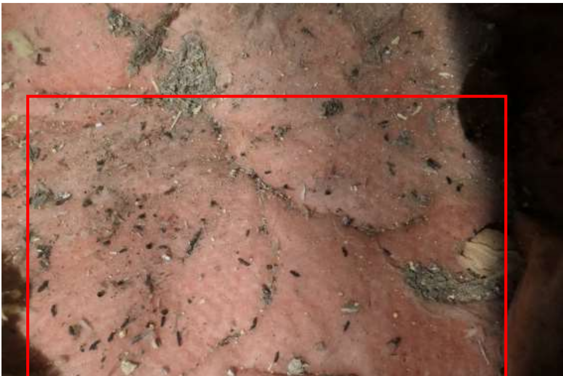
Photo 8 , cluster of bat droppings present within loft space and highlighted in red.
