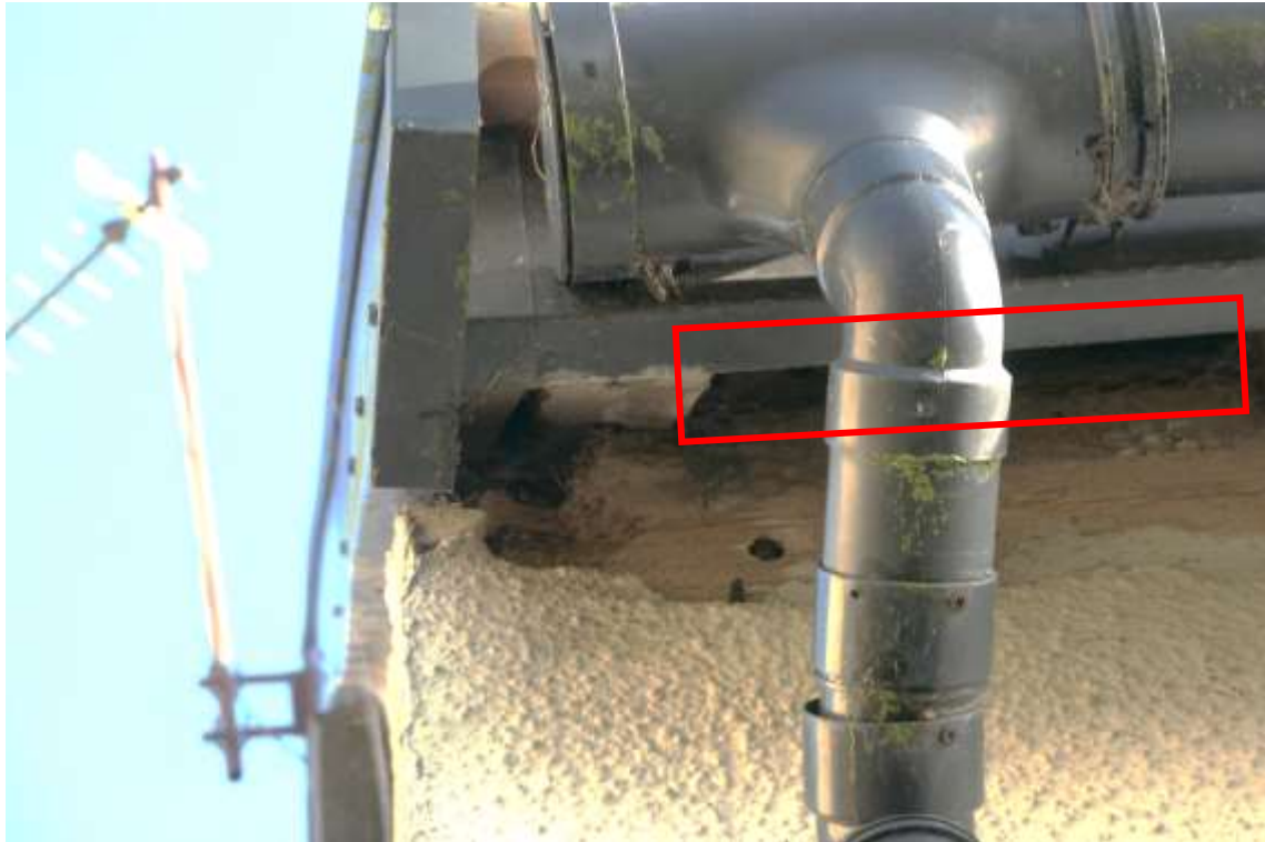
Photo 9 , gaps at eaves highlighted in red on the west aspect of building one.
