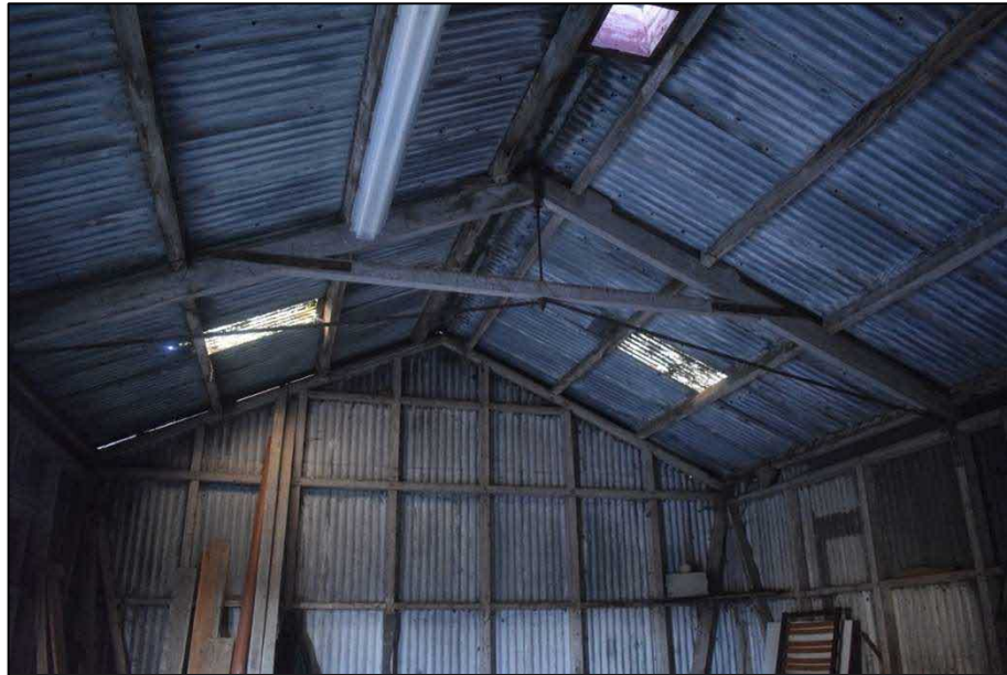
Fig. 10 Metal reinforced roof truss and details of wall frame in Outbuilding 3 Photo CPAT 5036-047
