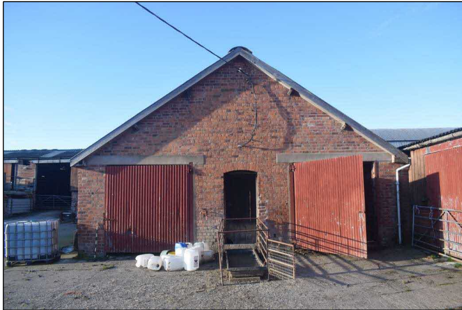
Fig. 11 Eastern gable end of Outbuilding 4, with modern doorway insertions and later brickwork Photo CPAT 5036-051
