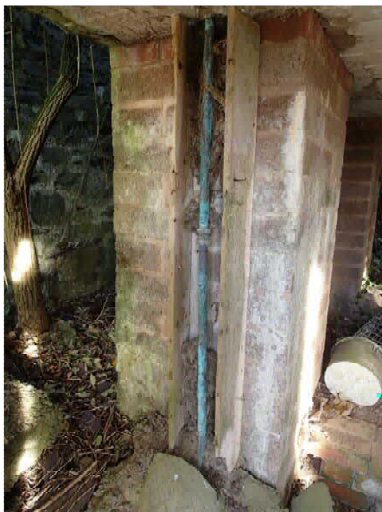
Copper pipe (possibly pumped supply) covered in green patina, which will eventually corrode the pipe.
