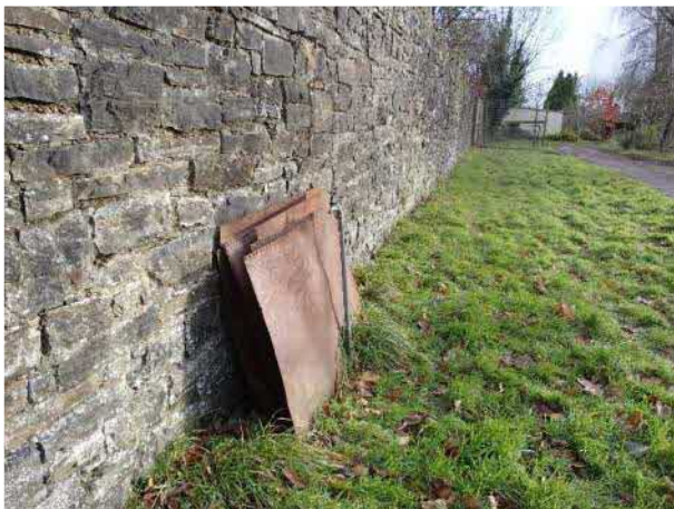
External water stand-pipe against outside of site wall. The tap was not working.
