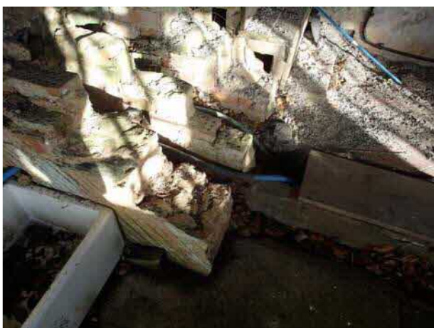
Exposed blue water pipe in lean-to
