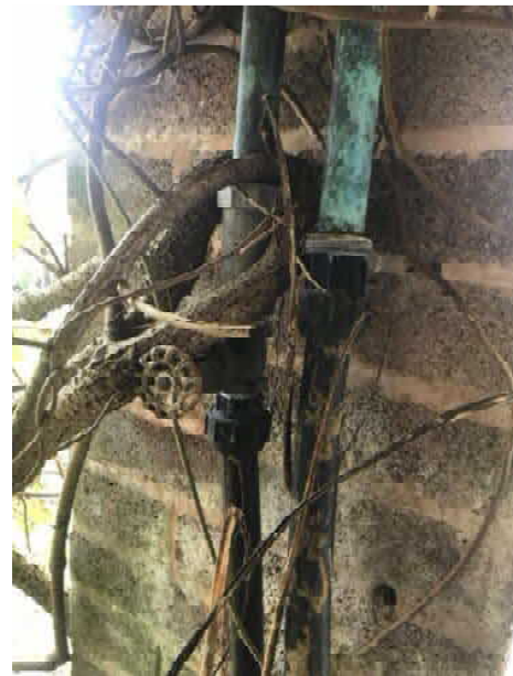
Immovable valve and pipes under cistern tangled with thick tree branches.
