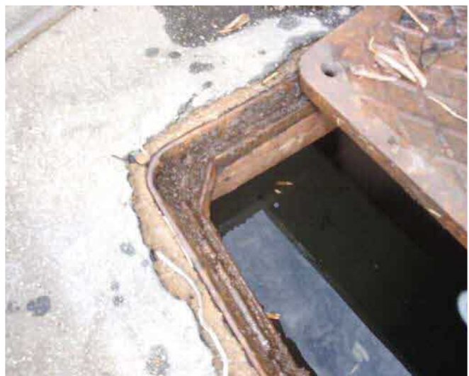
Cistern access cover. Cover will not fully protect against mud, insects and rain water entry. There is no seal or locking nuts.
