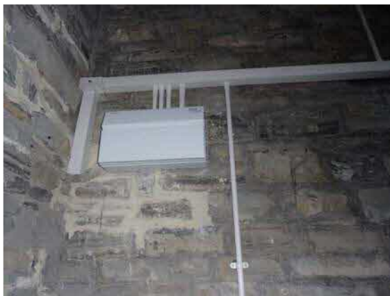
Bothy single phase power and lighting electrical consumer unit
