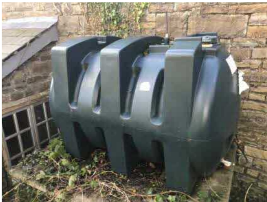
Oil storage tank behind bothy
