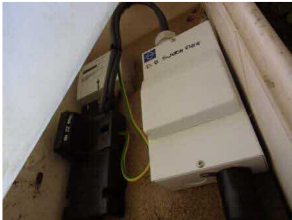
Existing incoming power supply and meter located under dilapidated lean-to. The supply has a 415v fuse cut-out indicating that the incoming supply is 3 phase.
