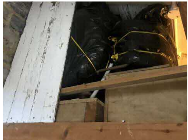
Insulated domestic water tanks serving bothy
