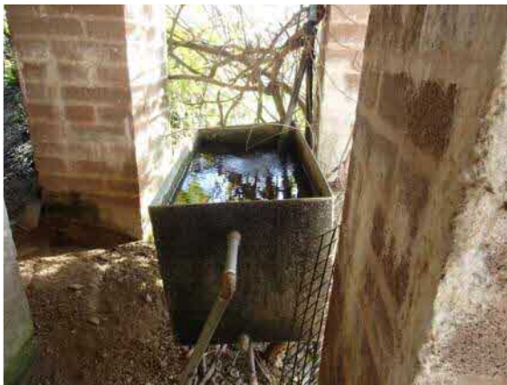
Unknown open vessel below cistern. Possibly an overflow tank of some description for cistern above.
