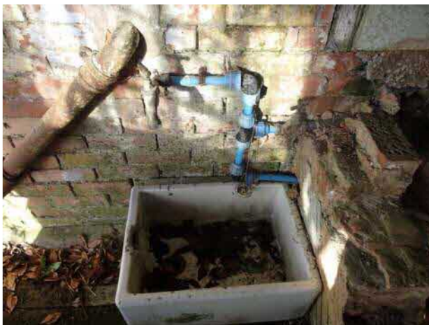
Earthenware sink with MDPE water supply in bothy
