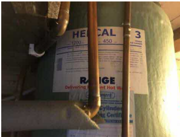
Direct heated hot water cylinder serving bothy
