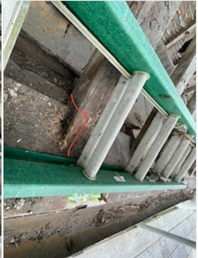
Figure 12: Showing area of decay.
