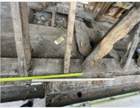
Figure 3: Showing defective section of wall plate.
