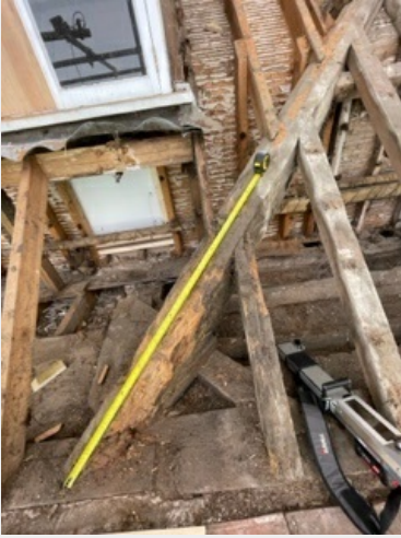
Figure 1: Showing defective hip rafter.
