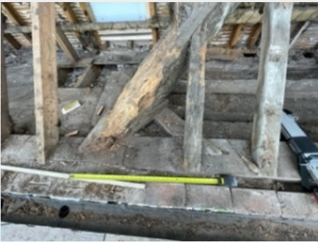
Figure 2: Showing defective section of wall plate.
