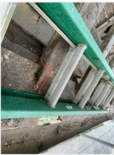
Figure 12: Showing area of decay.
