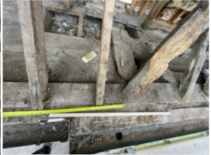
Figure 3: Showing defective section of wall plate.
