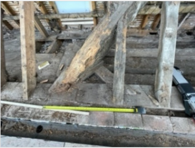
Figure 2: Showing defective section of wall plate.
