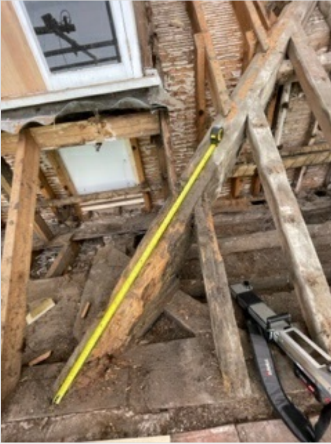
Figure 1: Showing defective hip rafter.
