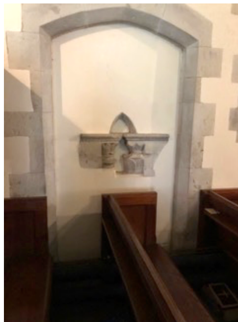
5 Blocked-in doorway in the North Aisle. Fragments of Norman masonry have been embedded in the wall. These will be re-installed beneath an adjacent window.
