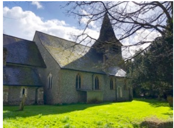
4 North Aisle viewed from the east. The enclosure against the aisle is above the underground oil tank.
