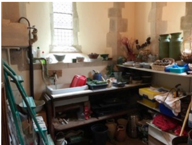
4 Interior of partitioned area. This will once again be part of the North Aisle. Its contents will be accommodated in the extension.
