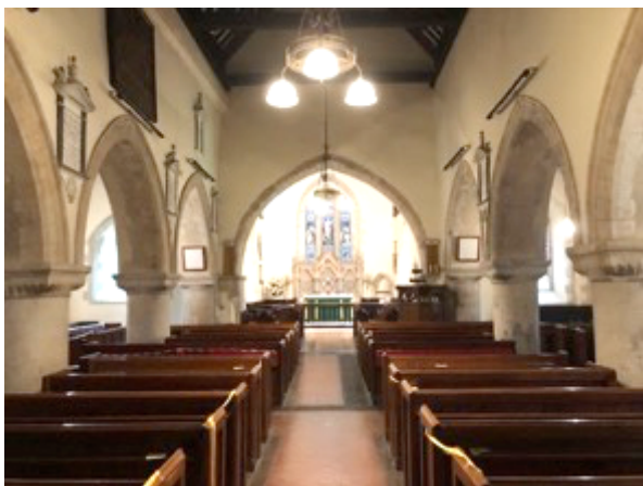
1 Interior looking east. The modest scale of the arcade offsets the loftiness of the roof. The Nave suffers from a lack of natural light.
