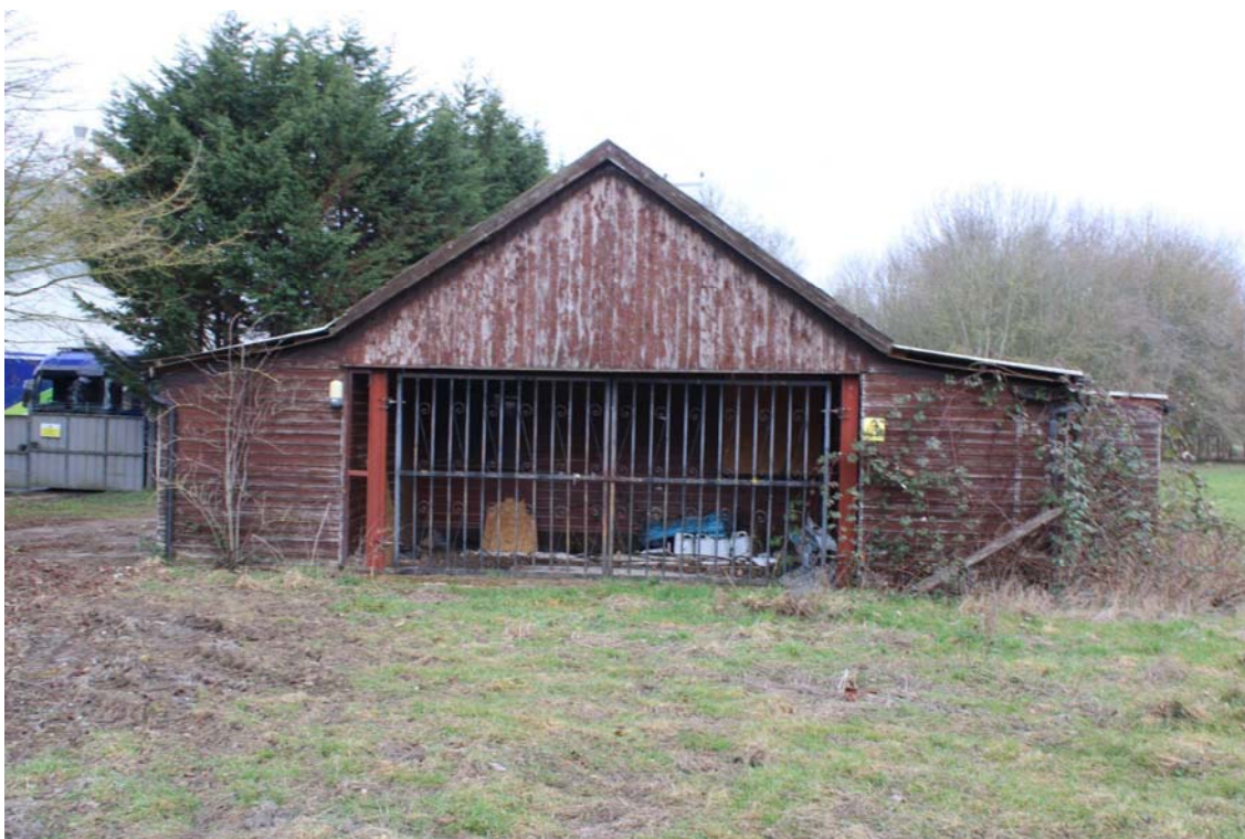
Plate 9: Detail of the southern elevation of the disused sports pavilion, with concrete foundation pad extending west as a surface
