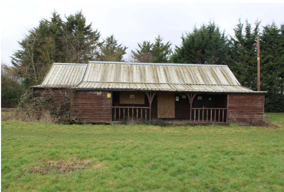
Plate 10: Detail of the east-facing elevation of the pavilion, with no extension of the concrete pad beyond the south, east and north elevations
