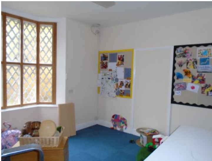
Lower floor Room 17 showing bay window facing west to receive replacement secondary glazing
