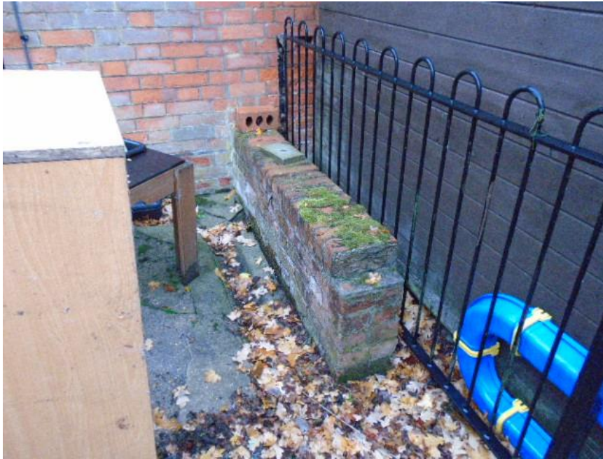
Section of low wall to be removed, adjacent to shed and fencing to be removed
