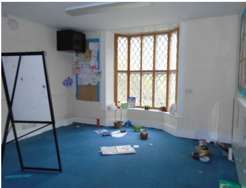
Lower floor Room 18 showing bay window facing west to receive replacement secondary glazing
