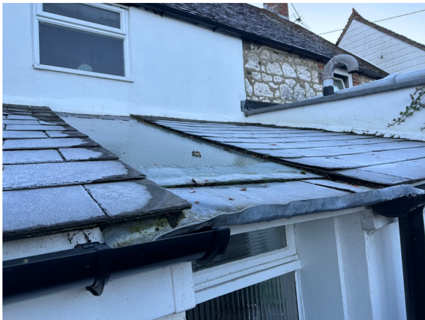
Existing roofs are too shallow, leak and not insulated.
