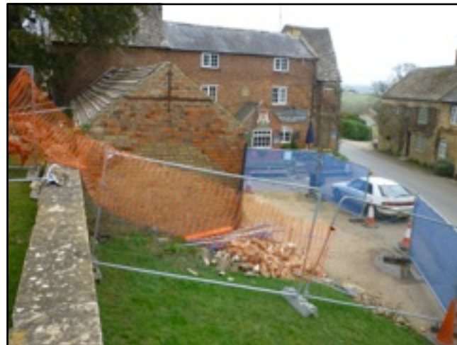
Top: View of site prior to collapse Middle: View of site following collapse Bottom: View of site from Churchyard
