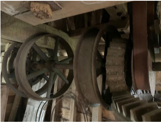
The Ancillary drives over the Crown wheel will be cleaned, repaired as necessary and painted in dark grey
