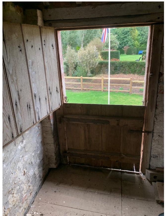
The loading doorway on the stone floor will be retained. The stable door arrangement will be refurbished and pinned back to the wall and used as an internal working shutter. The opening will be infilled with fixed double glazing to comprise 6mm toughened and laminated glass, to conform to current building regulations standard.
