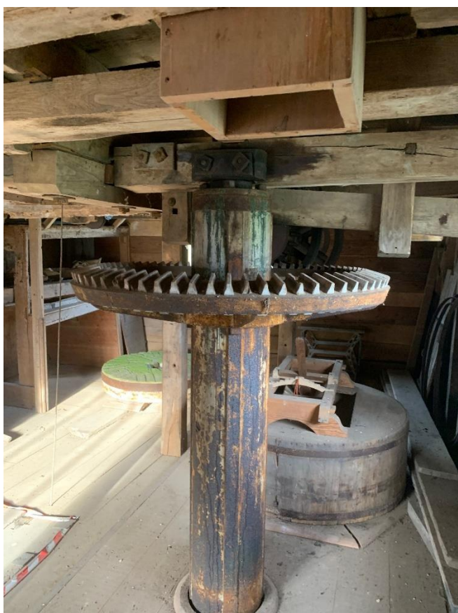
The Stone Floor (First floor) – The Hopper, Crown wheel and Mainshaft will be retained as part of the refurbishment plan. These elements will be cleaned, repaired as necessary and painted in dark grey. Note the sack flaps, bottom left of this photo to be retained.
