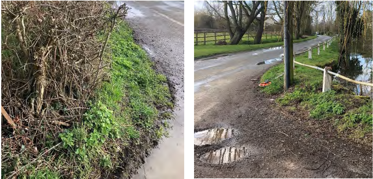
Image 1 – Indications of vehicle overrun at both edges of the site access.
