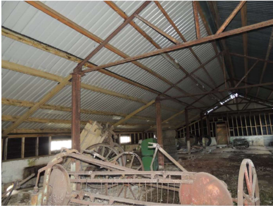
The interior of building 5 had no features that might be occupied by bats
