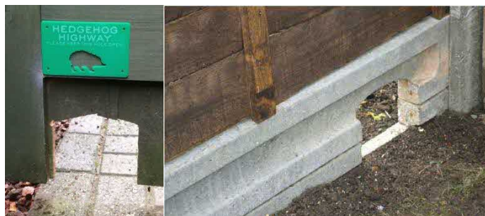
Insert 3: Showing wildlife access gap within fencing
